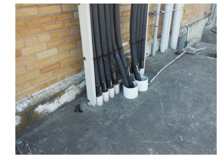
CABLES & CONDUITS AT SOUTH SUBSTATION
