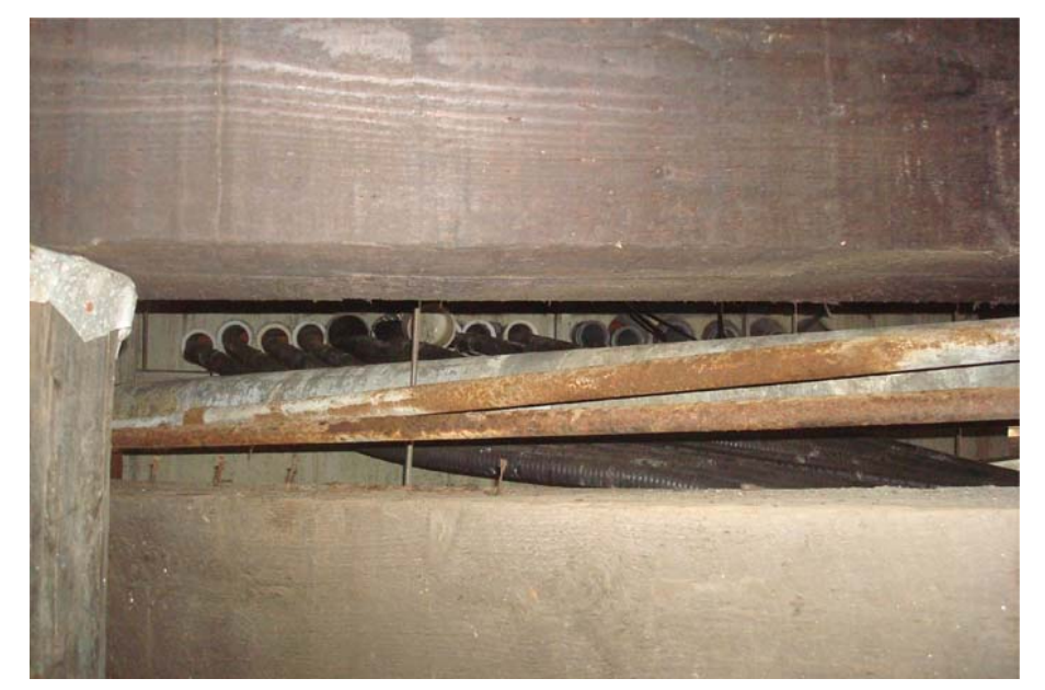
CABLES TRANSITIONING FROM SLEEVES/CONDUITS TO TRAY UNDER JETTY
