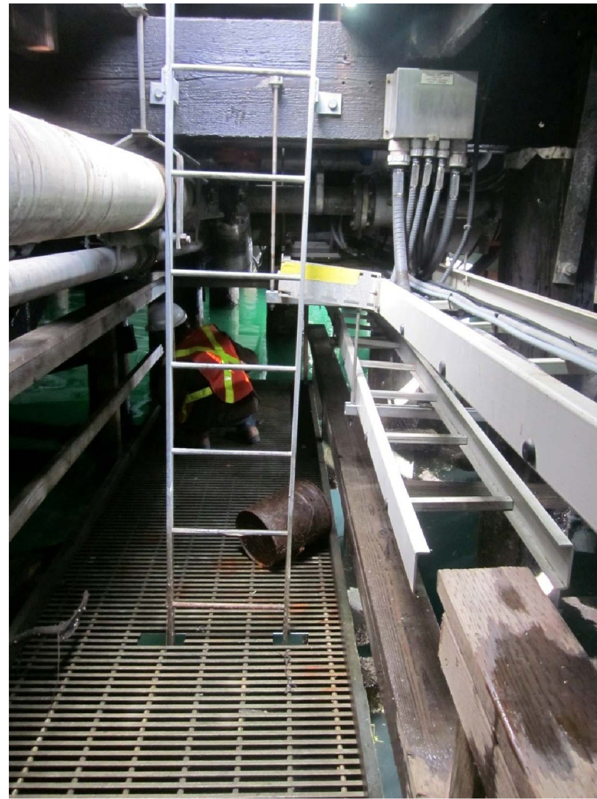
PHOTO C16-01 SOUTH JETTY CATWALK LADDER ACCESS AND CABLING LAYOUT
