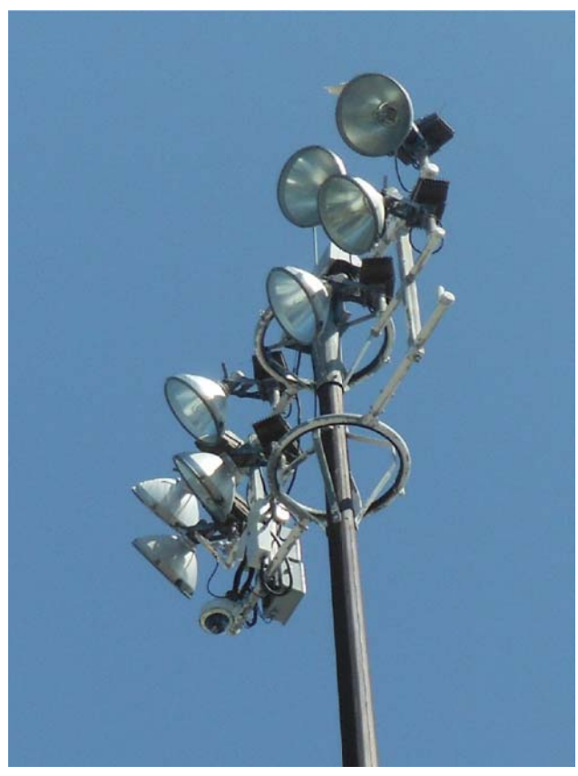
HIGH MAST LIGHT (HML) ASSEMBLY & CCTV CAMERA SYSTEM
