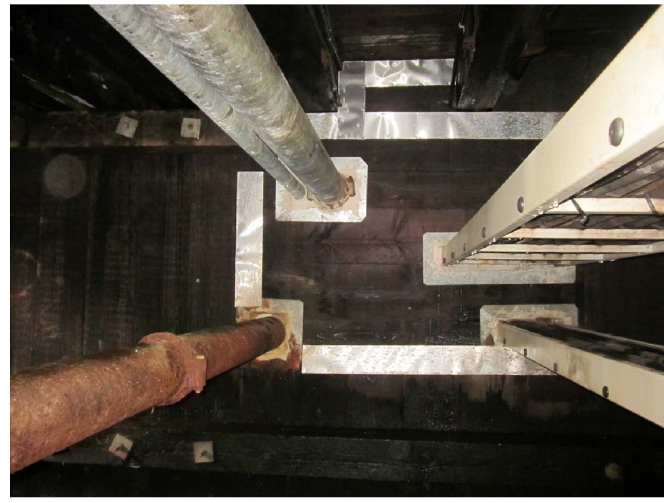
PHOTO C16-04 UNDER-PIER MECHANICAL AND ELECTRICAL SERVICES AT TIMBER FIRE STOP WALL
