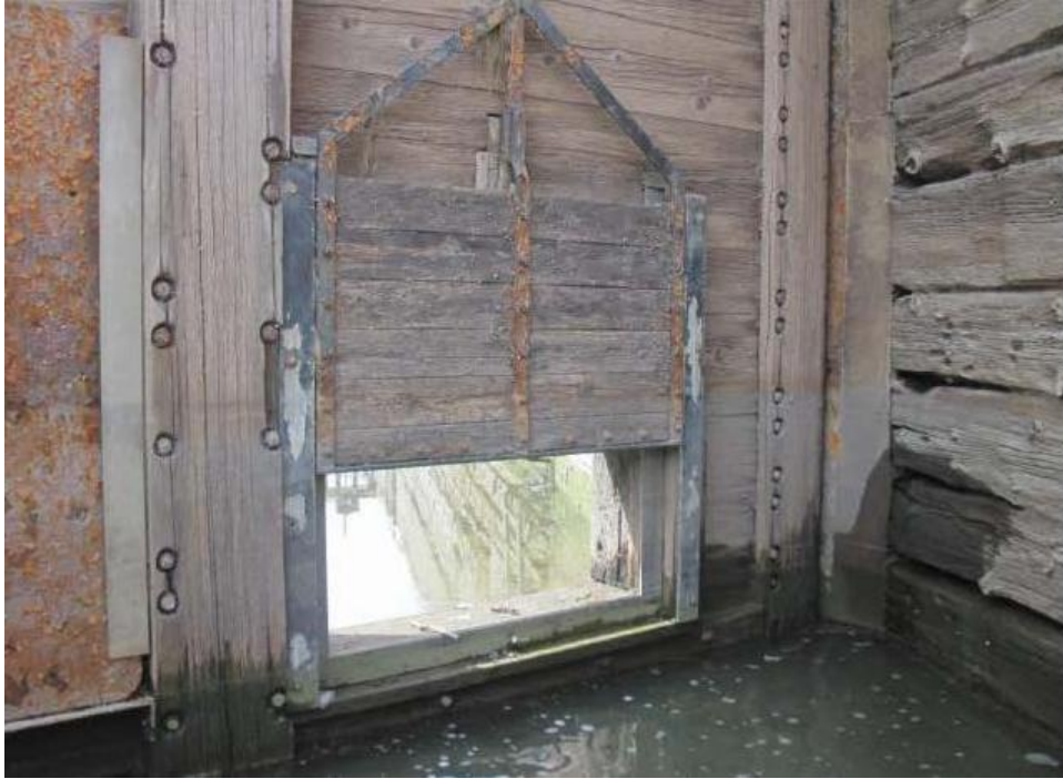
Photograph 2 - Right Bank Slide Gate
