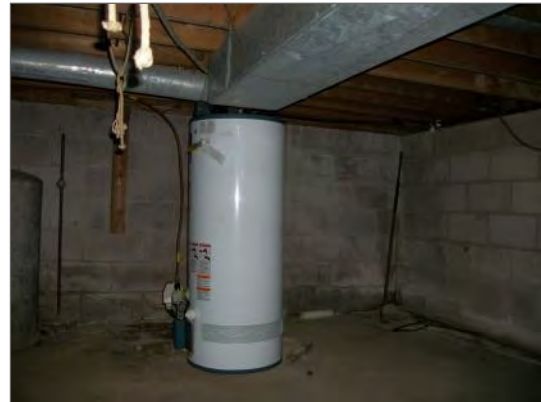
Domestic hot water heater is insulated with fibreglass, Crawlspace
