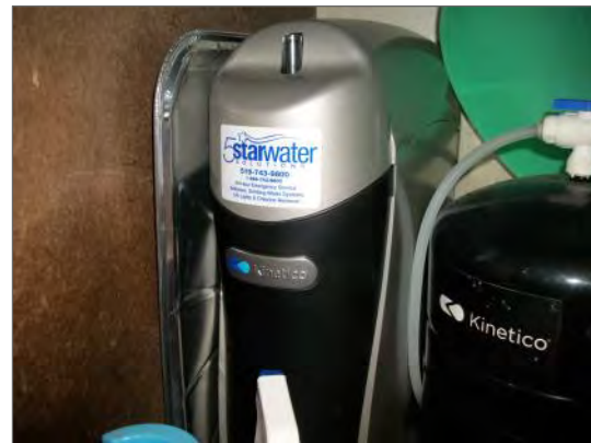
Water softener and associated chemicals, Ground Level Kitchen
