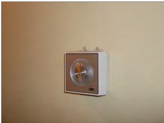
Mercury-containing thermostat, Upper Level Corridor
