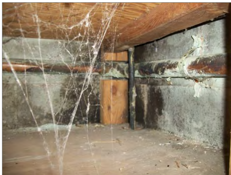
Suspect mould growth on concrete block wall, Closet within Basement Laundry Room
