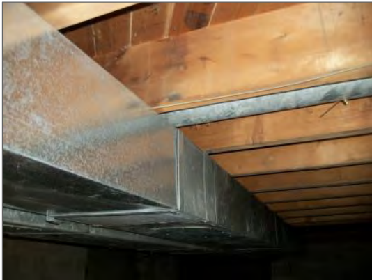
Uninsulated ductwork, Crawlspace
