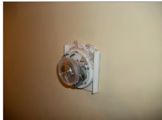
Mercury-containing thermostat ampoule, Upper Level Corridor
