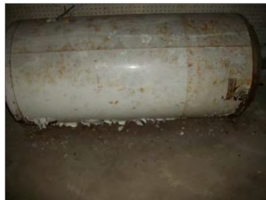
Flaking lead-containing off-white paint on redundant water heater, Crawlspace
