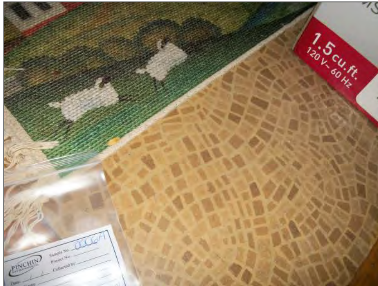
Non-asbestos vinyl sheet flooring, brown mosaic pattern (samples 0006a-c), Main Level Living Room
