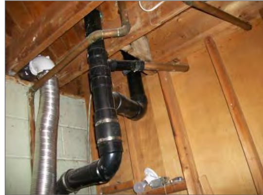
Uninsulated pipes, Basement Laundry Room
