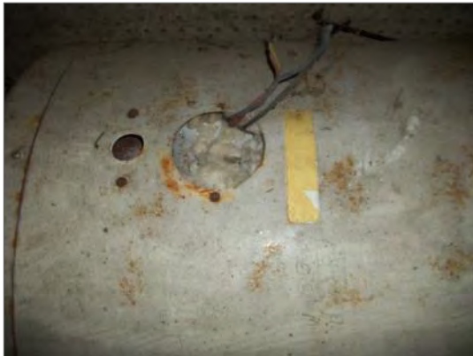
Redundant domestic hot water heater is insulated with fibreglass, Crawlspace
