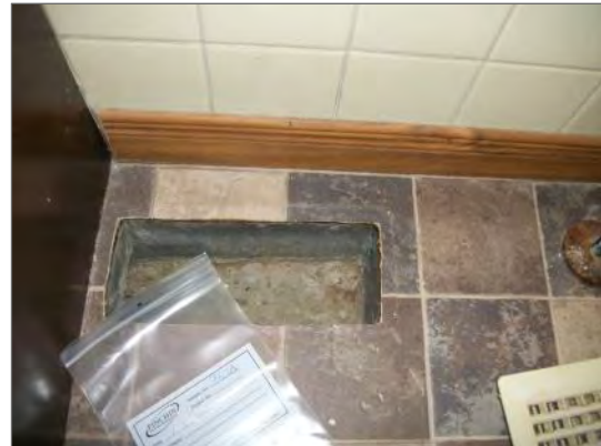
Vinyl sheet flooring with asbestos-containing vinyl backing, brown tile pattern, Upper Level Washroom
