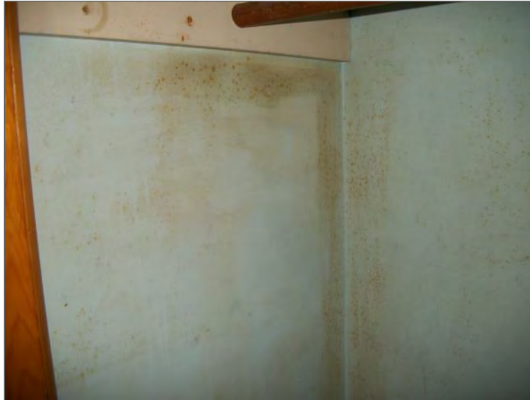
Suspect mould growth on plaster walls, Closet within Upper Level Bedroom
