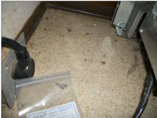
Asbestos-containing vinyl sheet flooring, beige square pattern, Kitchen
