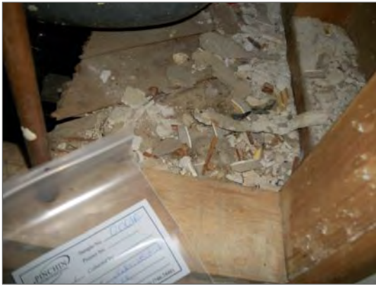
Non-asbestos plaster debris with asbestos-containing yellow adhesive (sample 0001e, Phase A), at bathtub as accessed from the Closet in the Upper Level Office
