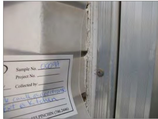
Asbestos-containing white caulking at door frame, Exterior at Kitchen Entrance
