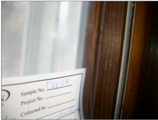
Asbestos-containing brown caulking within wood window frame, Upper Level Office
