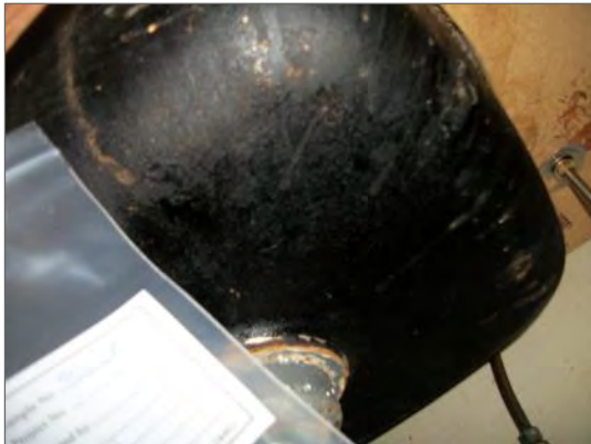
Asbestos-containing black undercoating on sink, Kitchen
