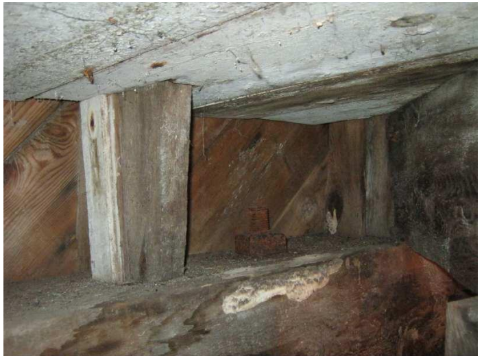
#16 - Anchor Bolt - Missing Plate Washer
