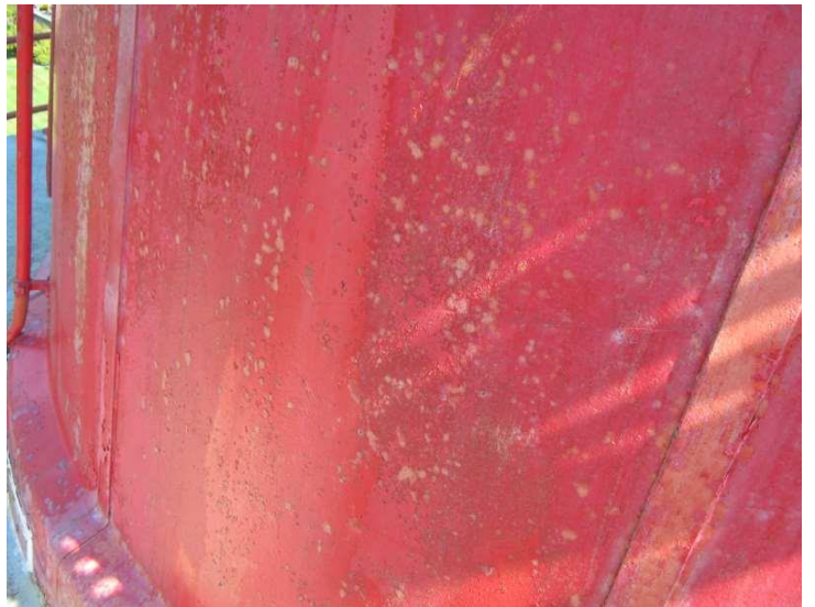
#66 - Lantern House Wall Panel – Crack
