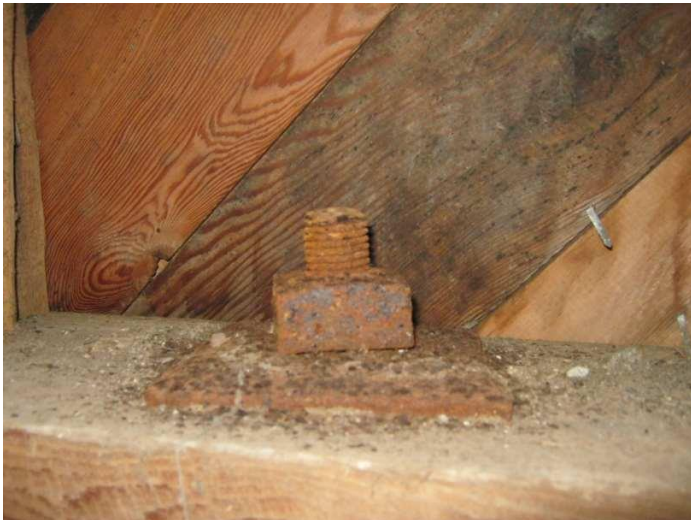
#15 - Anchor Bolt - Corroded
