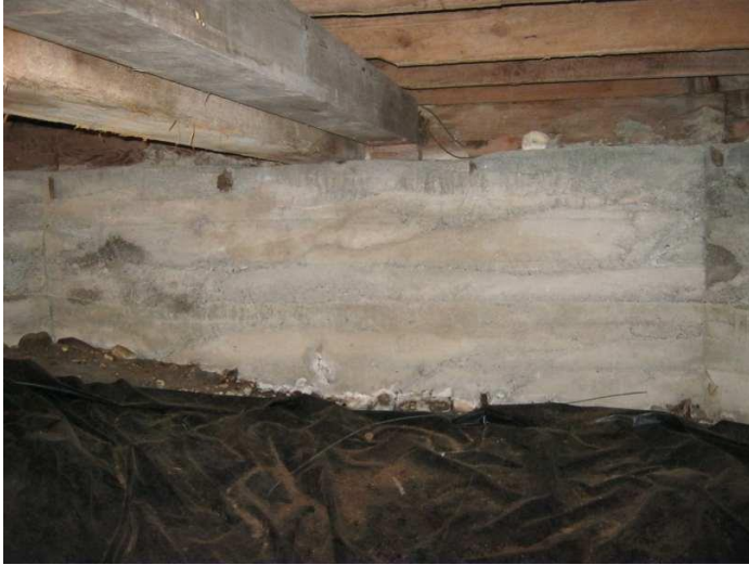
#13 - Foundation Crack - West Wall
