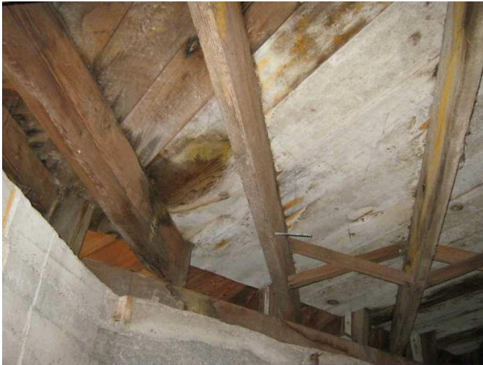
#21 - Main Floor Bridging Missing
