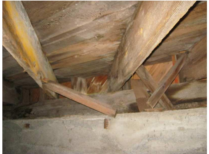
#22 - Main Floor Joist Bridging Deterioration
