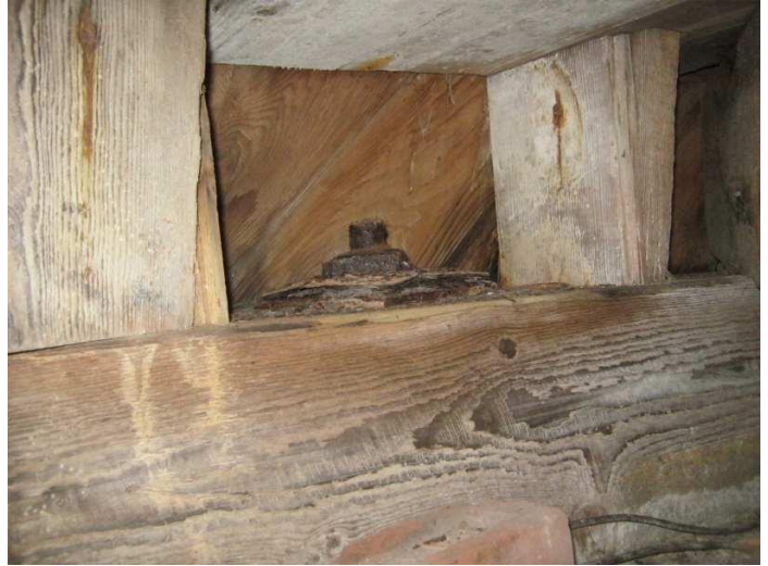
#14 - Anchor Bolt - Corroded
