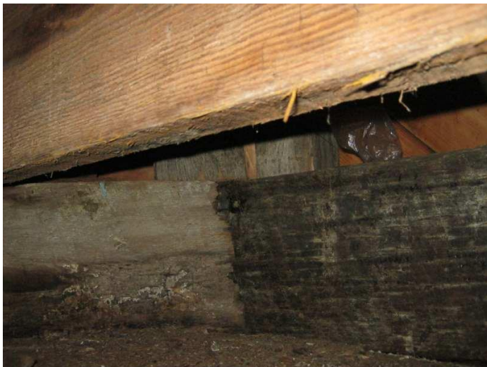
#17 - Bottom Wall Plate - Fire Damage
