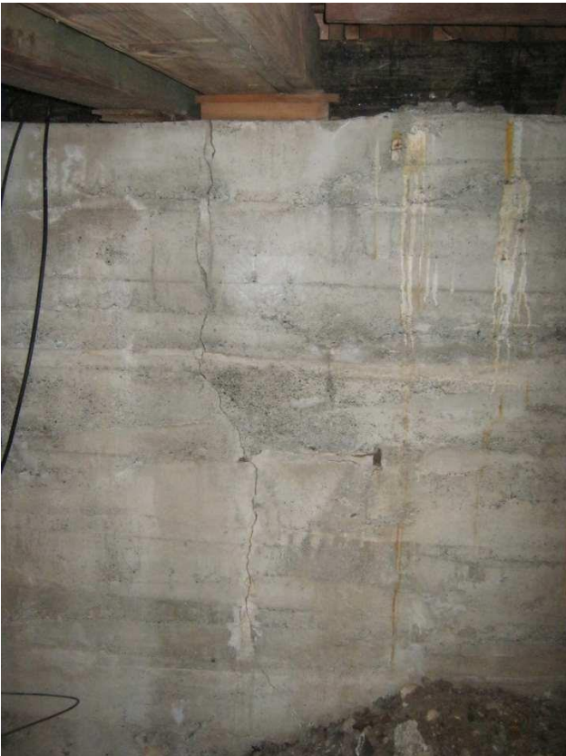
#11 - Foundation Crack - East Wall
