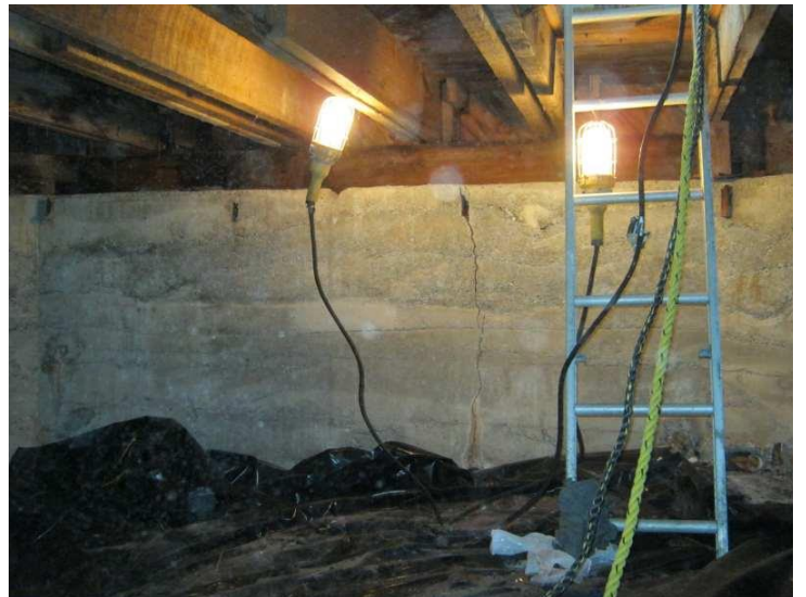
#12 - Foundation Crack - South Wall
