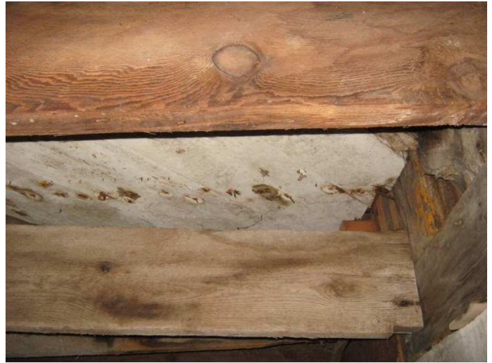
#20 - Main Floor Joist Connection Failed
