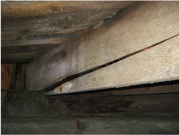
#19 - Main Floor Joist Failed
