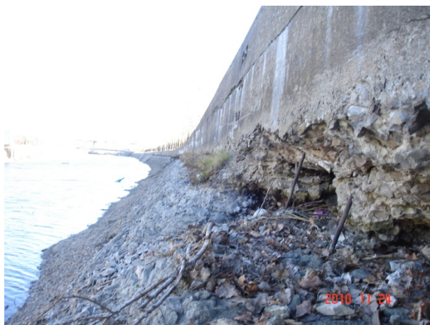
PHOTO 11 - Typical damage to be repaired
