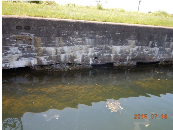
PHOTO 13 - Typical damage to be repaired
