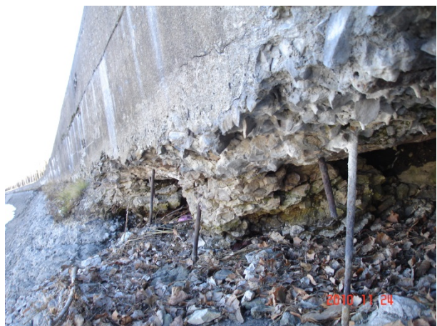
Photo 12 - Typical damage to be repaired
