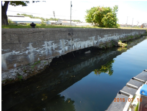
PHOTO 15 - Typical damage to be repaired
