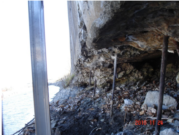
PHOTO 07 - Typical damage to be repaired
