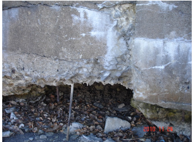
Photo 08 - Typical damage to be repaired
