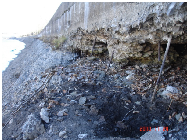
Photo 06- Typical damage to be repaired
