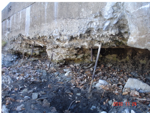
PHOTO 05- Typical damage to be repaired
