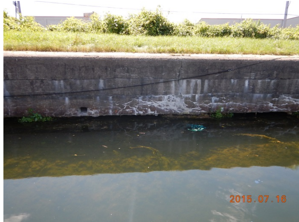
Photo 14 - Typical damage to be repaired rer
