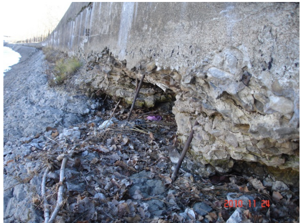
Photo 10- Typical damage to be repaired
