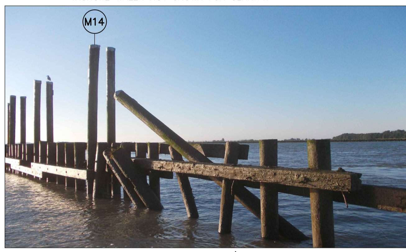
PHOTO No.3 - MISSING/DAMAGED WALL SECTION EAST END
