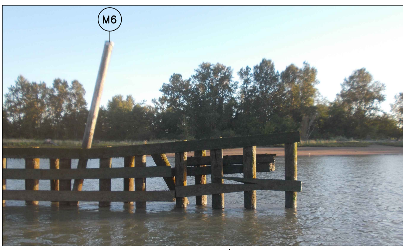
PHOTO No.2 - MISSING/DAMAGED WALL SECTION WEST END
