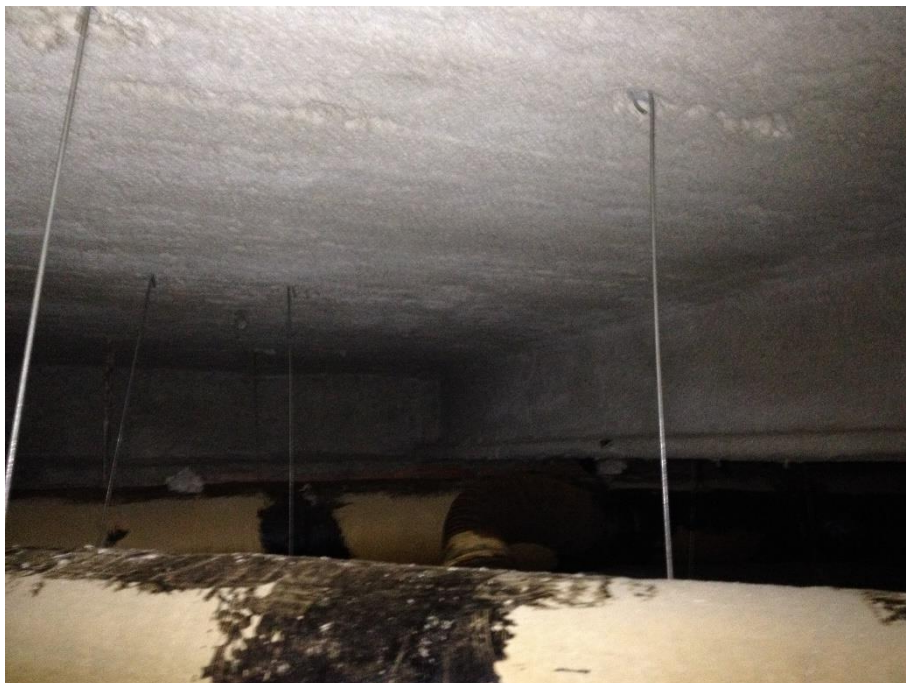
Photo 4: Spray-applied fireproofing was observed on the ceiling deck and structural beams throughout the ground floor south wing. Overspray and debris were also observed throughout.
