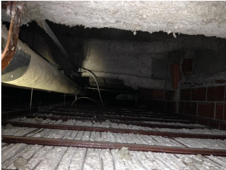
Photo 3: Spray-applied fireproofing was observed on the ceiling deck and structural beams throughout the ground floor south wing. Overspray and debris were also observed throughout.
