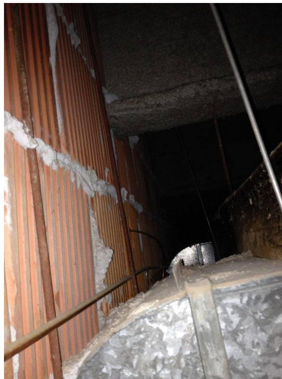
Photo 6: Spray-applied fireproofing was observed on the ceiling deck and structural beams throughout the ground floor south wing. Overspray and debris were also observed throughout.
