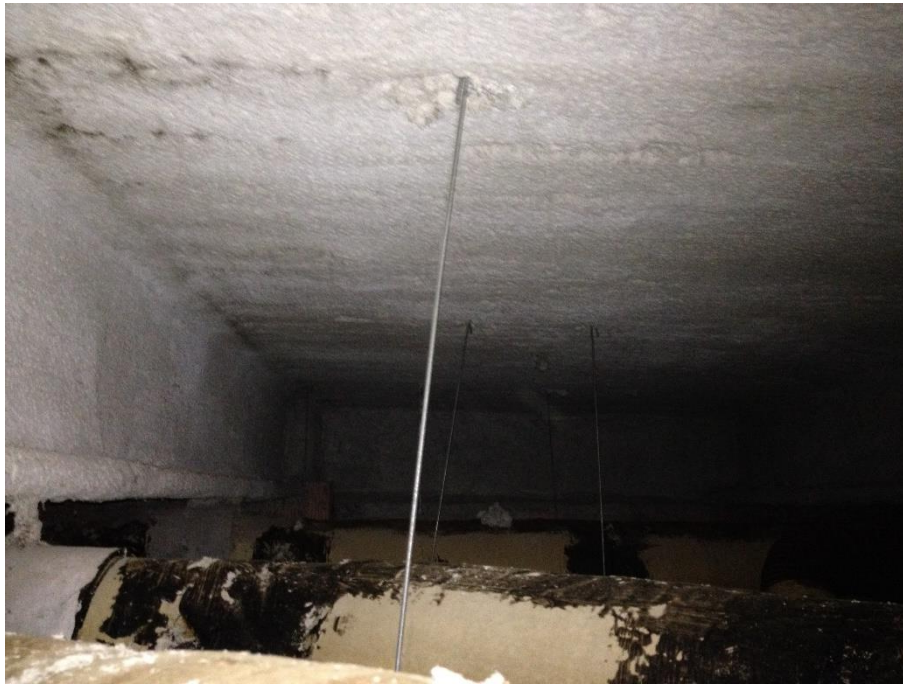
Photo 5: Spray-applied fireproofing was observed on the ceiling deck and structural beams throughout the ground floor south wing. Overspray and debris were also observed throughout.
