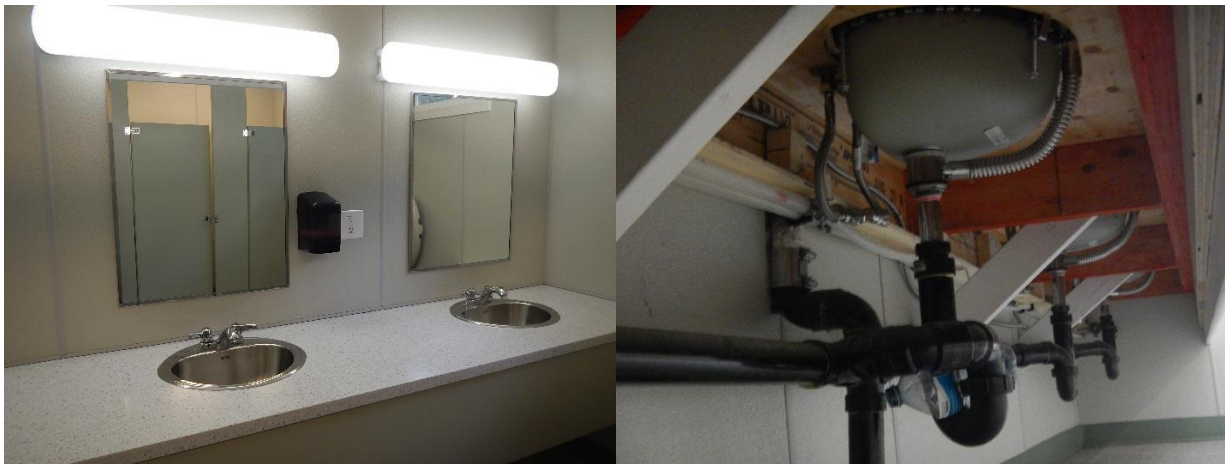
New counter, apron (In current scope, reduce apron to 6"), mirror, lights, sinks, soap dispenser reference
