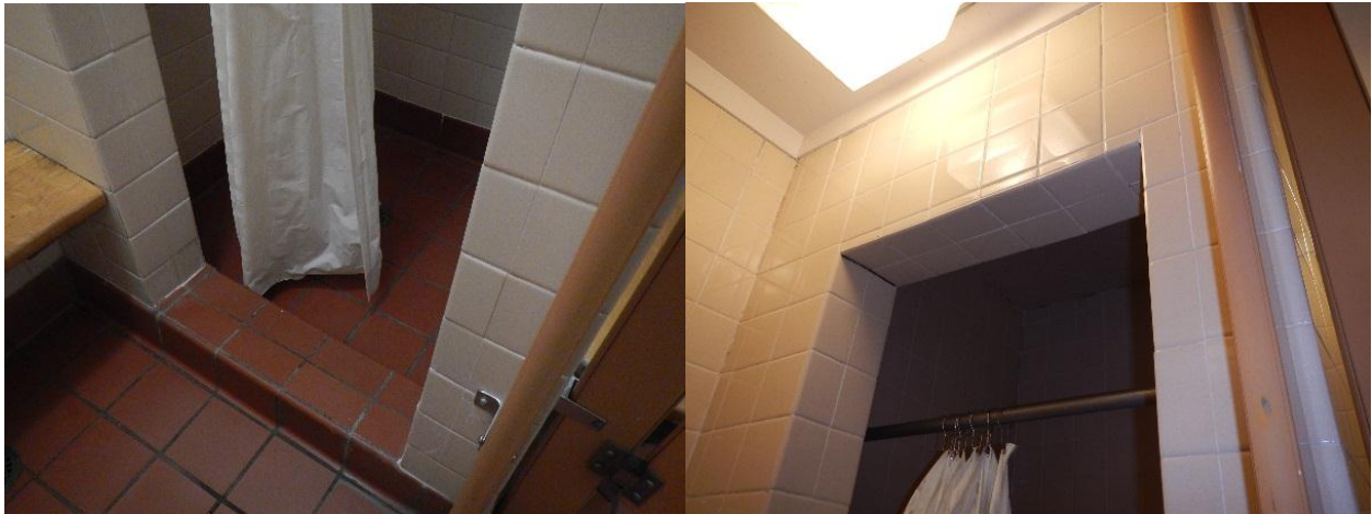
Existing Washroom/Shower Building – Shower stall framing to be demolished and rebuilt suit new shower inserts.
