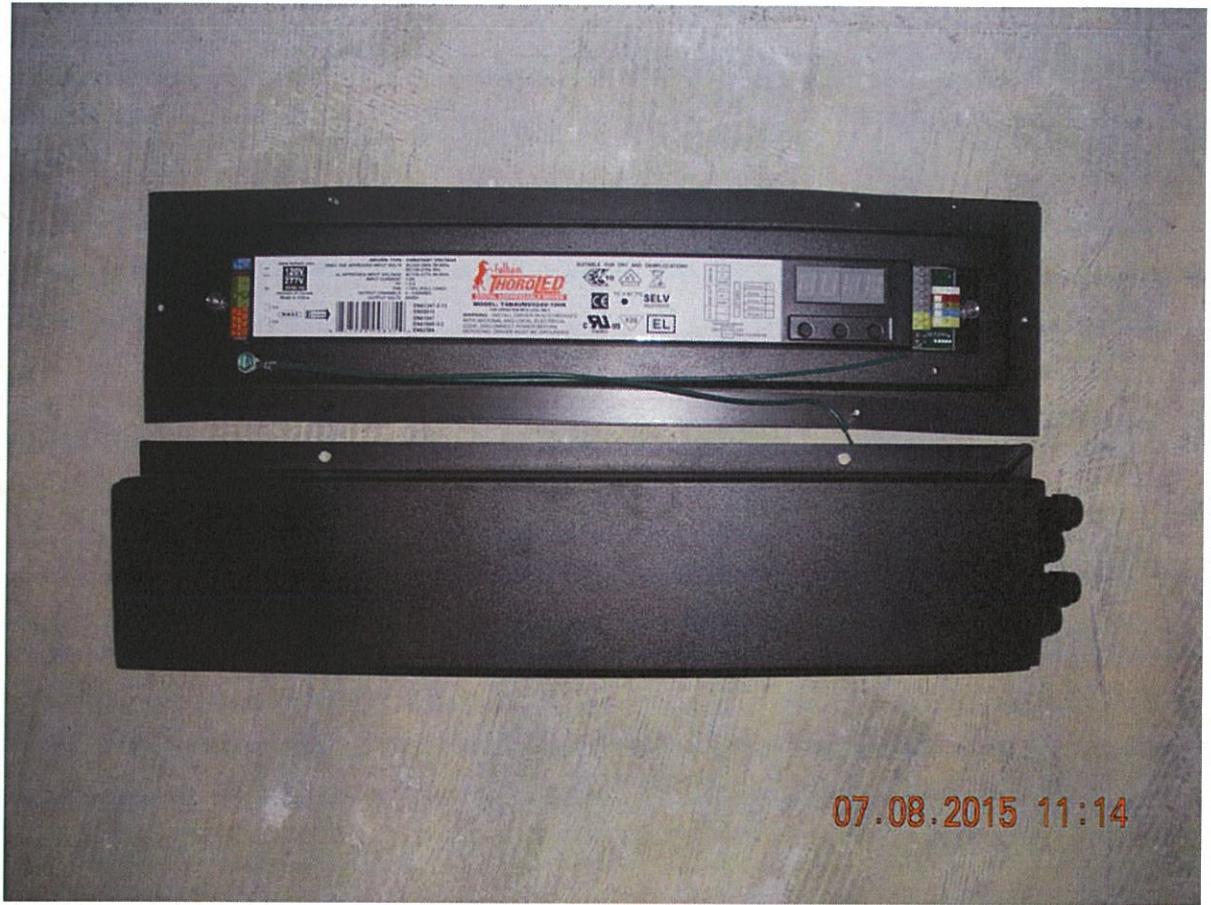
'L2' Luminaire Power Supply with Cover Removed.
