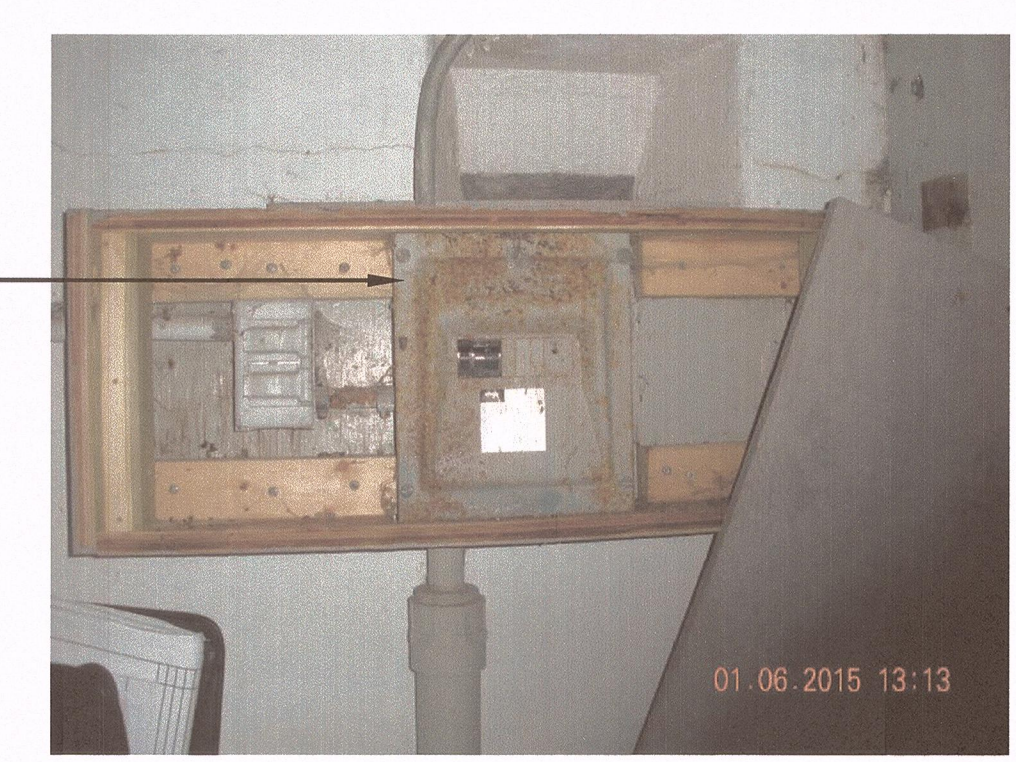
PHOTO #6 - LOWER BATTERY PANEL
