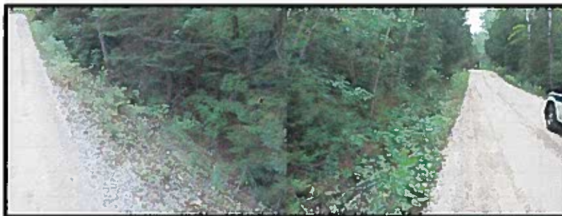
Photo 8- Photo for point 15 showing the steep drop off on the northwest side of the road (1 st photo). Road should be widen to the other side (2 nd photo) where the shoulder is not steep.
