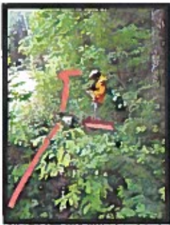
Photo 4- Shows the northeast side of the road at location 3 and 4. Red lines indicate a rough path for the fencing to follow and the red arrow identifies the culvert.
