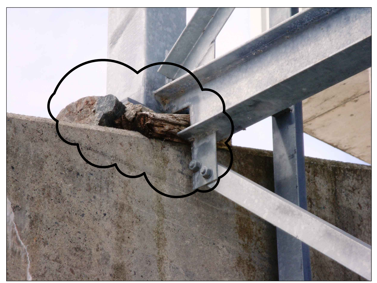
NOTE 7: REMOVE IMPROPER MATERIALS AND FILL REQUIRED AREAS WITH CEMENT OR GROUT TO MATCH EXISTING. REPAIR CUT OUT STEEL WITH PLATE 150mm x 150mm
