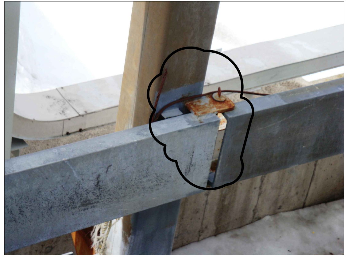
NOTE 3: WELD PLATE ON BACK SIDE OF C CHANNEL ON BOTH SIDES. NO LONGER NEEDED TO SWING. SEE DETAIL ON S-2.02.
