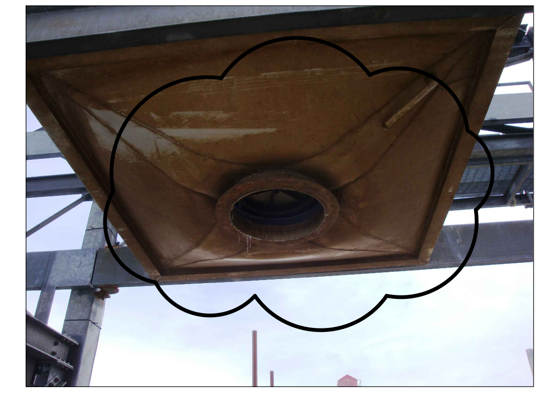
NOTE 5: CUT OUT AND REPLACE BOTTOM OF BASKET WITH 15mm PLATE SLOPED TO EXISTING LATCH FOR FISH CHUTE. SEE DETAIL 5 ON S-3.03
