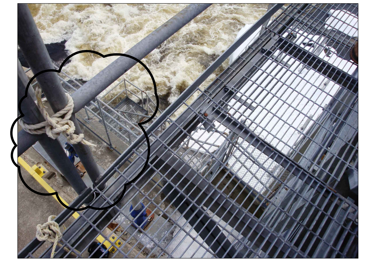
NOTE 6: WELD RAILINGS TO SUPPORT CHANNEL HOUSING TO ELIMINATE MOVEMENT. ENSURE GRATE DECKING PROPERLY SECURED TO SUPPORT CHANNEL
