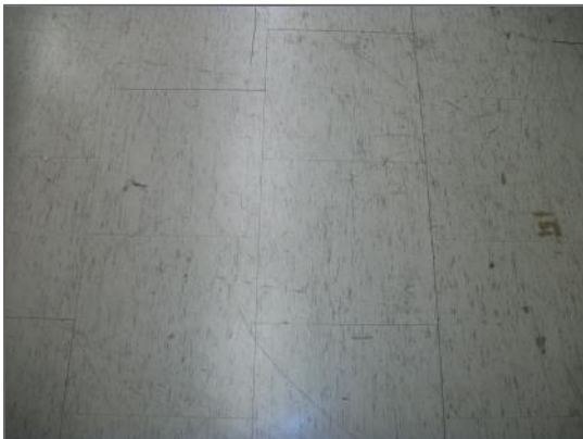
Asbestos-containing 12" x 12" vinyl floor tiles, grey with black streaks, Lab L435
