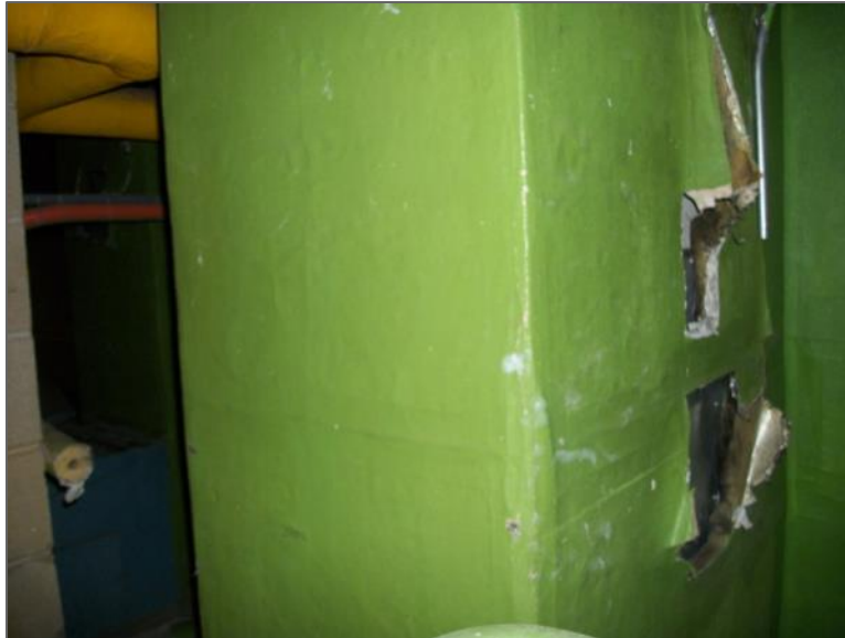
Damaged asbestos-containing paring cement on insulated ductwork, WTC Mechanical Penthouse
