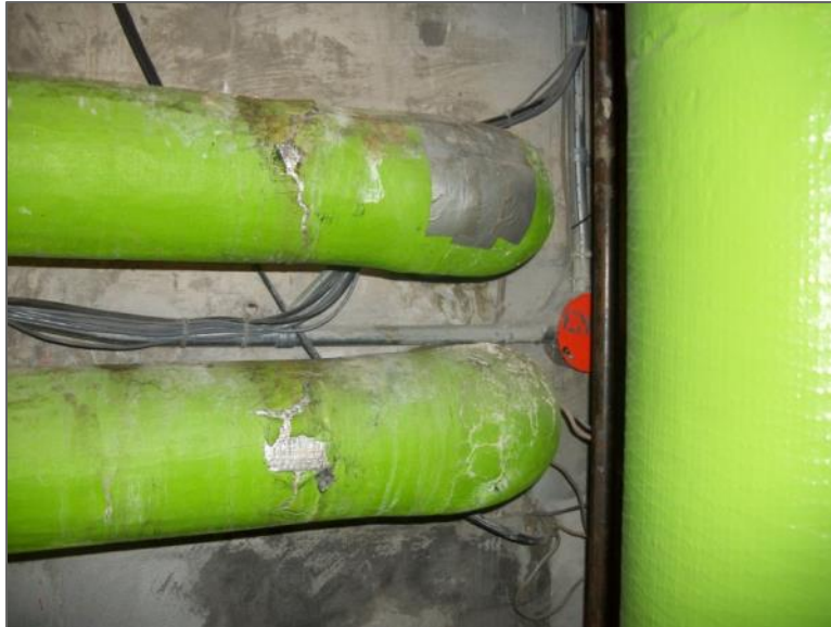
Damaged asbestos-containing parging cement on pipe fittings, Tunnel to WTC at CCIW
