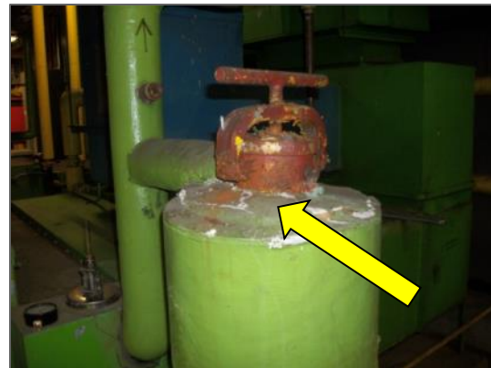
Damaged parging cement fitting at System 5 HVAC unit, R&D Mechanical Penthouse
