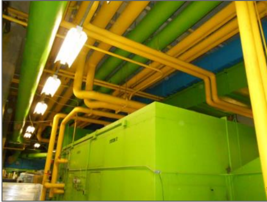
Uninsulated AHU 27, Third Floor Mechanical Penthouse
