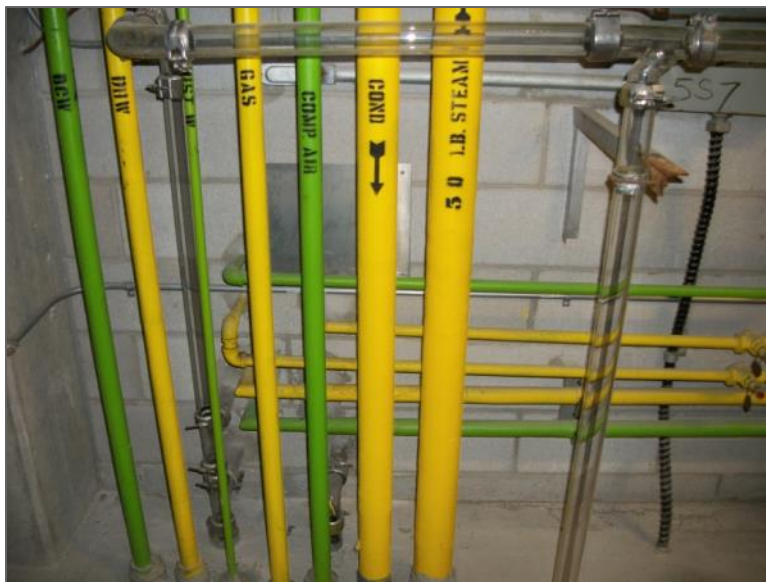
Asbestos-containing magnesia block insulation on condensate pipe straight, Service Core at Laboratory L527
