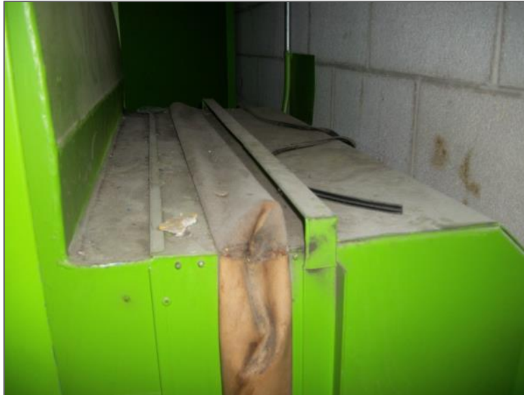
Asbestos-containing parging cement debris on ductwork of abandoned AHU, Equipment Room H245
