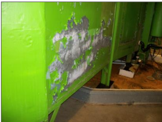
Flaking green paint on the back of AHU 1 in R&D Mechanical
