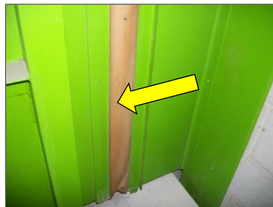
Non-asbestos vibration damper on abandoned AHU, Equipment Room H245
