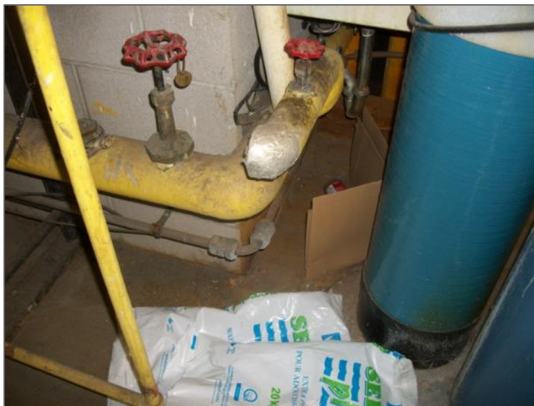
Damaged asbestos-containing parging cement pipe fittings, WTC Mechanical Penthouse
