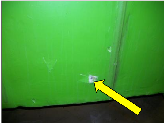
Damaged asbestos-containing parging cement on square ductwork serving System 1, R&D Mechanical Penthouse
