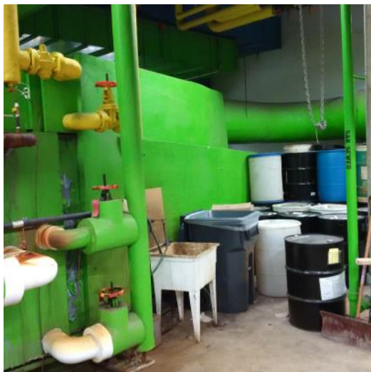
Asbestos-containing paring cement on fibreglass insulated ductwork, AHU 27, Third Floor Mechanical Room
