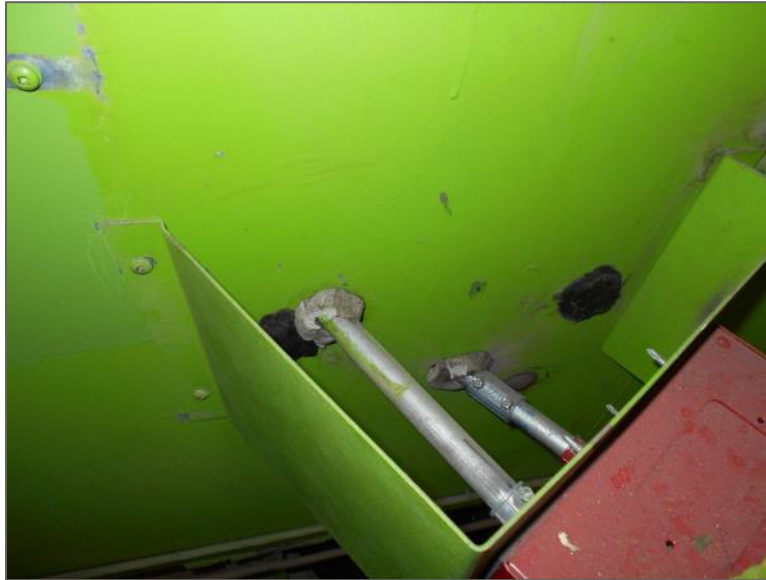
Non-asbestos grey putty at pipe penetrations into AHU 27, Third Floor Mechanical Room
