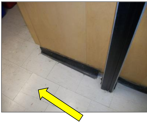
Asbestos-containing vinyl floor tiles, Lab H530
