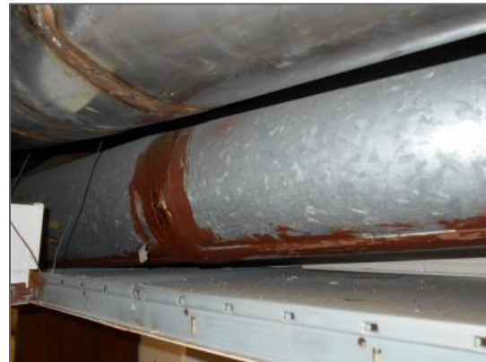
Asbestos-containing brown mastic on redundant metal exhaust duct, Lab L435
