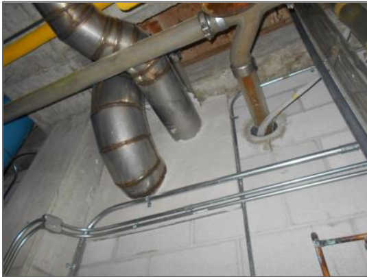
Non-asbestos rough plaster at duct penetration through wall, Seventh Floor South Service Corridor
