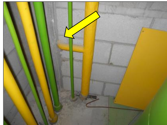
Asbestos-containing paring cement on pipe fitting, North end of Sixth Floor South Service Corridor
