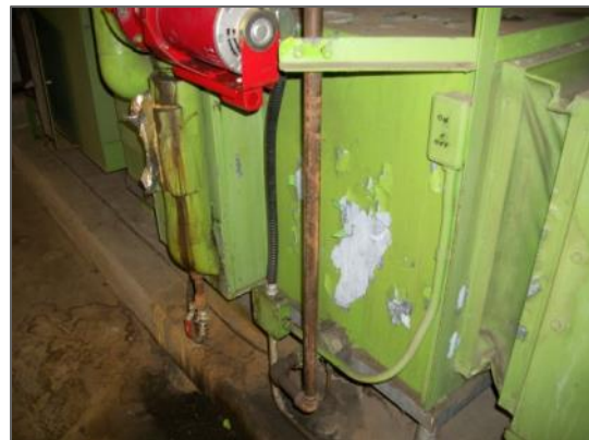
Flaking green paint on the AHU 3 in R&D Mechanical
