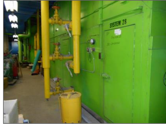
Uninsulated AHU 28, Third Floor Mechanical Penthouse
