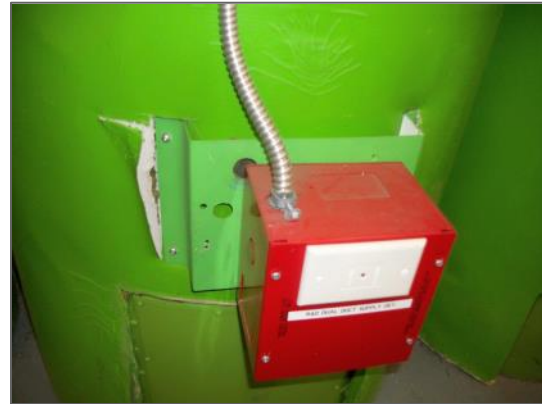
Asbestos-containing paper on two centre round hot ducts serving System 1, R&D Mechanical Penthouse
