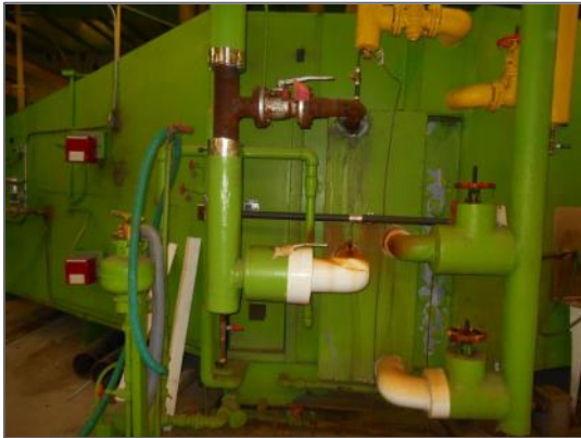
Flaking lead-containing green paint on AHU 27, Third Floor Mechanical Room
