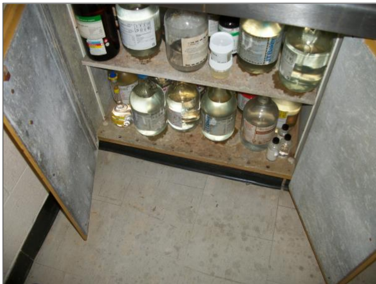
Transite board lining acid/base cabinet below fume hood, Laboratory L530
