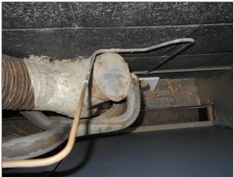
Asbestos-containing brown mastic on ductwork in fan unit, Fifth Floor Office L529
