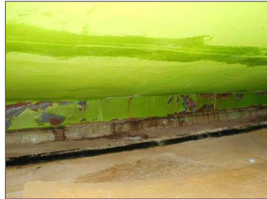
Flaking lead-containing green paint below ductwork on AHU 28, Third Floor Mechanical Room
