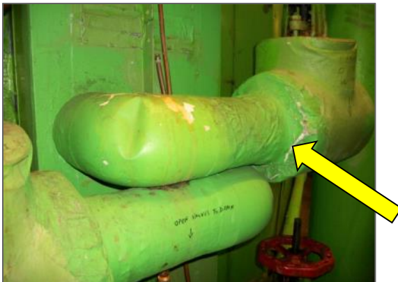
Damaged parging cement fitting behind System 1 HVAC unit, R&D Mechanical Penthouse
