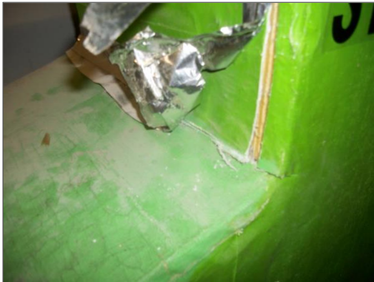
Asbestos-containing parging cement on insulated ductwork, Hydraulics Mezzanine Catwalk/Corridor Mechanical Area at Offices
