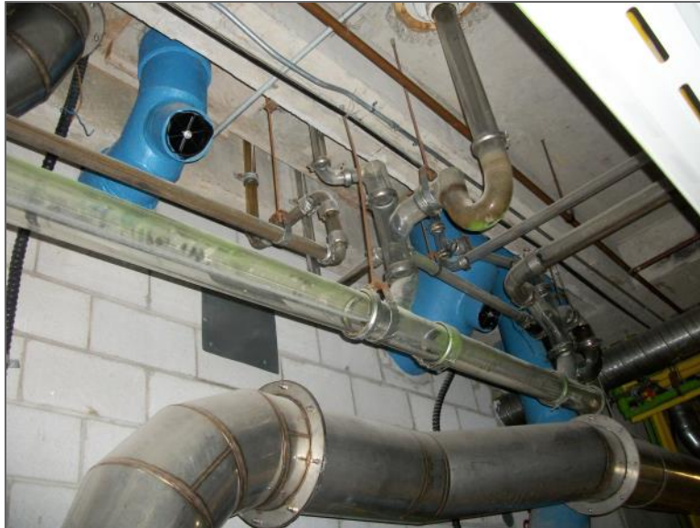
Transite exhaust serving Laboratory L530, Adjacent Service Core
