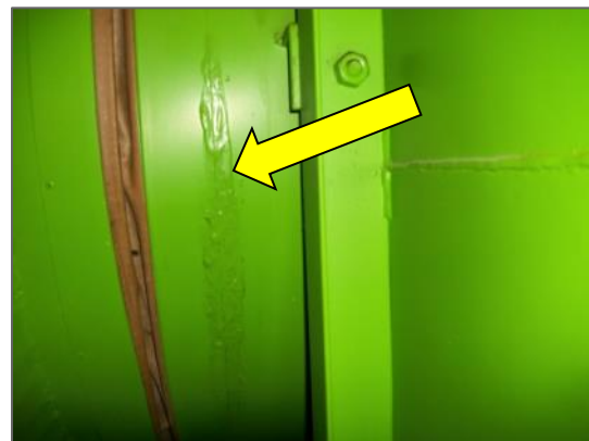
Painted asbestos-containing brown mastic on abandoned AHU, Equipment Room H245
