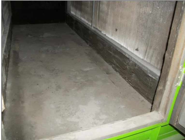
Non-asbestos black mastic on fibreglass insulation within abandoned AHU, Equipment Room H245
