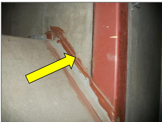
Asbestos-containing red mastic at joints of AHU 1, R&D Mechanical Penthouse
