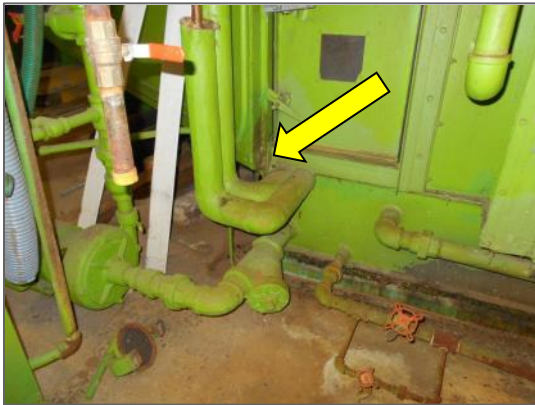
Asbestos-containing paring cement on pipe fittings at AHU 27, Third Floor Mechanical Penthouse
