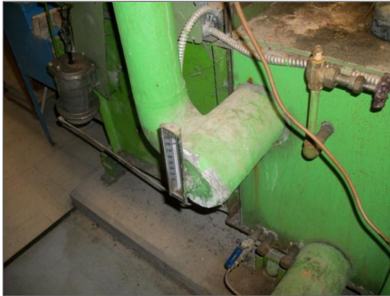
Asbestos-containing parging cement insulation on fitting, Hydraulics Mezzanine Catwalk/Corridor Mechanical Area at Offices
