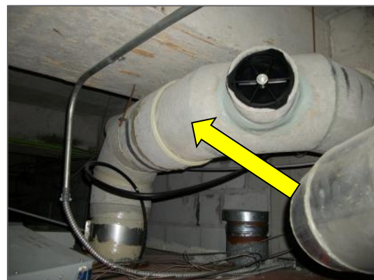
Transite pipe exhaust from fume hood, Laboratory L530
