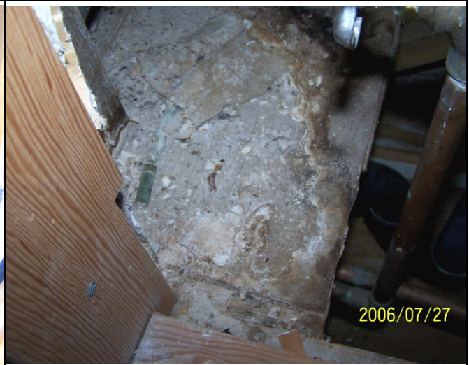
Figure 22: Second Floor Bedroom – Access Hatch to bathtub plumbing shows mould staining on floor from water damage.
