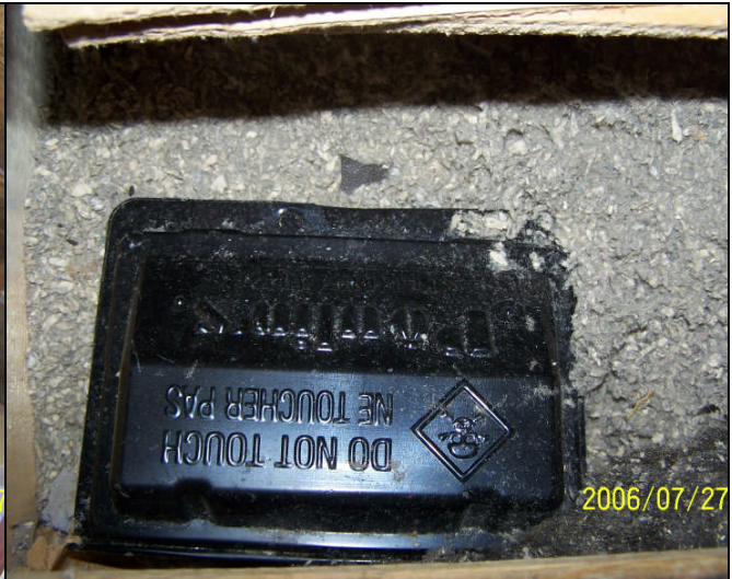
Figure 18: Second Floor Attic Area (off Bedroom) – Mouse bait station in Attic
