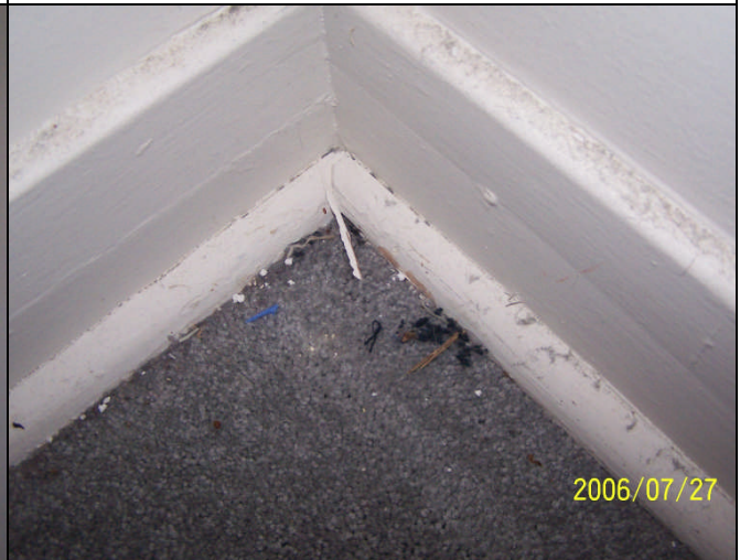
Figure 16: Second Floor Bedroom – Feces (mouse) on bedroom floor
