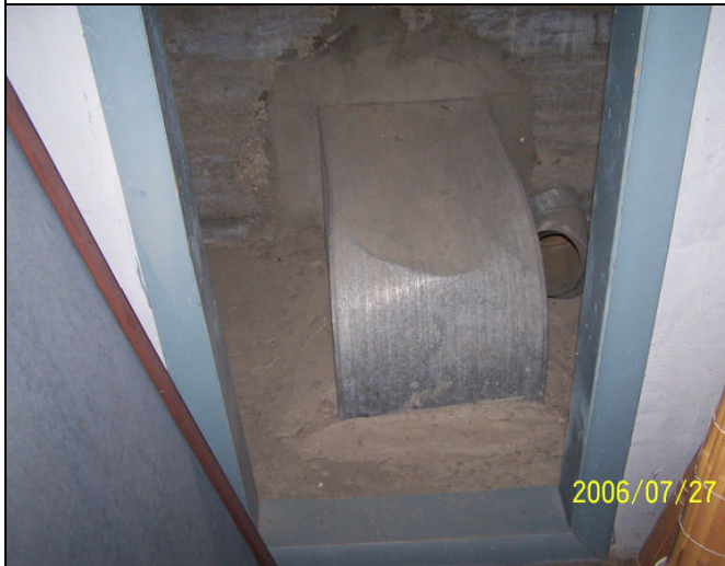
Figure 11: Basement – Abandoned (suspect return air) duct (possibly for a former furnace system).
