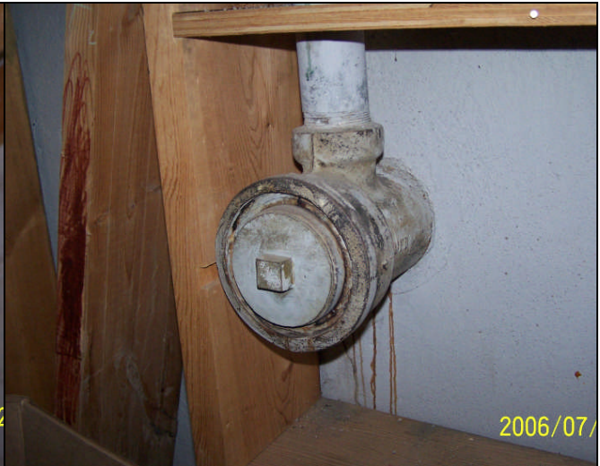
Figure 10: Basement – Dripping around Septic cleanout causing water pooling on Basement floor.
