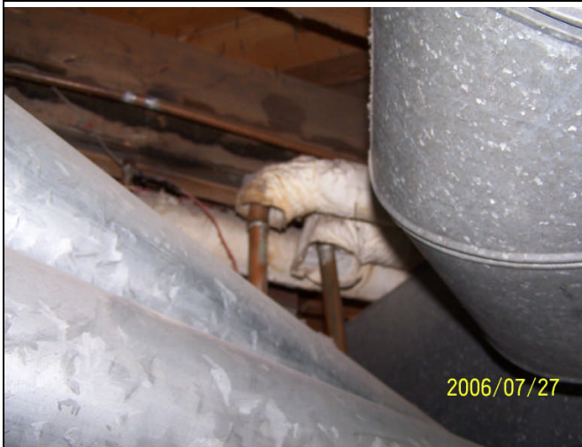
Figure 1: Basement – Suspect asbestos-containing fittings
