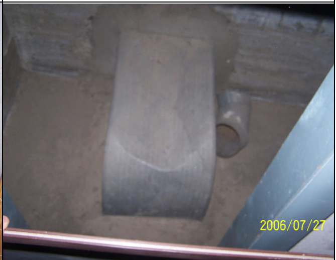
Figure 12: Basement – Abandoned (suspect return air) duct
