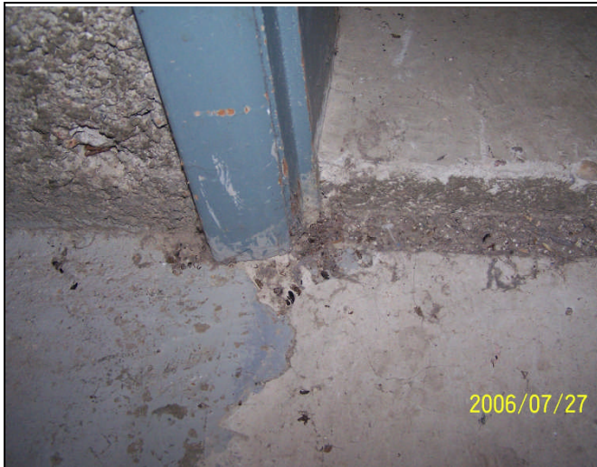
Figure 5: Basement – Feces (mouse) and dryer lint
