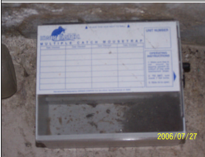
Figure 3: Basement – Mouse trap containing nesting material or carcasses
