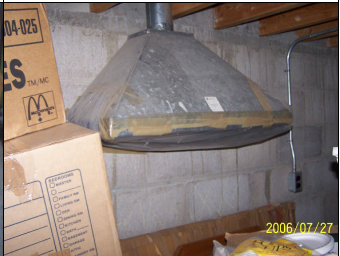
Figure 8: Basement – Fume hood may contain asbestos
