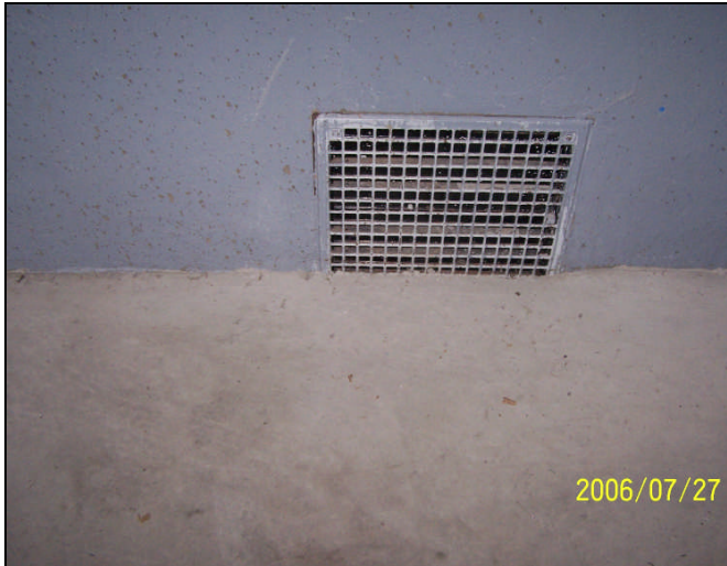
Figure 13: Basement – Vent for abandoned (return air) duct
