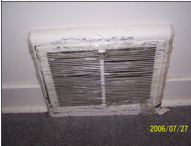
Figure 19: Second Floor Bedroom – Air vent blocked to prevent rodent entry
