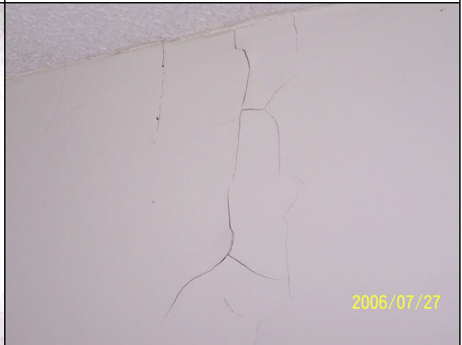
Figure 24: Second Floor Bedroom – Moisture damage to wall causing paint and plaster cracking
