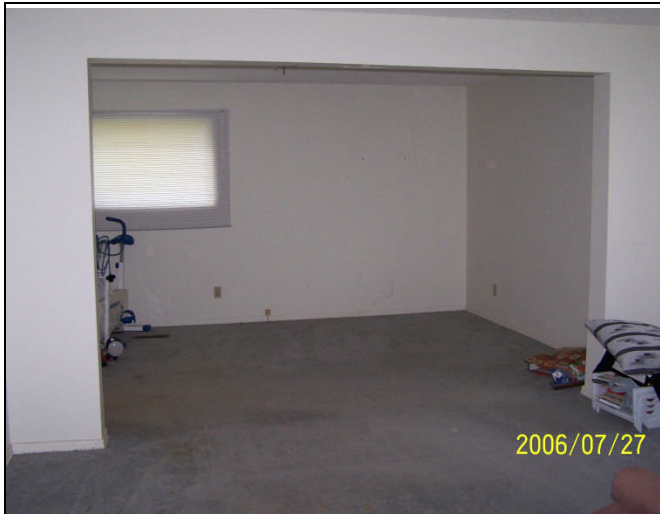
Figure 32: Living Room – Mice reportedly seen crossing floor on numerous occasions.
