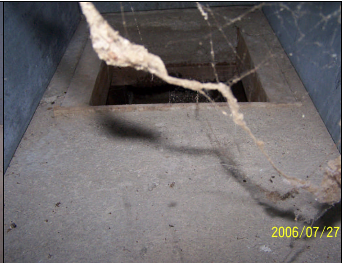
Figure 14: Basement – Interior view into duct (enables air entry from beneath slab floor). Suspect building access for rodents.
