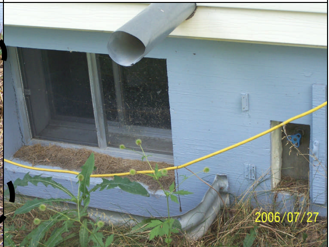
Figure 39: Building Exterior – Uncapped (Open) Dryer Vent (enables interior access by rodents)
