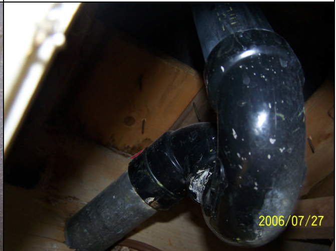
Figure 35: Living Room (Access Hatch) – Removal Access Panel identified trap for bathtub drain (second level).
