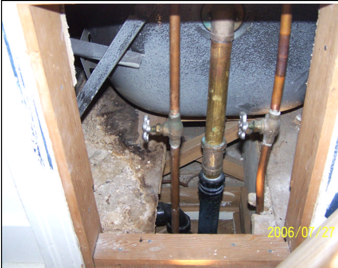
Figure 21: Second Floor Bedroom – Access Hatch to bathtub plumbing
