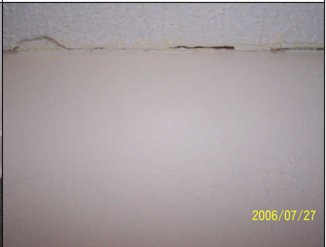
Figure 20: Second Floor Bedroom – Water damaged ceiling and paint cracking on wall
