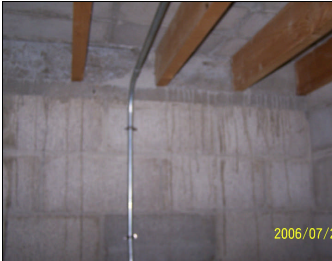
Figure 9: Basement – Drip lines indicating water seepage
