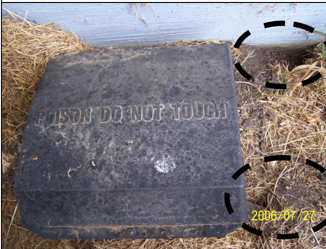
Figure 38: Building Exterior – Mouse Poison (two mouse holes visible beside poison container)
