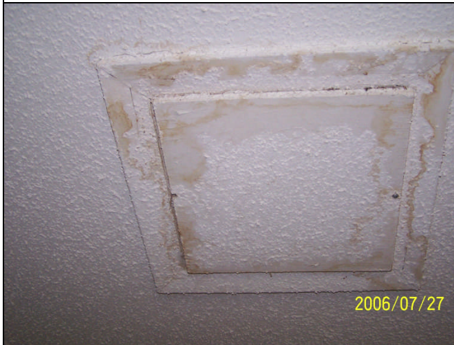
Figure 34: Living Room (Access Hatch) – Water reportedly poured from Access Hatch in Living Area below. Water staining evident on and around Access Hatch.
