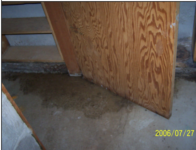
Figure 7: Basement – Water seepage on slab floor
