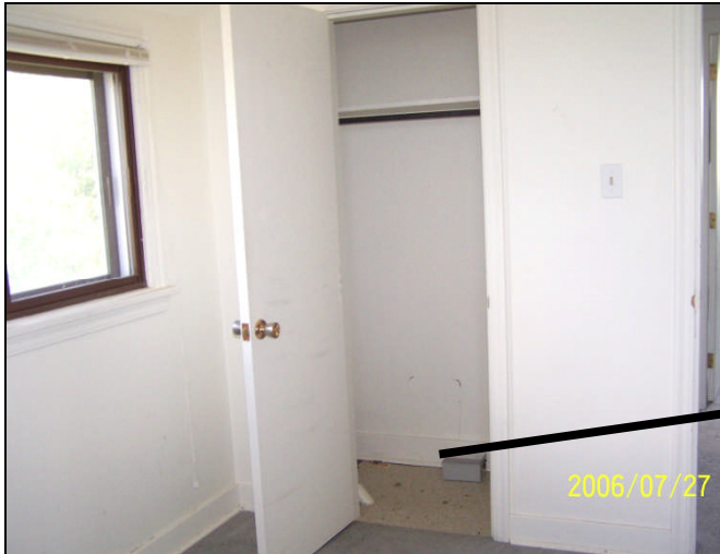
Figure 25: Second Floor Bedroom Closet – Contained three mouse traps
