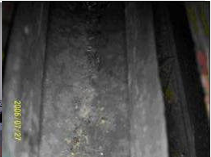
Figure 33: Living Room – Feces (mouse) visible in floor registers.
