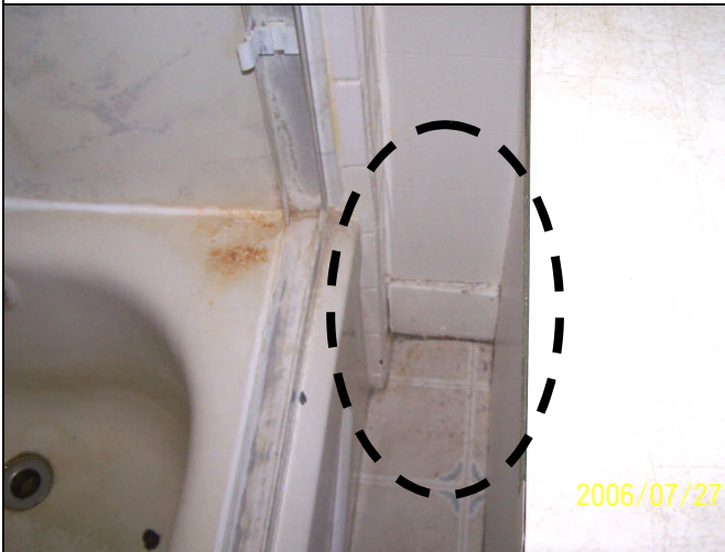
Figure 23: Second Floor Washroom – Suspect mould growth beside bathtub.
