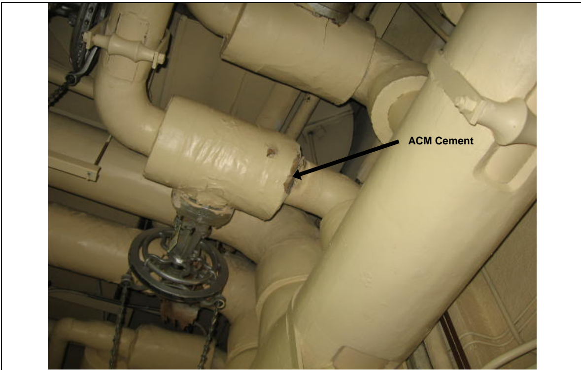
Photograph 11: ACM cement on end of fiberglass-insulated pipe valve. Room No. SB-1 (Sample No. ACM 38)
