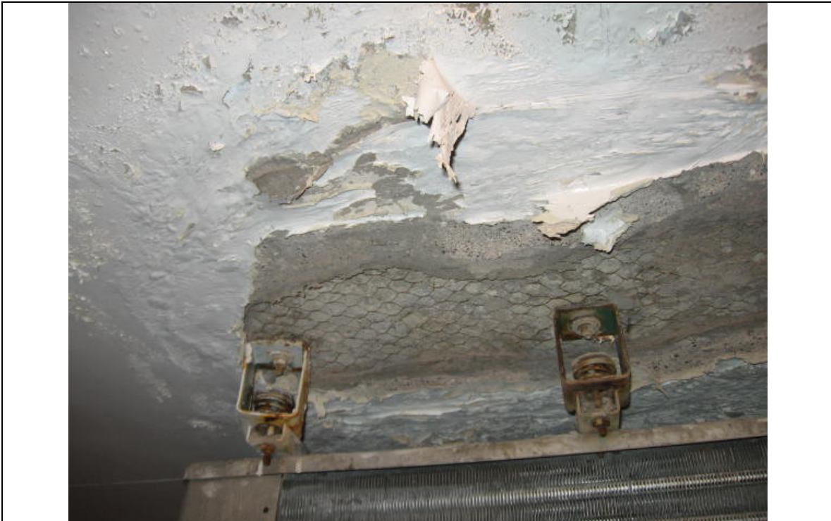
Photograph 15: Damaged plaster ceiling in Room No. B-21 (Freezer Room). (Sample No. ACM 47). Note that although analysis of this material showed no asbestos was detected, material should be treated as asbestos based on positive results of similar samples and non-homogeneous nature of material.
