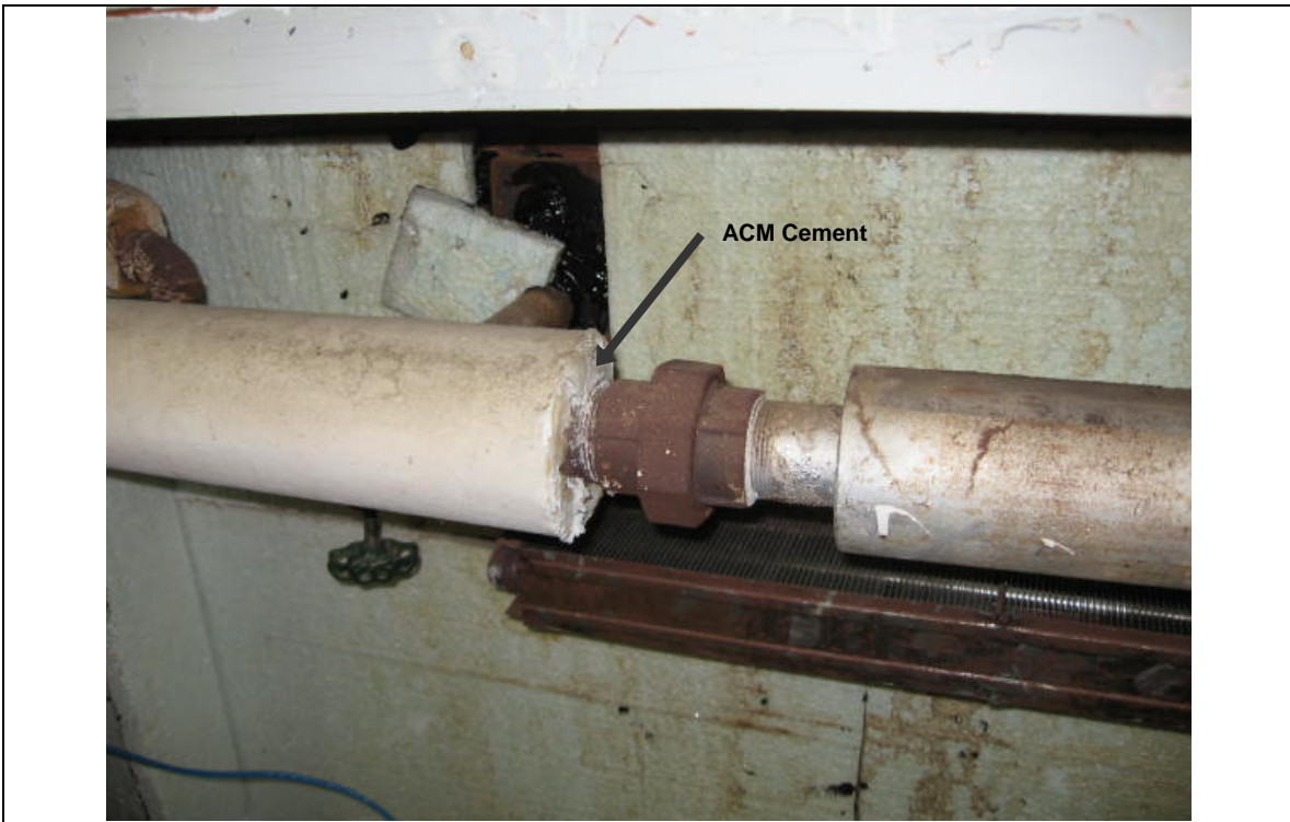
Photograph 9: ACM cement on end of fiberglass pipe wrap in Room No. 1-10 (Sample No. ACM 30).
