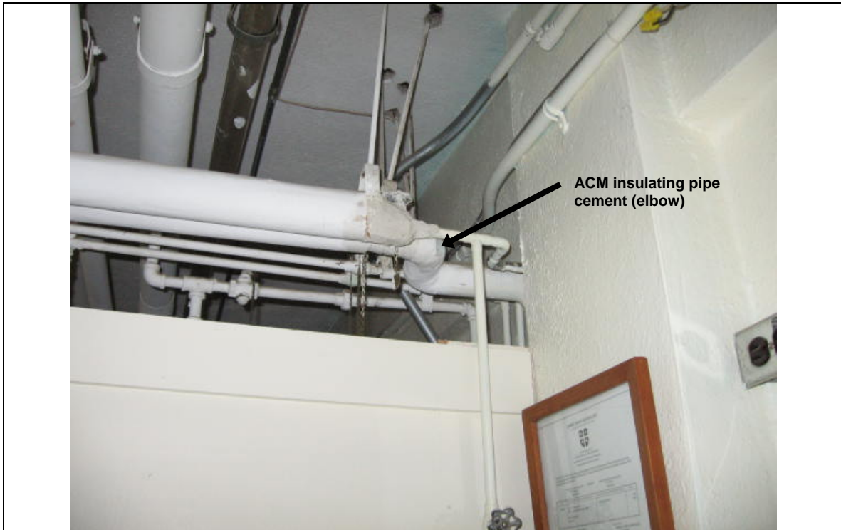
Photograph 17: ACM insulating pipe cement (elbow). Room No. B-25 (sample No. ACM 49)
