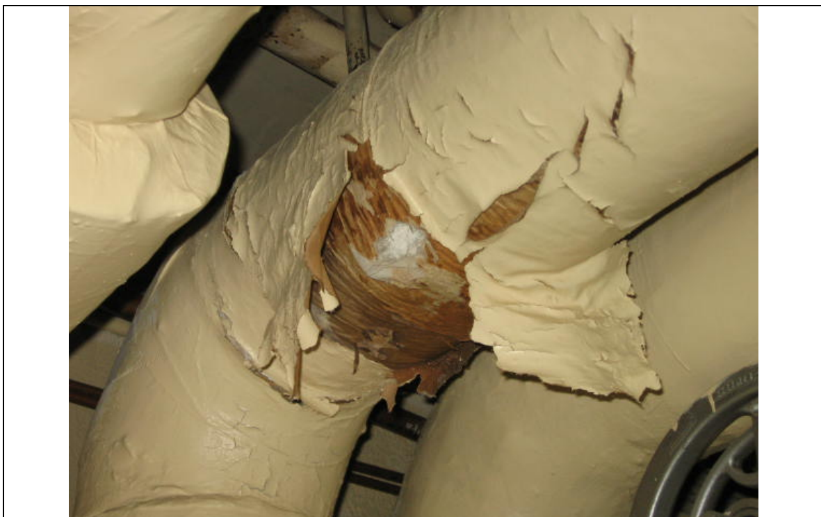
Photograph 6: ACM pipe insulation on overhead 300 mm dia. steam header piping. Room No. SB-1. (Sample No. ACM 19).
