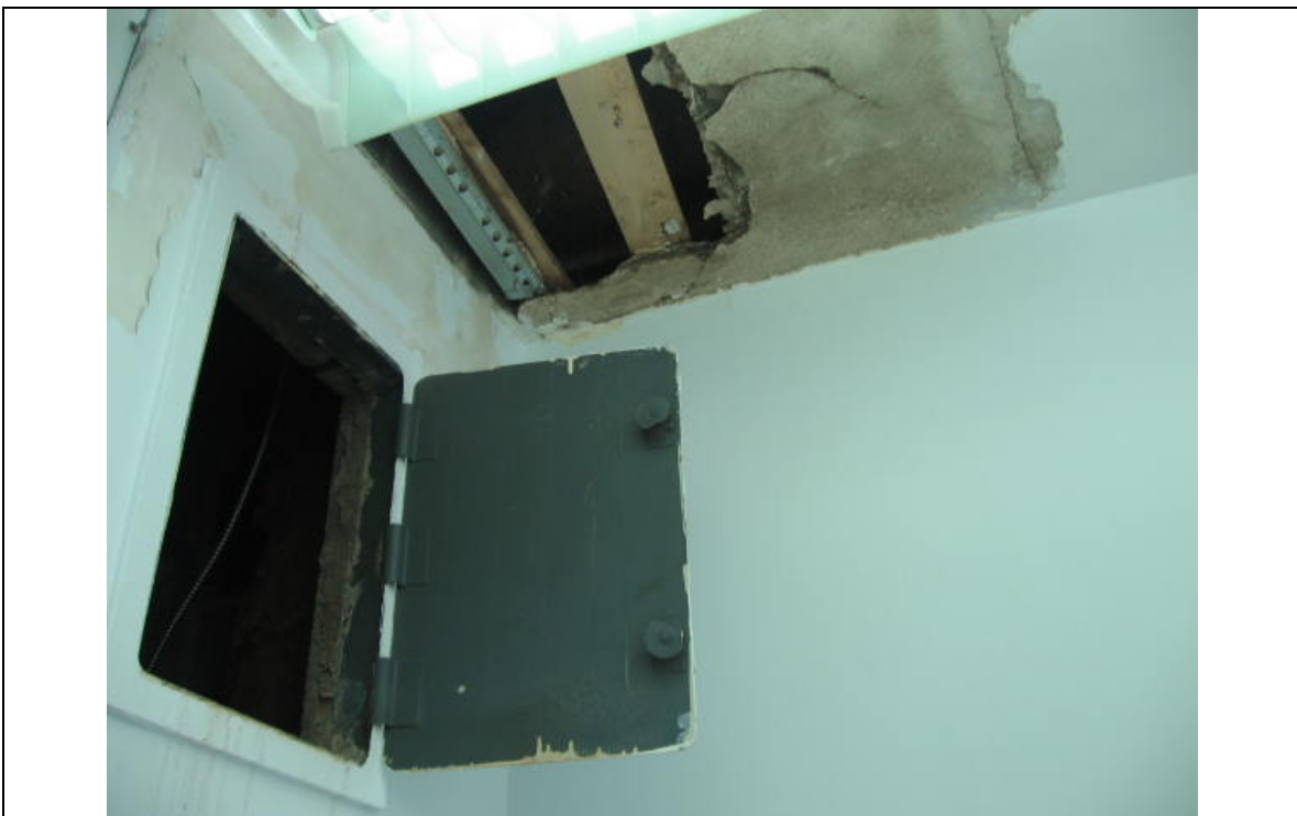
Photograph 12: Damaged ACM plaster ceiling, Room No. 1-16.
