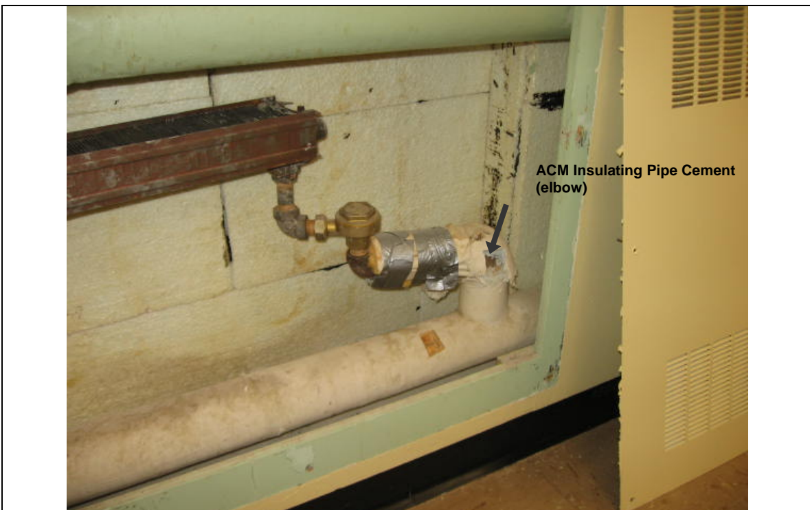
Photograph 8: ACM insulating pipe cement (elbow), located behind metal heater cover in Room No. 1-4. (Sample No. ACM 25).
