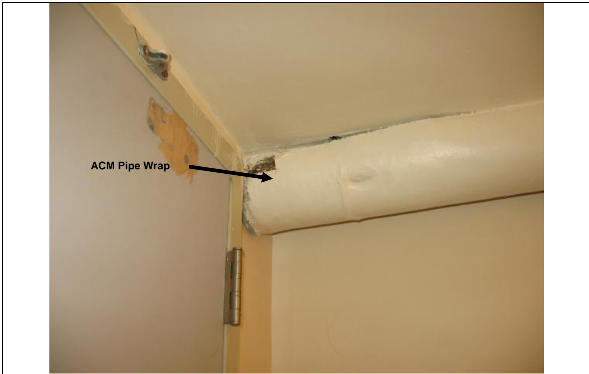
Photograph 3: ACM pipe wrap insulation, corrugated paper-type, Room No. SB-7. (Sample No. ACM 14)
