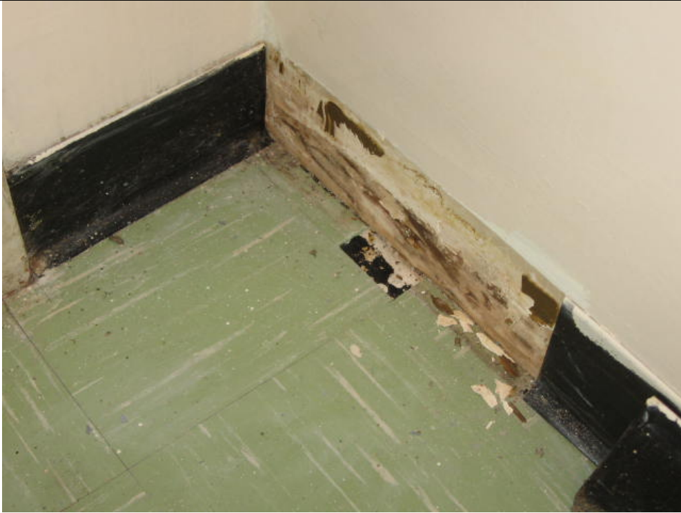
Photograph 1: Asbestos containing material (ACM), 23 x 23 cm, vinyl floor tile, Room No. SB-7 (Sample No. ACM 2). Note that eight other colours of ACM floor tile are also present in the building (no photos provided).
