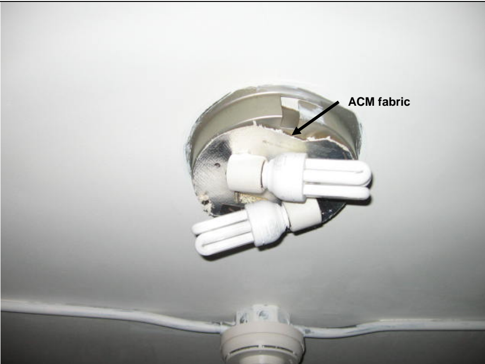
Photograph 2: ACM fabric on ceiling light fixture, Room No. SB-7. (Sample No. ACM 13)
