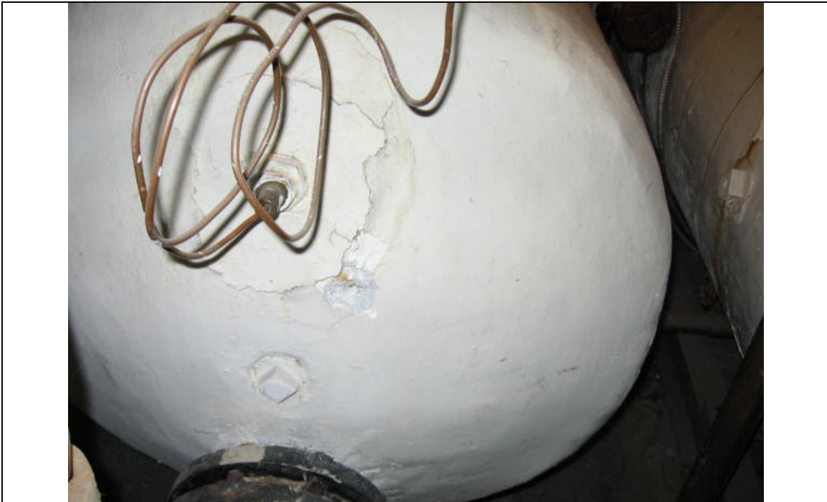
Photograph 7: ACM hot water tank insulation (2 tanks), Room No. B-2 (Sample No. ACM 22).
