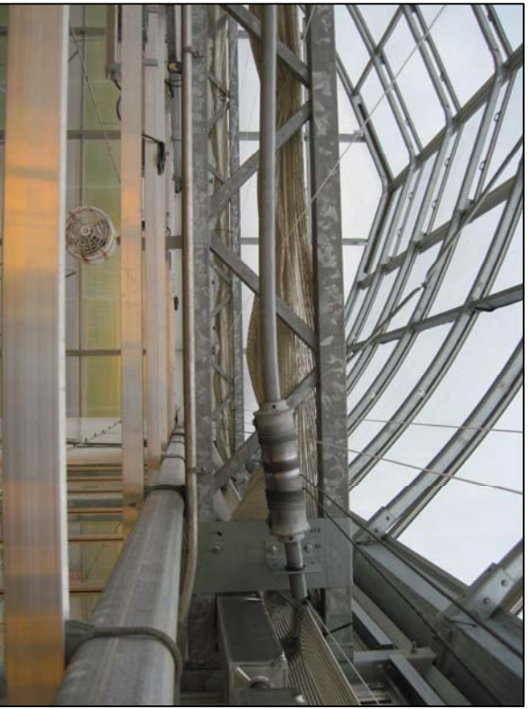
VIEW OF BENT DRIVE SHAFT IN GREENHOUSE A-2
