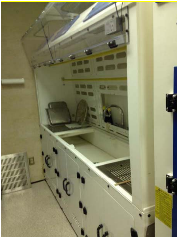
Figure #1 Fume Hood to be removed and reconnected-Refer to Phase II – Main Floor Demo.
