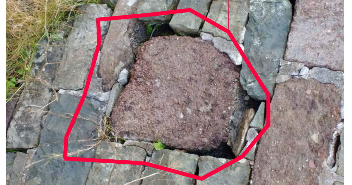
PHOTO 12-PORTAL LOSE AT JOINTS-BEDDING
