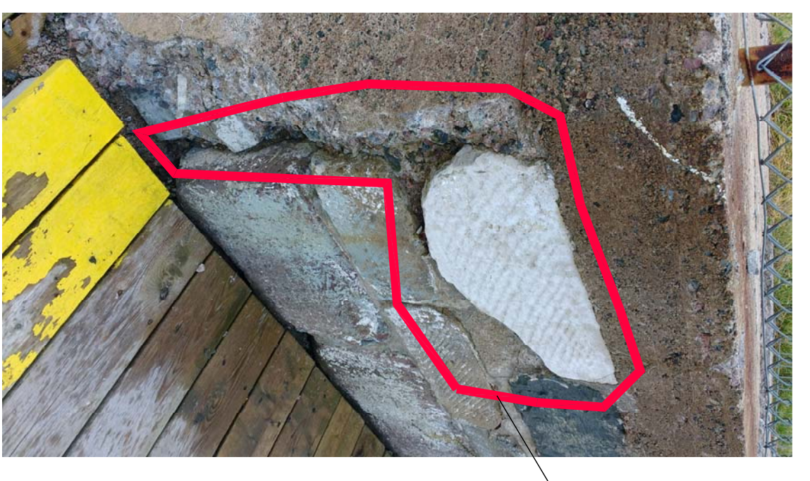
PHOTO 14-MASONRY JOINTS WITH CONCRETE DETRIORATION
