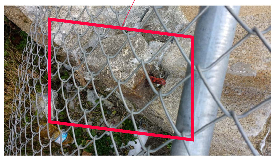
PHOTO 22-CORRODED REBAR INSIDE WALL
