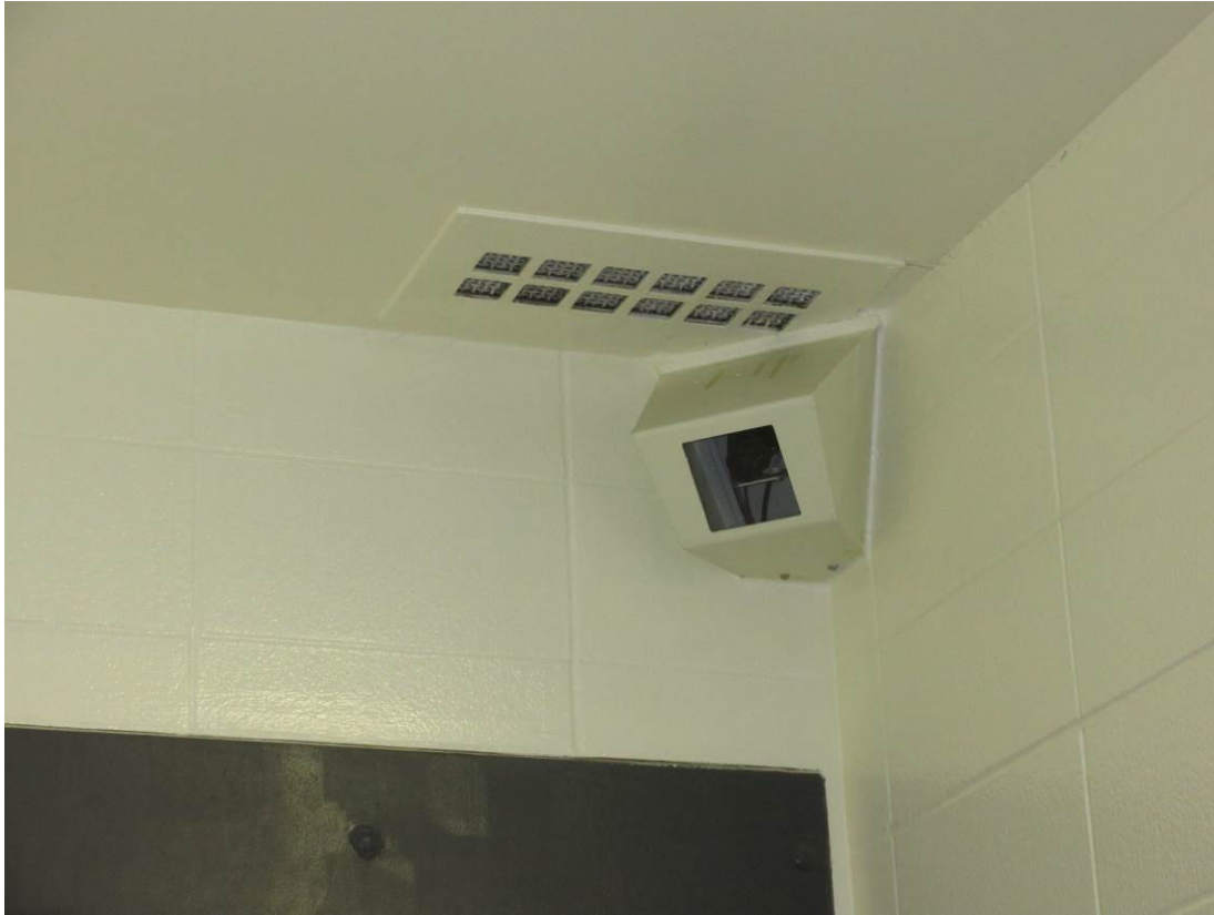
Photo 5 - Typical security camera housing and security grill
