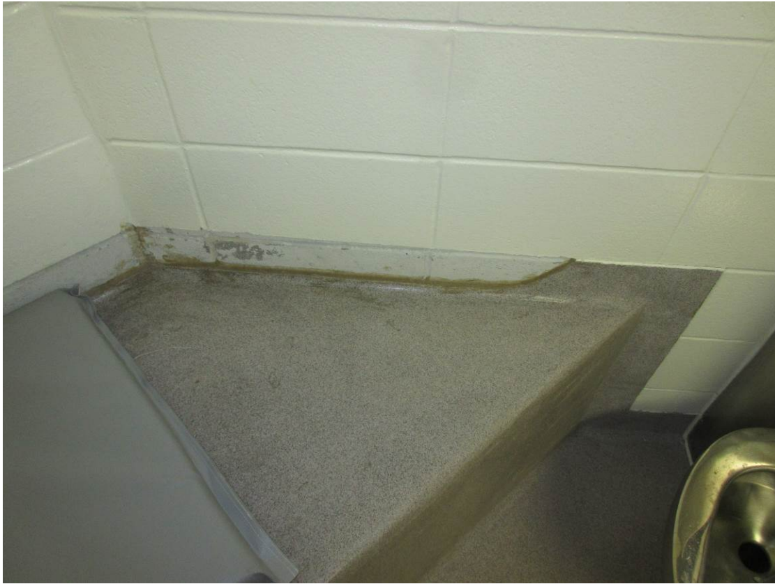
Photo 1 – Damaged Epoxy Cove
