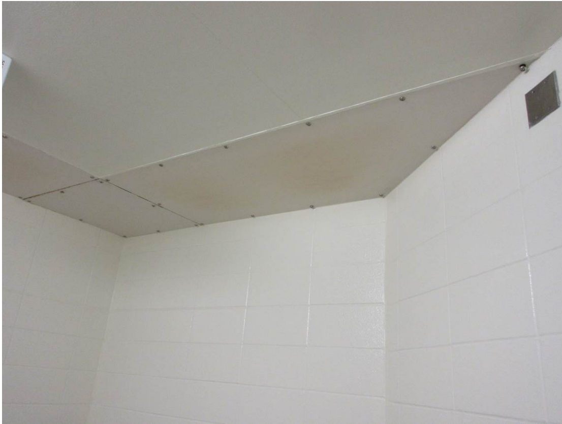
Photo 3 - Typical radiant panel – Caulk at Joints with Security Caulk and Replace Missing Fasteners
