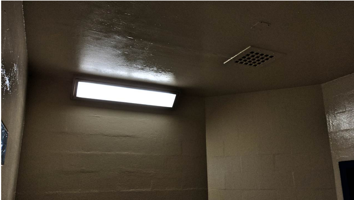
Photo 3 - Typical Light and Ceiling Grill
