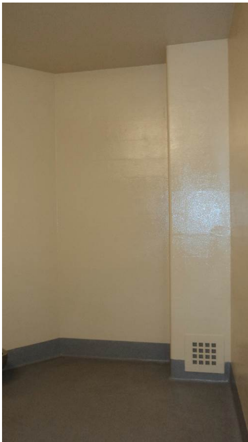
Photo 2 - Typical Wall Grill
