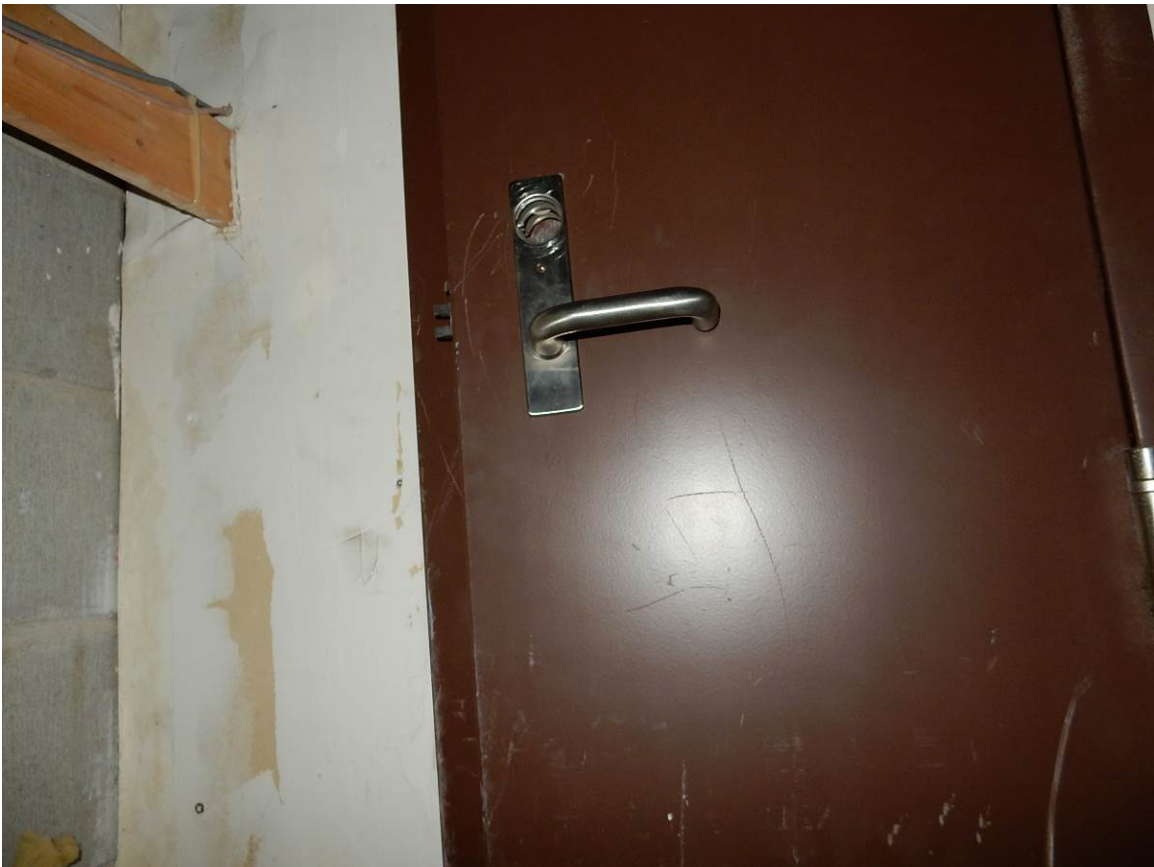
Photo 10 - Damaged Attic Door
