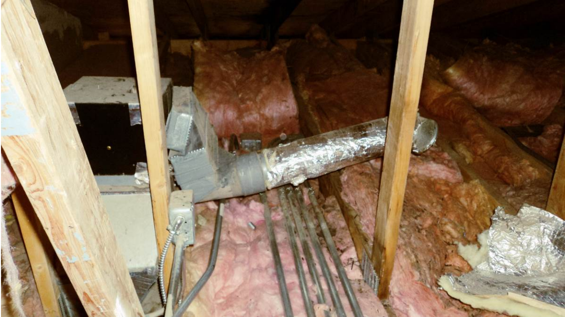
Photo 7 - Damaged Exhaust Fan in Attic
