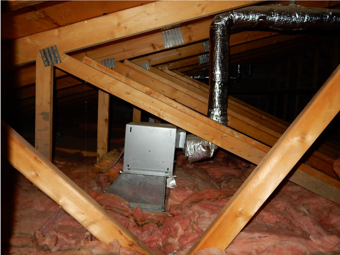
Photo 11 - Typical Exhaust Fan
