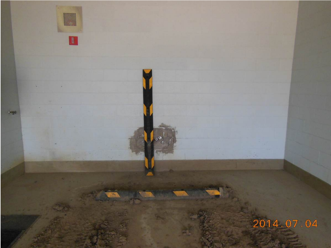
Photo 1 – Damage to Wall in Room 113
