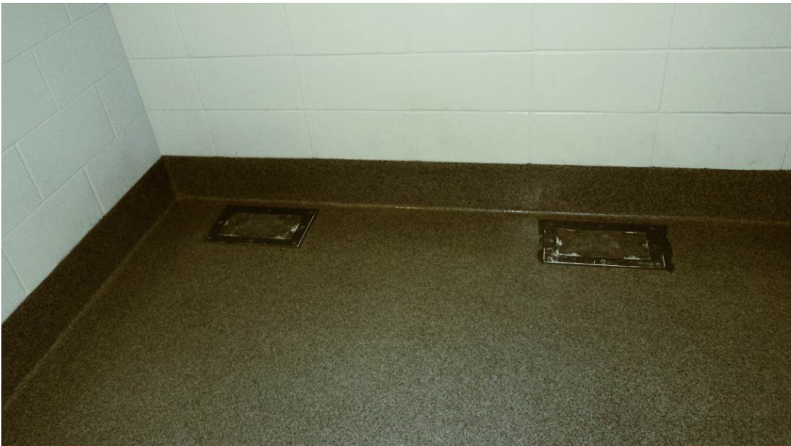
Photo 2 - Typical existing floor grills
