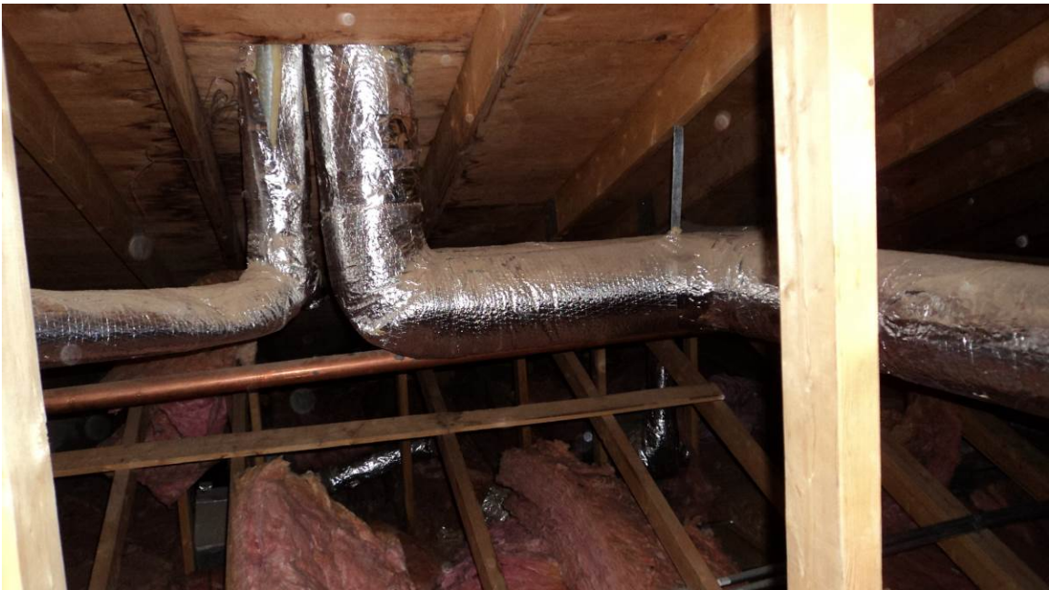
Photo 8 - Typical Exhaust Fan Attic Termination
