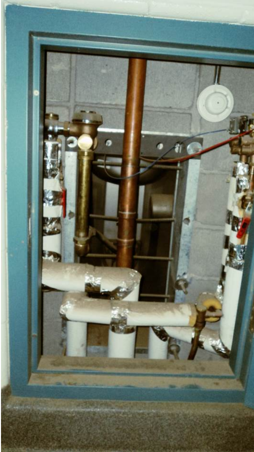
Photo 5 - Typical Detention Fixture Plumbing
