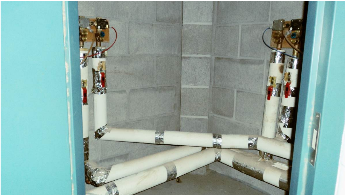
Photo 4 - Typical Detention Fixture Plumbing
