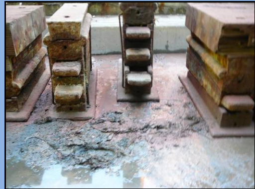
Sediment from the harbour often settles on dock bottom after dewatering. This may become contaminated with paint, etc. and must be disposed of.
