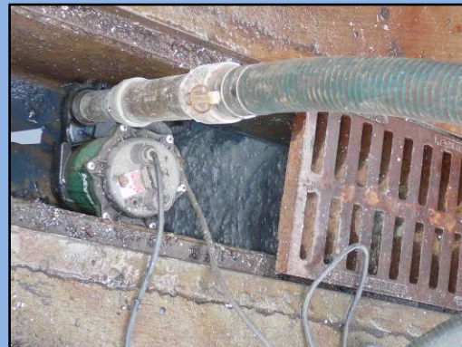
Example of a pump set up used to collect wash water on the NLW.
