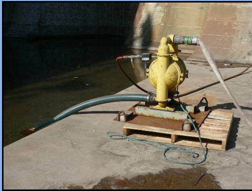
The sill diversion pump removes clean saltwater from the pool at the front of Section 1 (moon pool) and discharges to the tunnel drains through a hard pipe on the dock wall.
