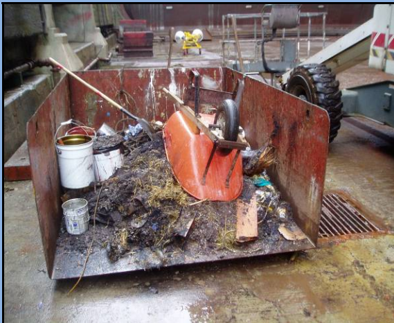
When cleaning dock bottom, skips of waste sandblast grit may leak contaminated water and should be removed as soon as possible.
