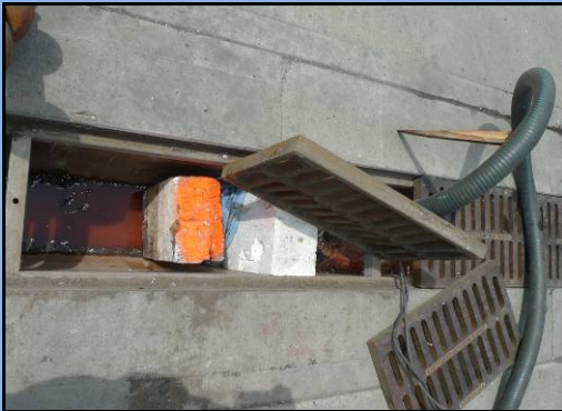
Example of styrofoam blocks used as a drain blocker on the NLW.
