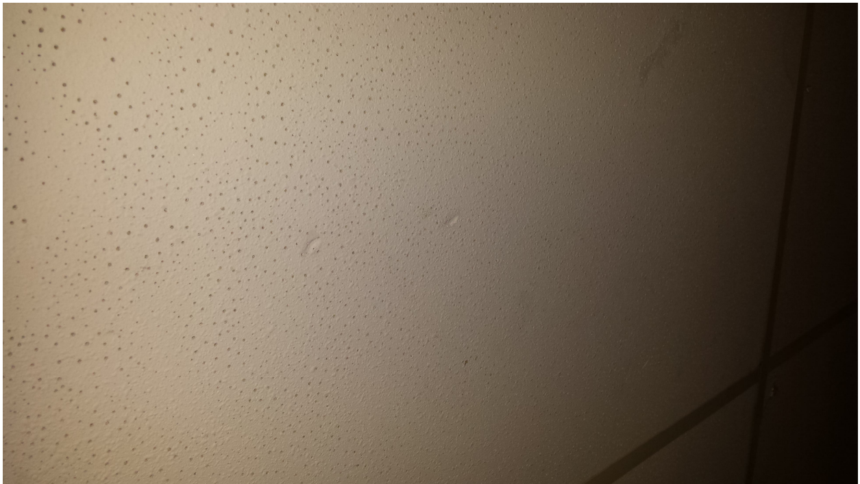
Photo 4 – Asbestos Containing Pink Back Acoustic Ceiling Tile
