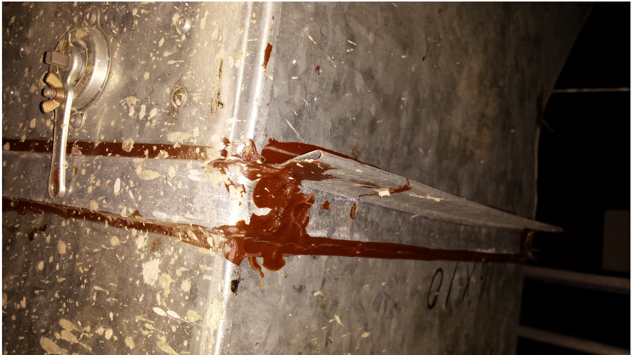
Photo 3 – Asbestos Containing Brown Duct Sealant
