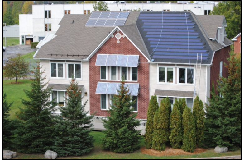
A roof-integrated photovoltaic system was installed on the InfoCentre of the CCHT. The InfoCentre also includes the FlexHouse.
