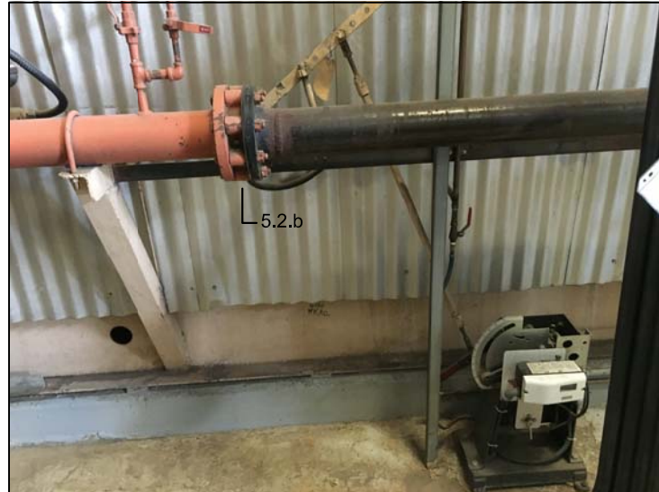
2 BOILER#3 CONTROL VALVE FOR REPLACEMENT M09 SPECIFICATION 23 00 00, ARTICLE 5.2.b
