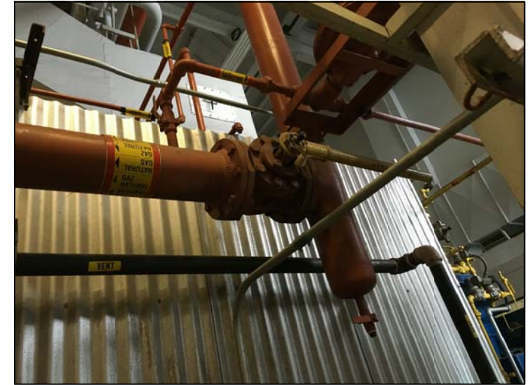
4 MOB BOILER#3 GAS SHUTOFF VALVE FOR REPLACEMENT SPECIFICATION 23 00 00, ARTICLE 3.2.d
