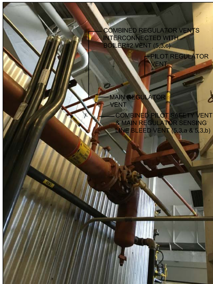
6 BOILER#3 PILOT REGULATOR & VENTS M09 SPECIFICATION 23 00 00, ARTICLE 5.3.a, 5.3.b & 5.3.c
