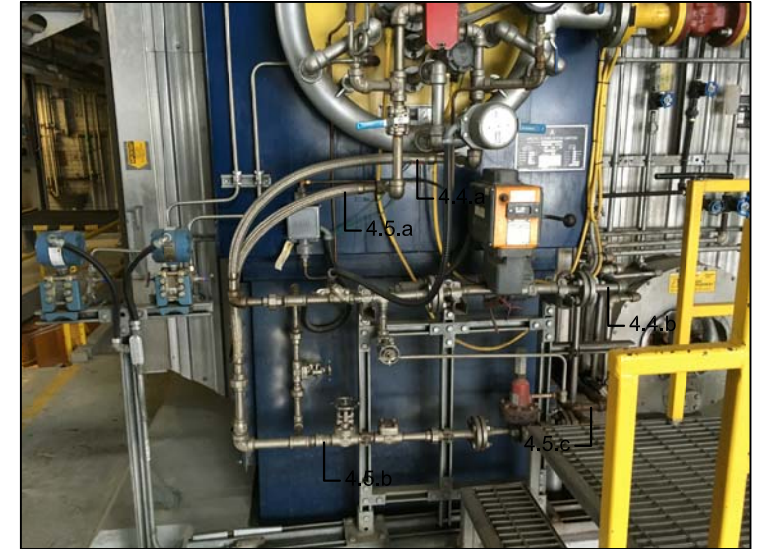
8 MOB BOILER#1 OIL & STEAM REPLACEMENTS & NEW WORK SPECIFICATION 23 00 00, ARTICLE 4.4.a, 4.4.b, 4.5.a, 4.5.b & 4.5.c
