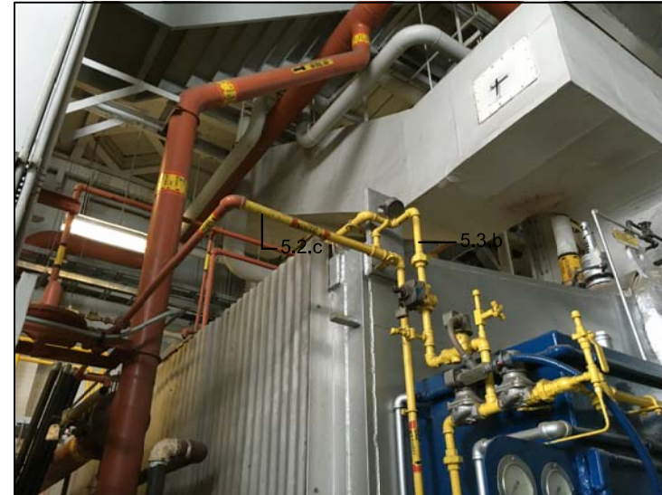
3 BOILER#3 PILOT REPLACEMENT & PILOT SAFETY VENT REMOVAL M09 SPECIFICATION 23 00 00, ARTICLE 5.2.c & 5.3.b
