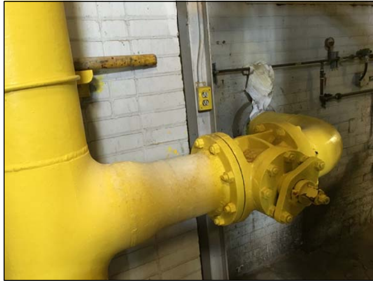
1 MOB MAIN 8" GAS SHUTOFF VALVE FOR REPLACEMENT SPECIFICATION 23 00 00, ARTICLE 3.2.g
