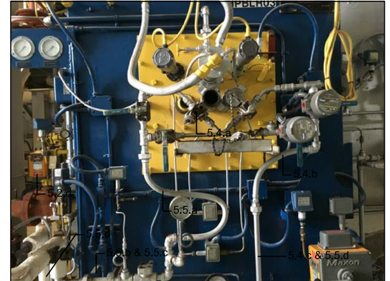
4 BOILER#3 OIL & STEAM REPLACEMENTS & NEW WORK M09 SPECIFICATION 23 00 00, ARTICLE 5.2.d, 5.4.a, 5.4.b, 5.4.c, 5.4.d & 5.5.a, 5.5.b, 5.5.c & 5.5.d
