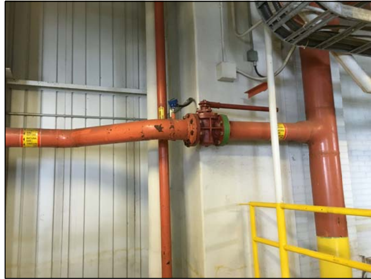
2 MOB BOILER#4 GAS SHUTOFF VALVE FOR REPLACEMENT SPECIFICATION 23 00 00, ARTICLE 3.2.b
