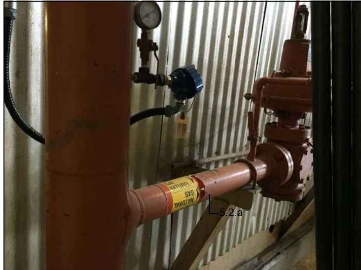
1 BOILER#3 GAS STRAINER LOCATION M09 SPECIFICATION 23 00 00, ARTICLE 5.2.a
