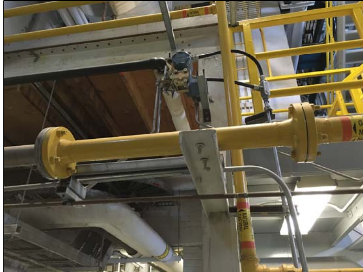
5 MOB BOILER#1 GAS STRAINER LOCATION SPECIFICATION 23 00 00, ARTICLE 4.2.a
