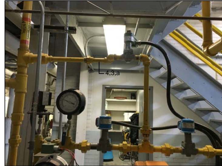
7 MOB BOILER#1 GAS PILOT SAFETY VALVE REMOVAL SPECIFICATION 23 00 00, ARTICLE 4.3.a
