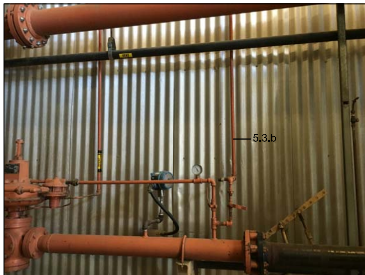
5 BOILER#3 MAIN REGULATOR & VENTS M09 SPECIFICATION 23 00 00, ARTICLE 5.3.b
