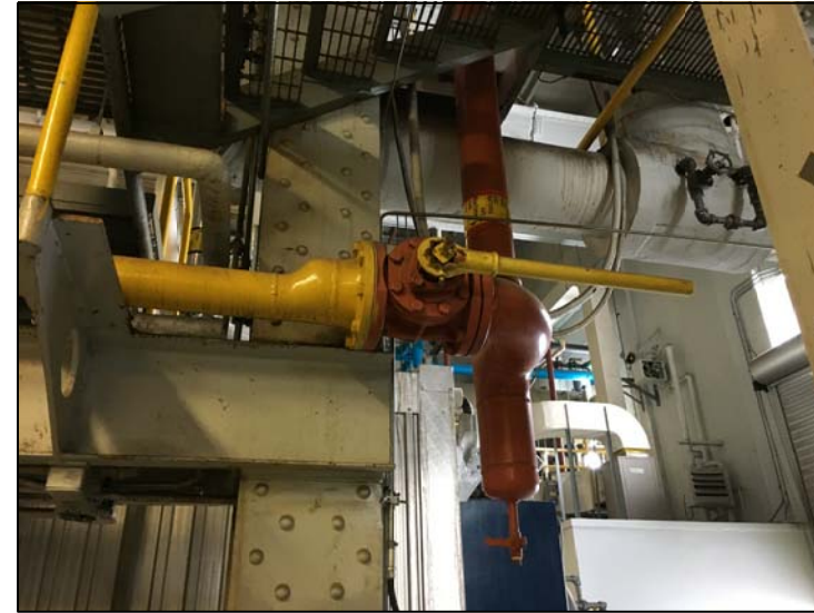
3 MOB BOILER#2 GAS SHUTOFF VALVE FOR REPLACEMENT SPECIFICATION 23 00 00, ARTICLE 3.2.c
