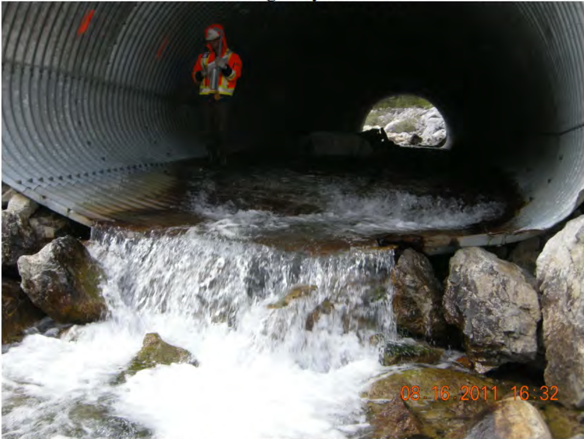
P11 - South Barrel - Outlet - Floor has Drooped Down ~400 mm in Both Barrels Due to Erosion of Supporting Material Below Outlet in Past
