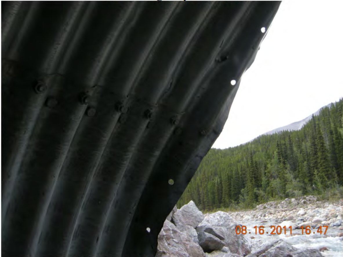
P13 - North Barrel - Minor Collision Damage to Inlet Rim
