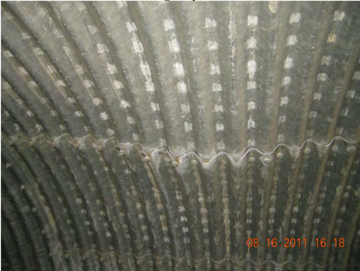
P09 - South Barrel - Ring 5 - Roof Kinked Down ~150 mm
