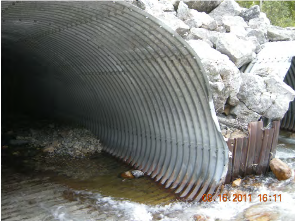
P05 - South Barrel - Minor Collision Damage both Sides of Inlet Rim
