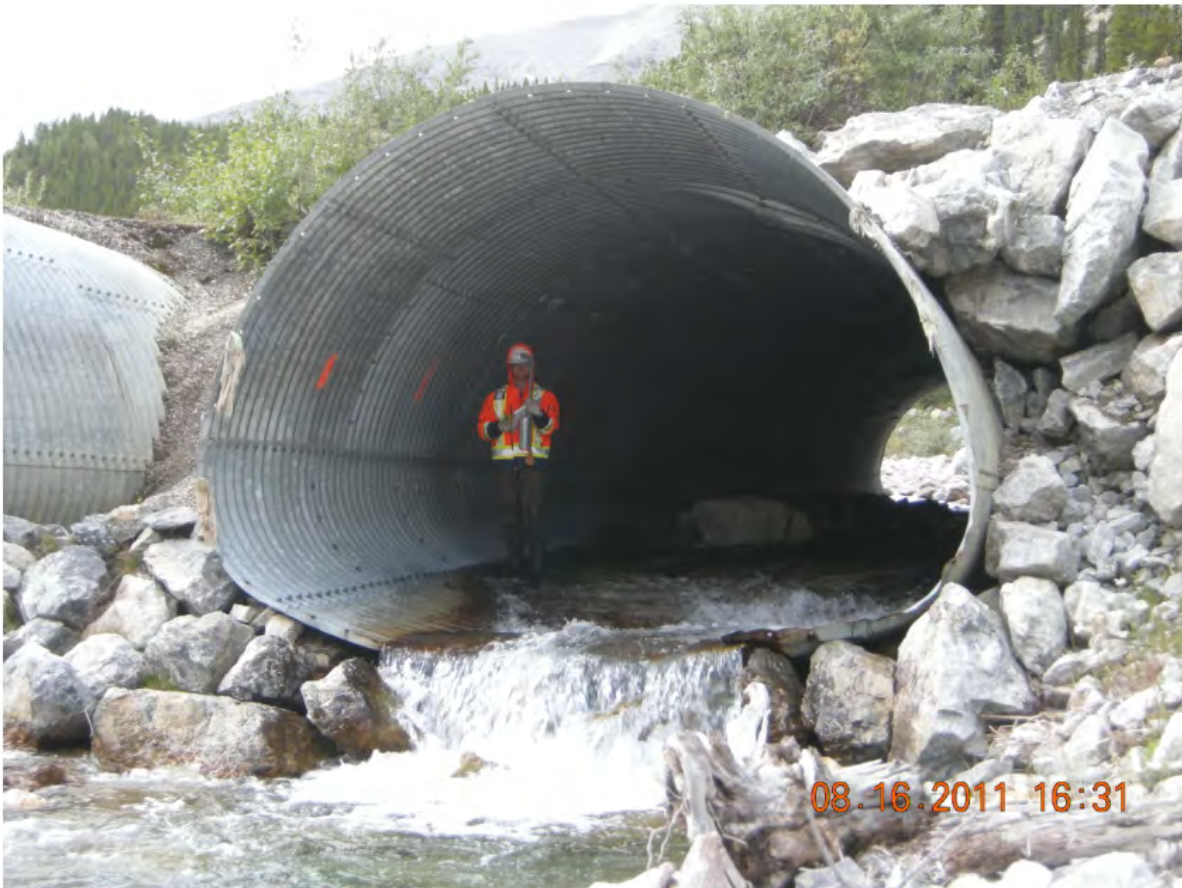
P10 - South Barrel - Floor has Drooped Down ~400 mm in Both Barrels - Collision Damage Kink in Roof at Ring 14
