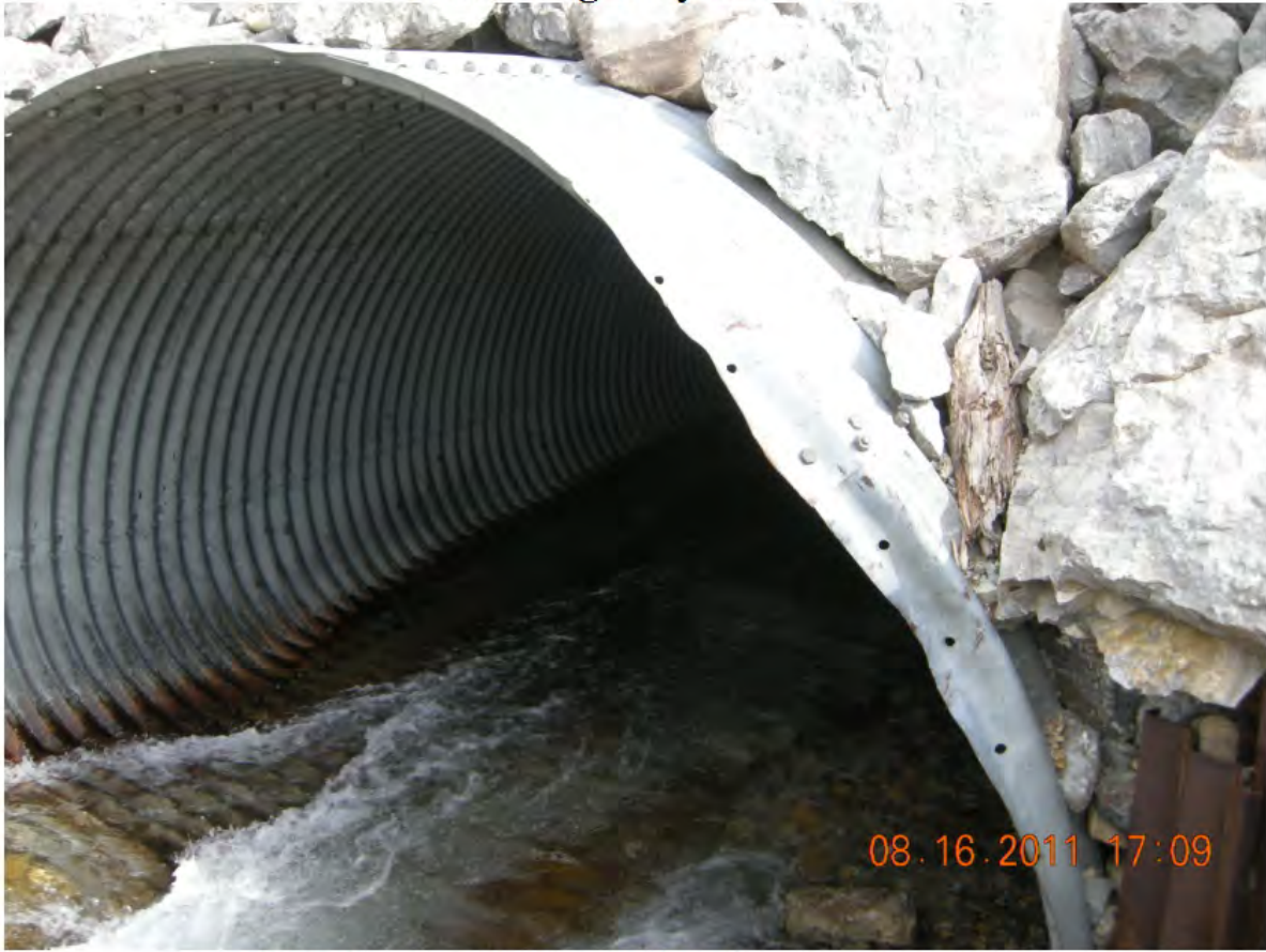
P19 - North Barrel - Minor Collision Damage to Outlet Rim
