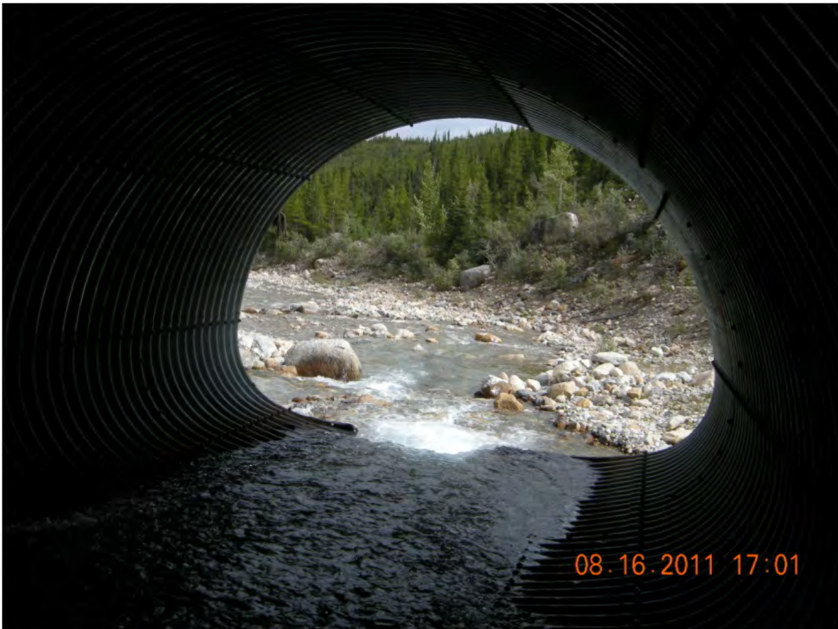
P16 - North Barrel - Floor has Dropped Down ~400 mm in Both Barrels
