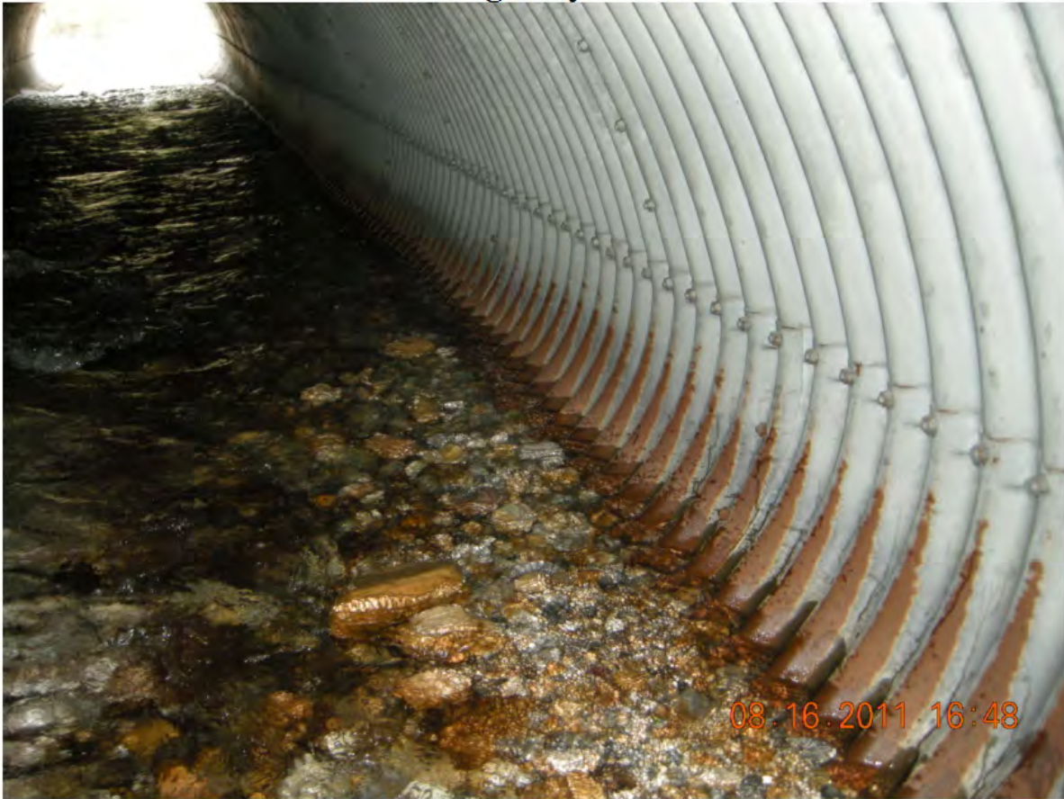
P15 - North Barrel - Light Surface Corrosion to High Water Level
