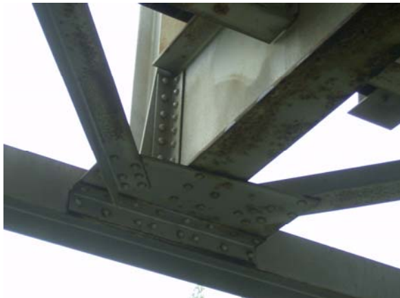
Figure 10: Floor Beam to Vertical Truss Member Connection and Diagonal Bracing to Floor Beam Connection.
