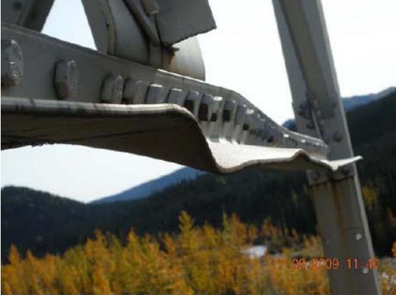
Figure 18: Example of Typical Vehicle Collision Damage to Truss Lateral Bracing.
