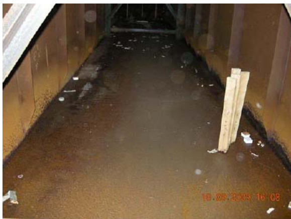
Figure 13: Water-Pooling Inside of West Box Girder.
