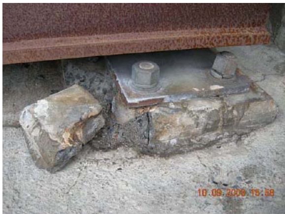
Figure 14: Typical Spalling of Bearing Seats.
