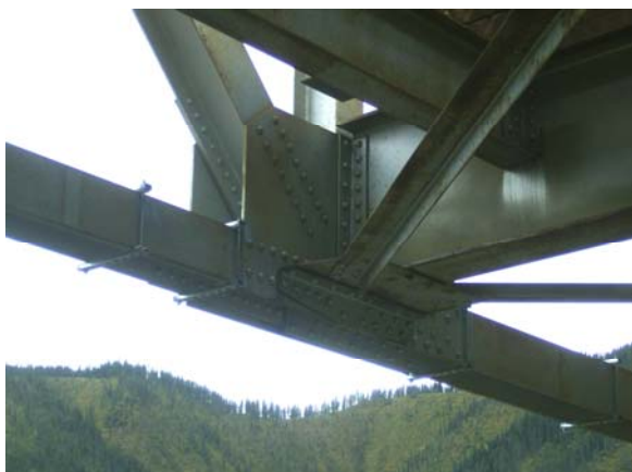
Figure 11: Diagonal Truss Member to Vertical Truss Member and Bottom Chord Truss Member Connection.
