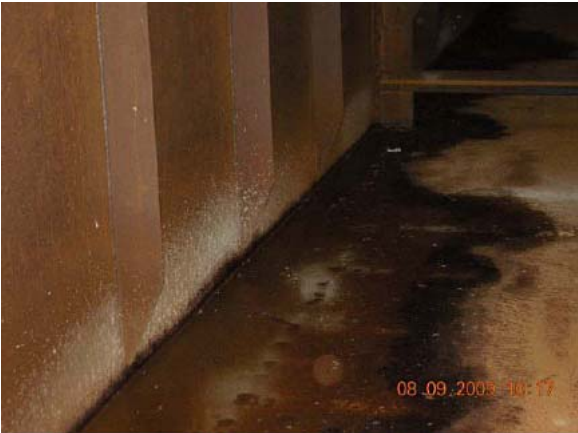
Figure 11: Water-Pooling Inside of Both Box Girders.
