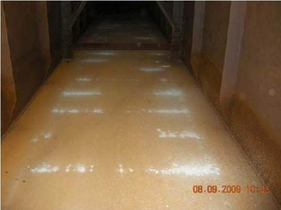
Figure 12: Efflorescence Staining Inside of Both Box Girders.
