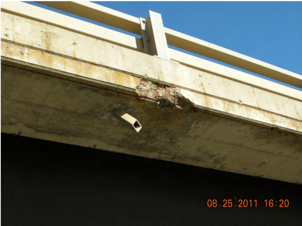
P32 - Span 3 - Spall in West Cantilever Facia ~60 mm Deep with Exposed Rebar at Midspan
