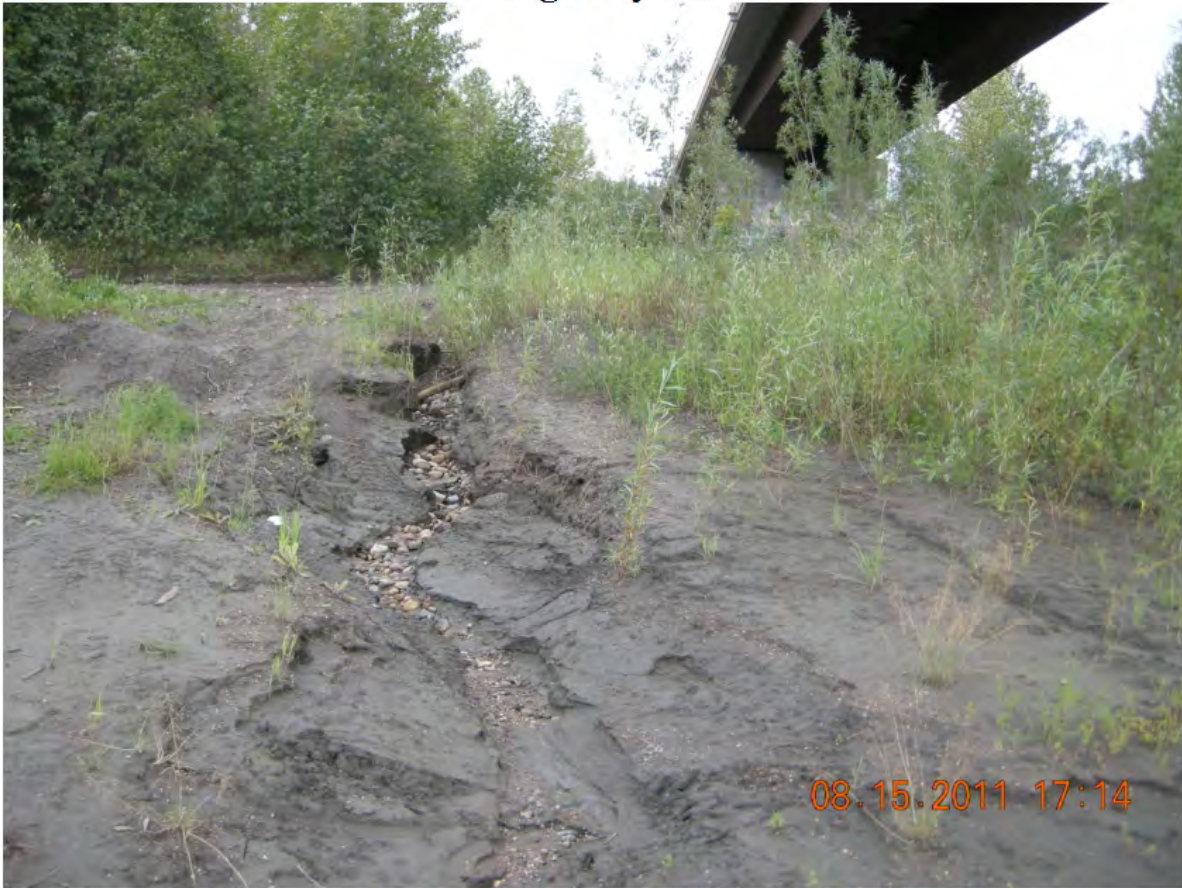
P65 - South Embankment - Erosion Gully up to 400 mm Deep
