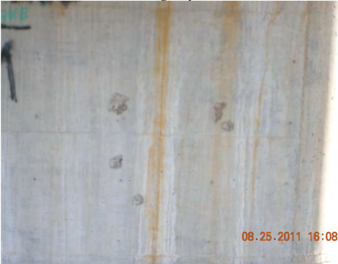
P71 - Pier 3 - North Face - Rifle Shot Spalls
