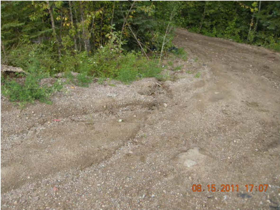
P23 - SE Corner Embankment - Minor Erosion Gullies - 100 mm Deep
