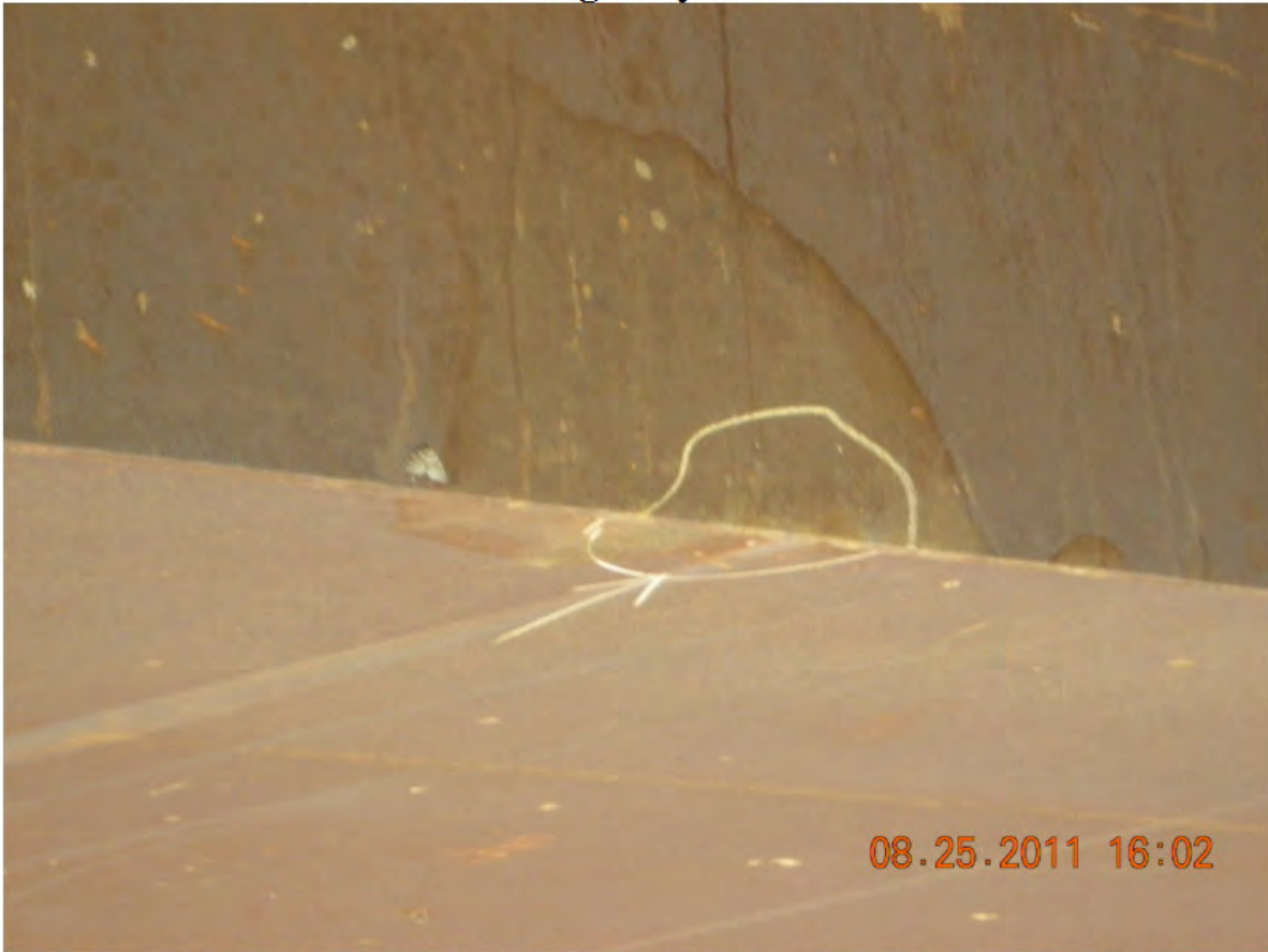
P37 - Span 4 - East Girder - Notch in West Side of Bottom Flange - From Overheight Vehicle
