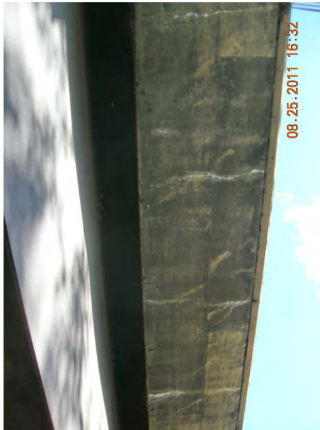
P28 - Span 2 - Narrow Transverse Cracks in Cantilevers - Typical - No Sign of Recent Moisture Staining
