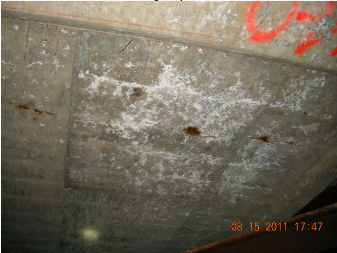
P43 - East Girder - Span 3 Soffit - Random Rust Staining - No Recent Moisture Staining
