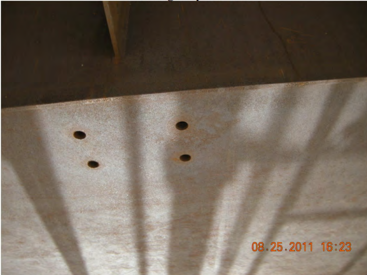
P39 - Box Girder Bottom Flanges - Typical - Obsolete Bolt Holes Likely Used for Shipping or Erection
