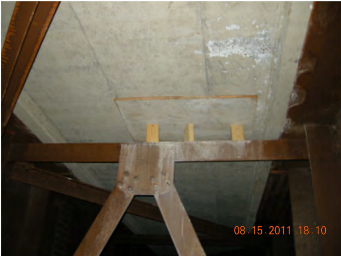
P54 - West Girder - Span 3 - Patch in Soffit with Formwork Still in Place
