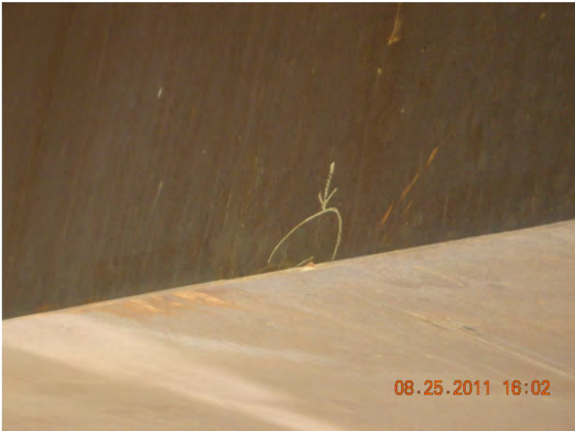
P36 - Span 4 - West Girder - Notch in East Side of Bottom Flange - From Overheight Vehicle
