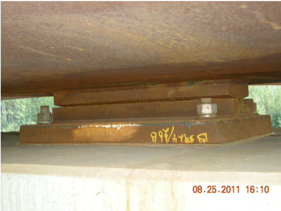
P72 - Pier 3 - West Girder - East Fixed Bearing - Fixed Bearings on Pier 3 Only
