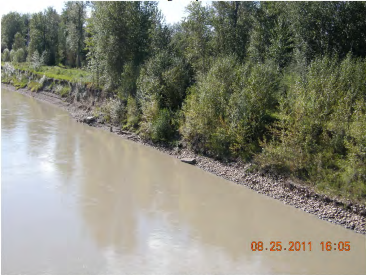
P07 - Erosion Upstream on the NW River Embankment
