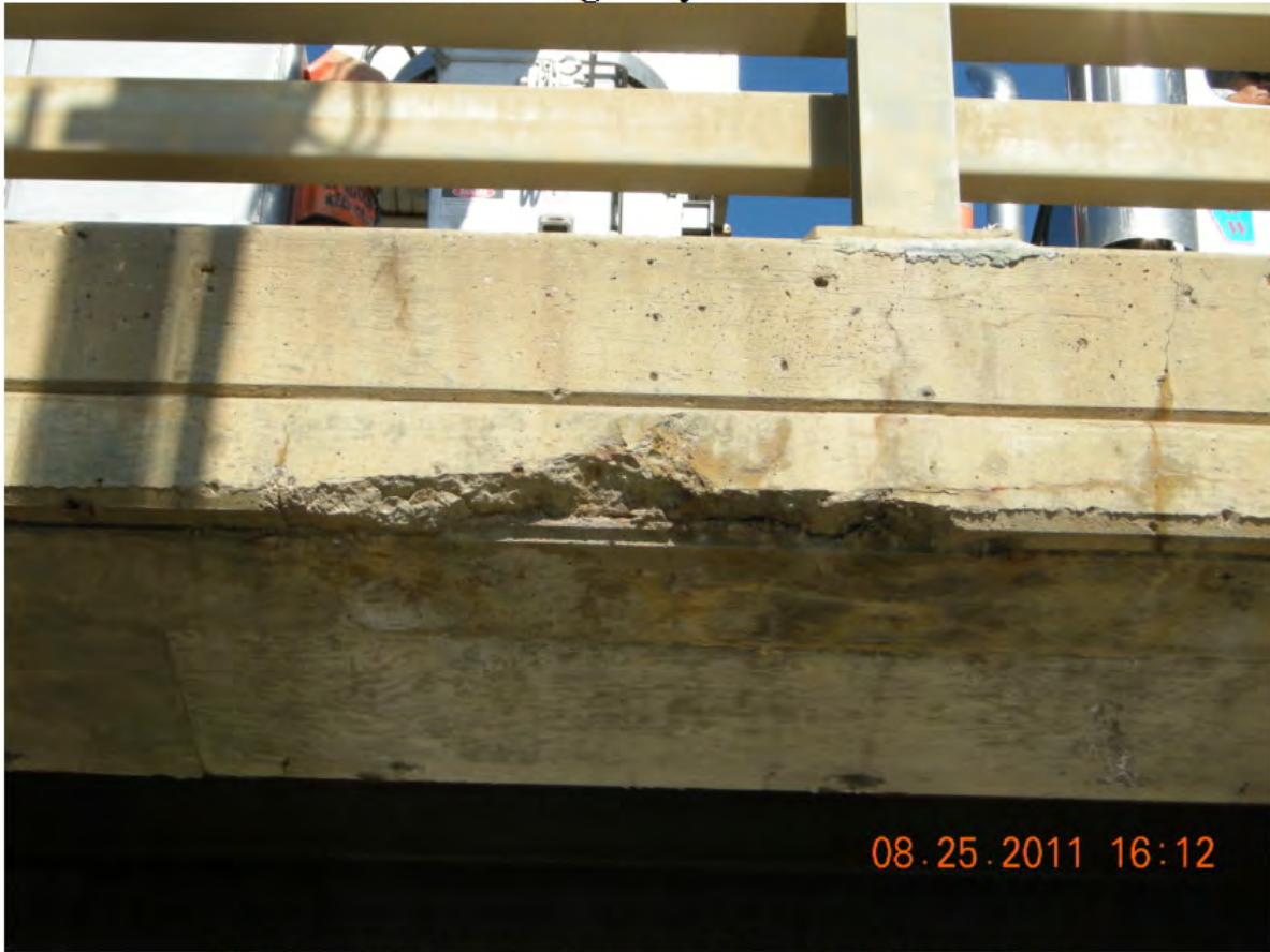
P33 - Span 3 - Spall in West Cantilever Fascia ~40 mm Deep at Pier 3
