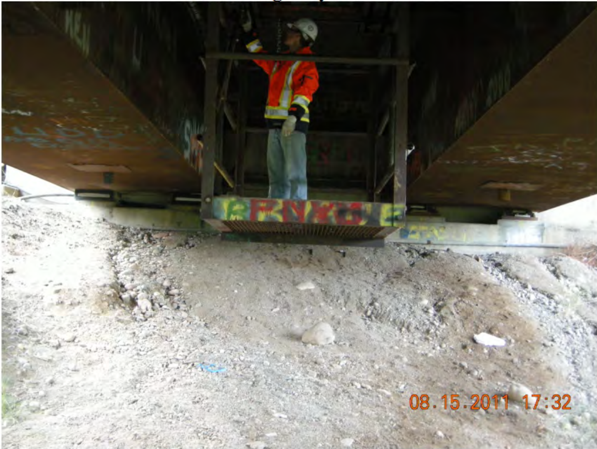
P77 - North Abutment - Inspection Platform Locked Out
