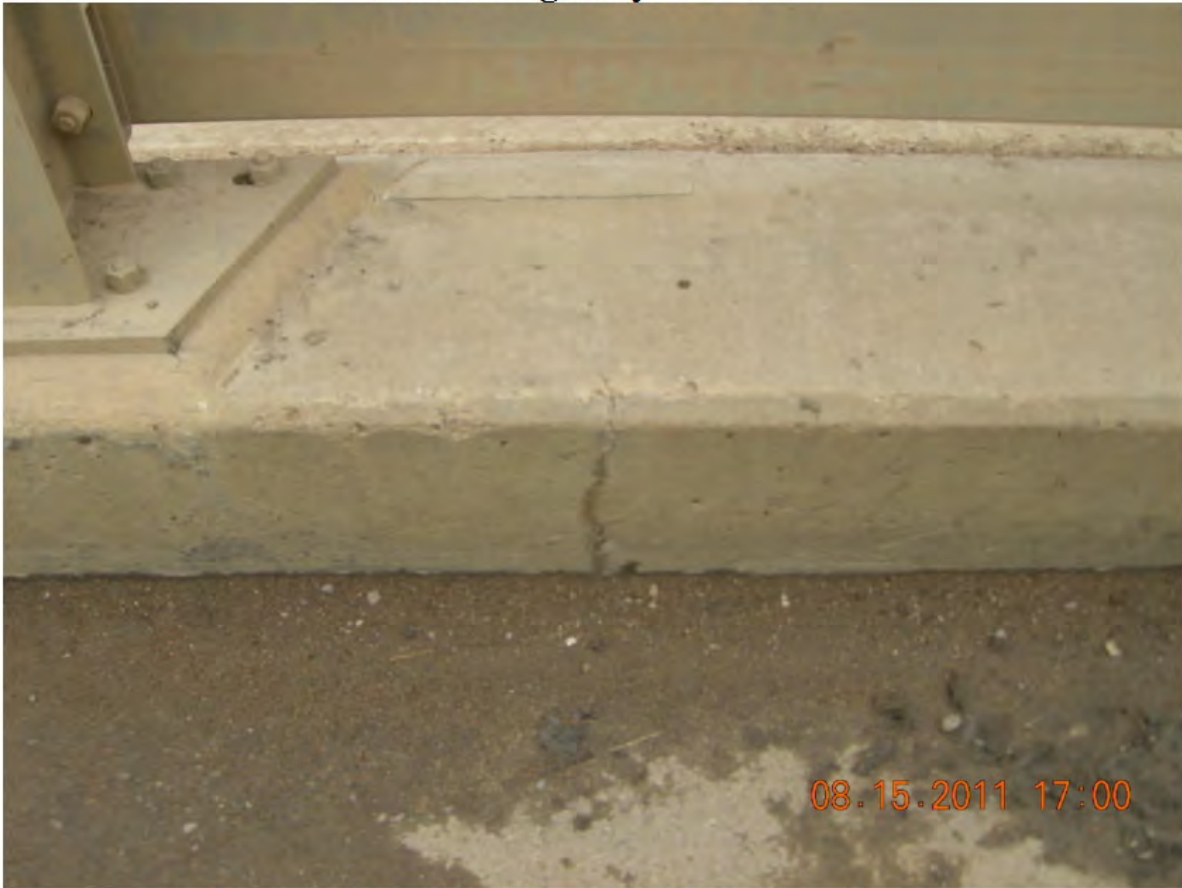
P21 - East Curb - Random Narrow Shrinkage Cracks Throughout
