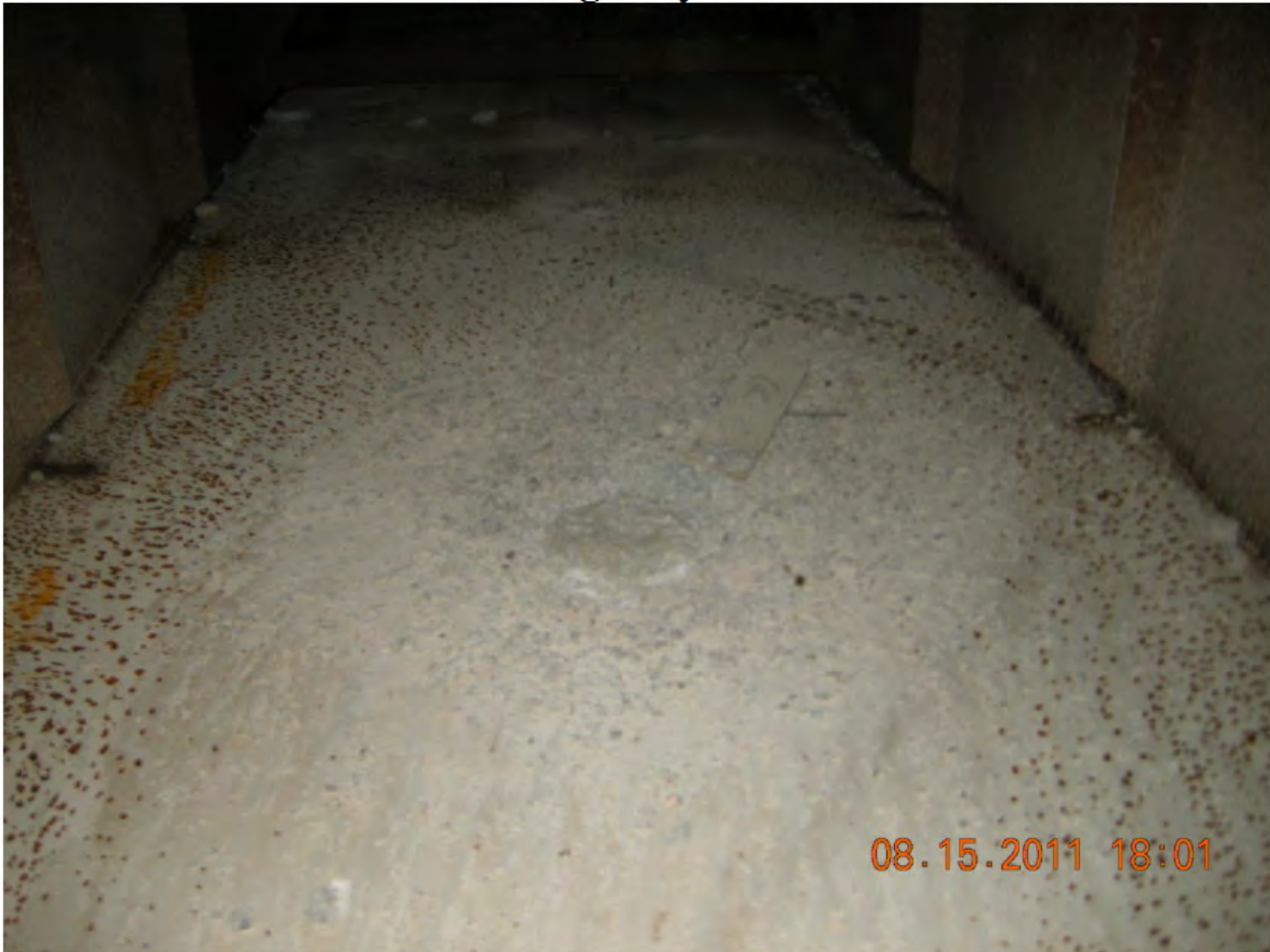
P45 - East Girder - Span 4 - Concrete on Bottom Flange below Deck Patch from Deck Repairs
