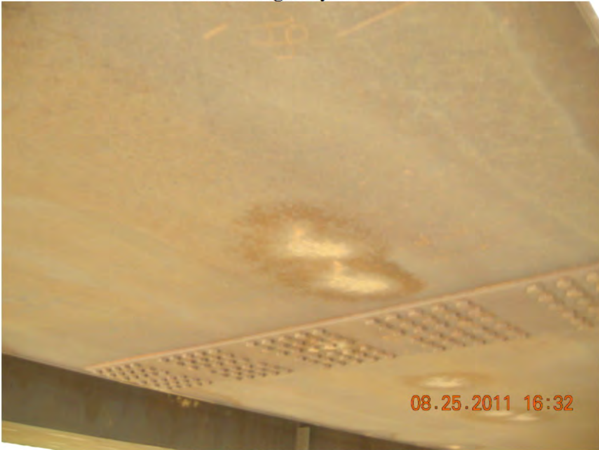
P27 - Span 2 - Paint Ball Marks on Both Girders
