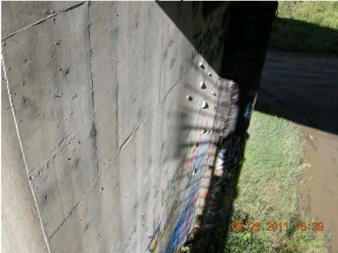
P63 - Pier 1 - South Face - Stones Epoxied to South Face Likely for Climbing
