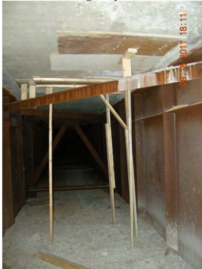
P53 - West Girder - Span 3 - 3 Soffit Patches near Midspan - Formwork Left in Place - Leaked Concrete on Bottom Flange
