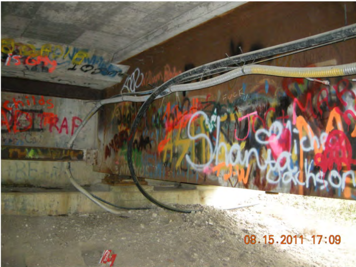
P60 - Several Utility Conduits Attached to the Inside Web of the West Girder
