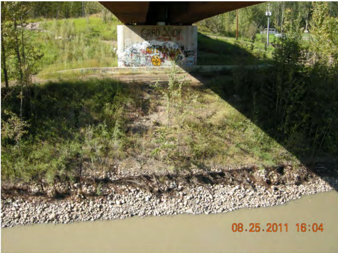
P08 - North Embankment and Pier 4 - Erosion along Embankment
