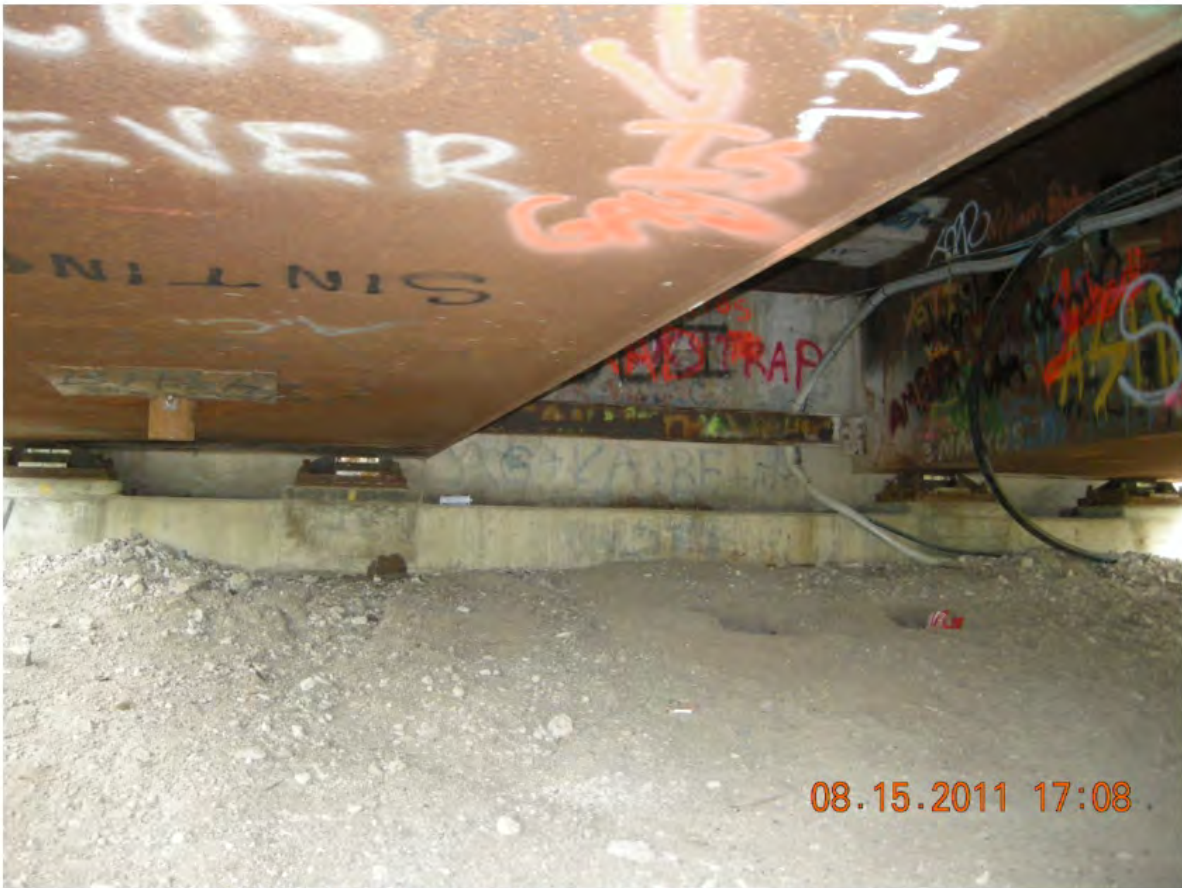
P58 - South Abutment - Cladding Missing on All Bearings
