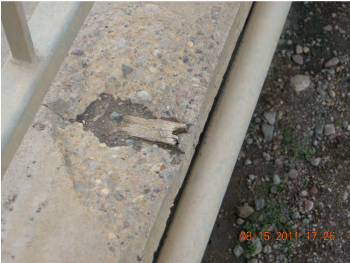
P18 - Span 5 - East Curb Spalled ~60 mm Deep with Timber Formwork Embedded
