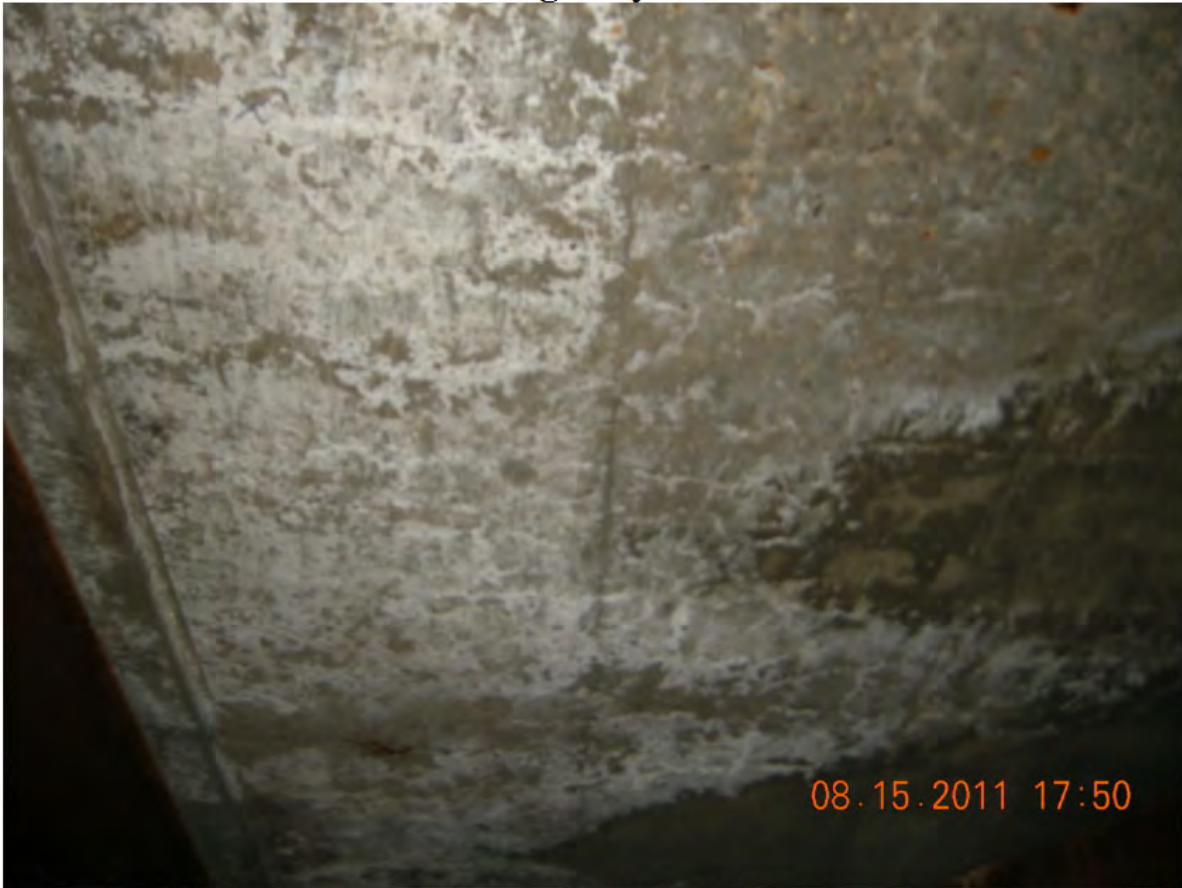
P41 - East Girder - Span 2 Soffit - Leaching Hairline Map Cracks - Typical - No Sign of Recent Seepage - No Delamination
