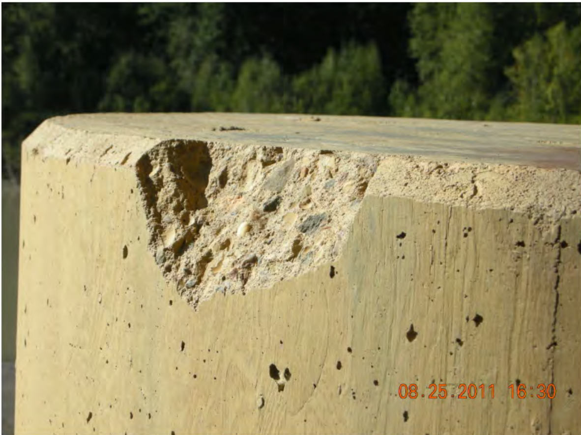
P66 - Pier 2 Bearing Seat - Minor Spall 30 mm Deep at West End
