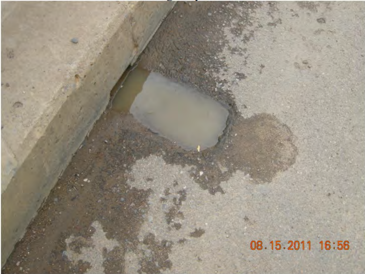
P19 - Some Deck Drains Plugged
