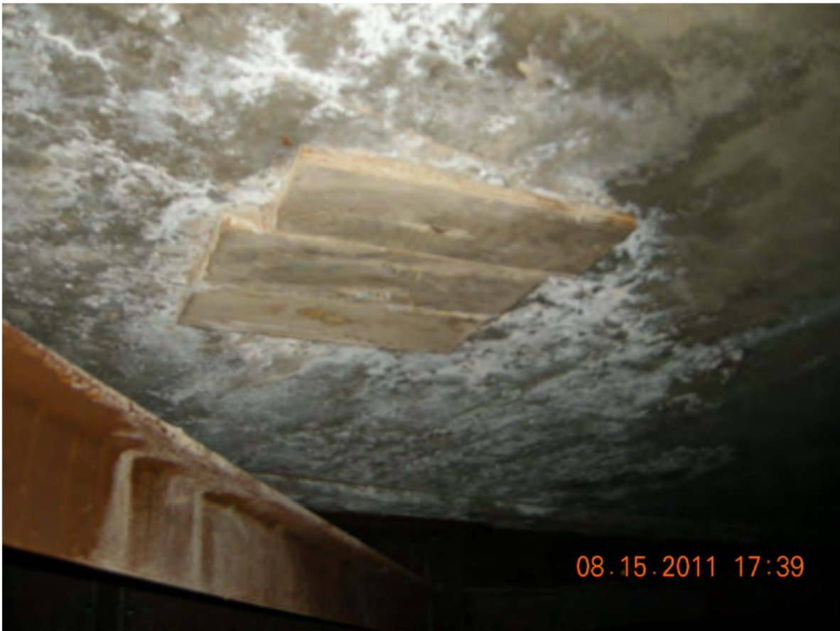
P48 - East Girder - Span 5 - Soffit Patch at Midspan - Formwork Left In - Leaching Narrow Map Cracks - No Delaminations
