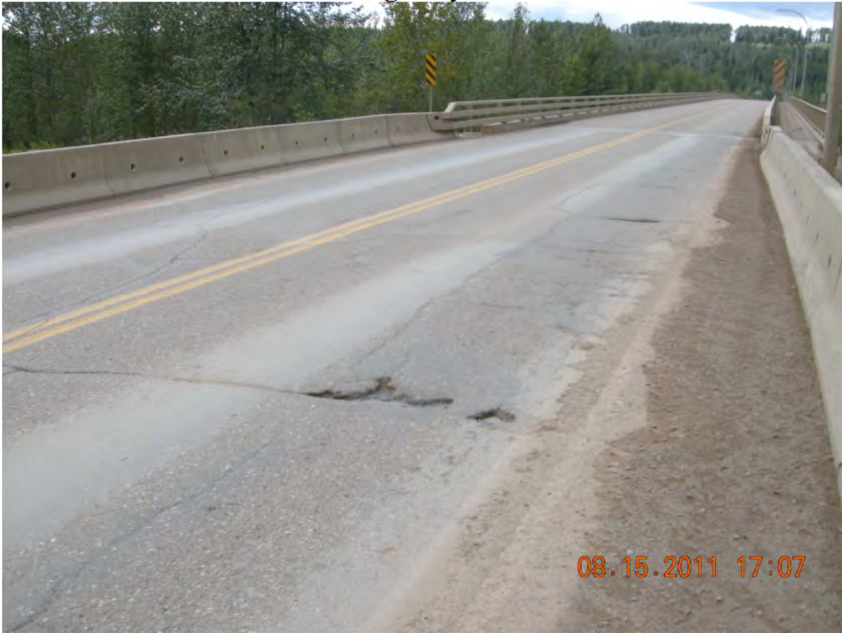
P15 - South Approach - Wide Transverse Cracks and Pot Holes in Asphalt
