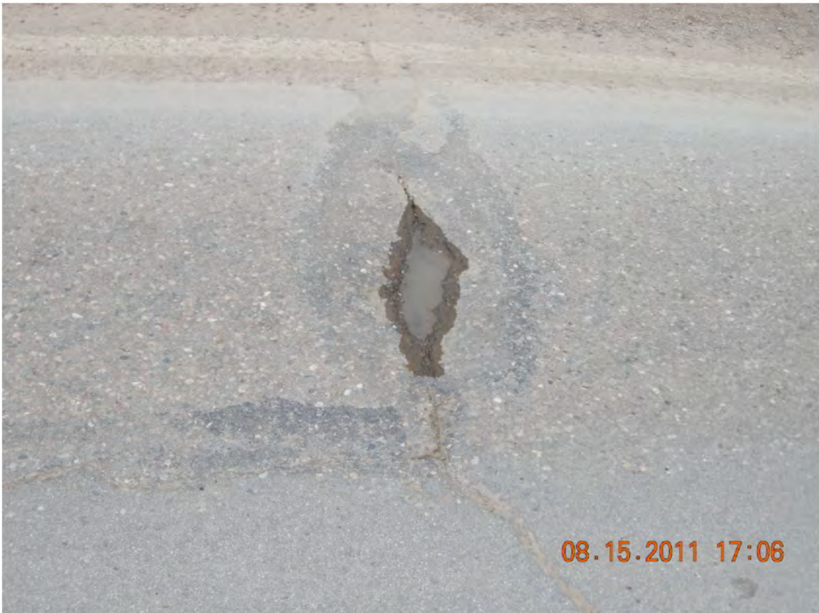
P16 - South Approach - Wide Transverse Cracks and Pot Holes in Asphalt
