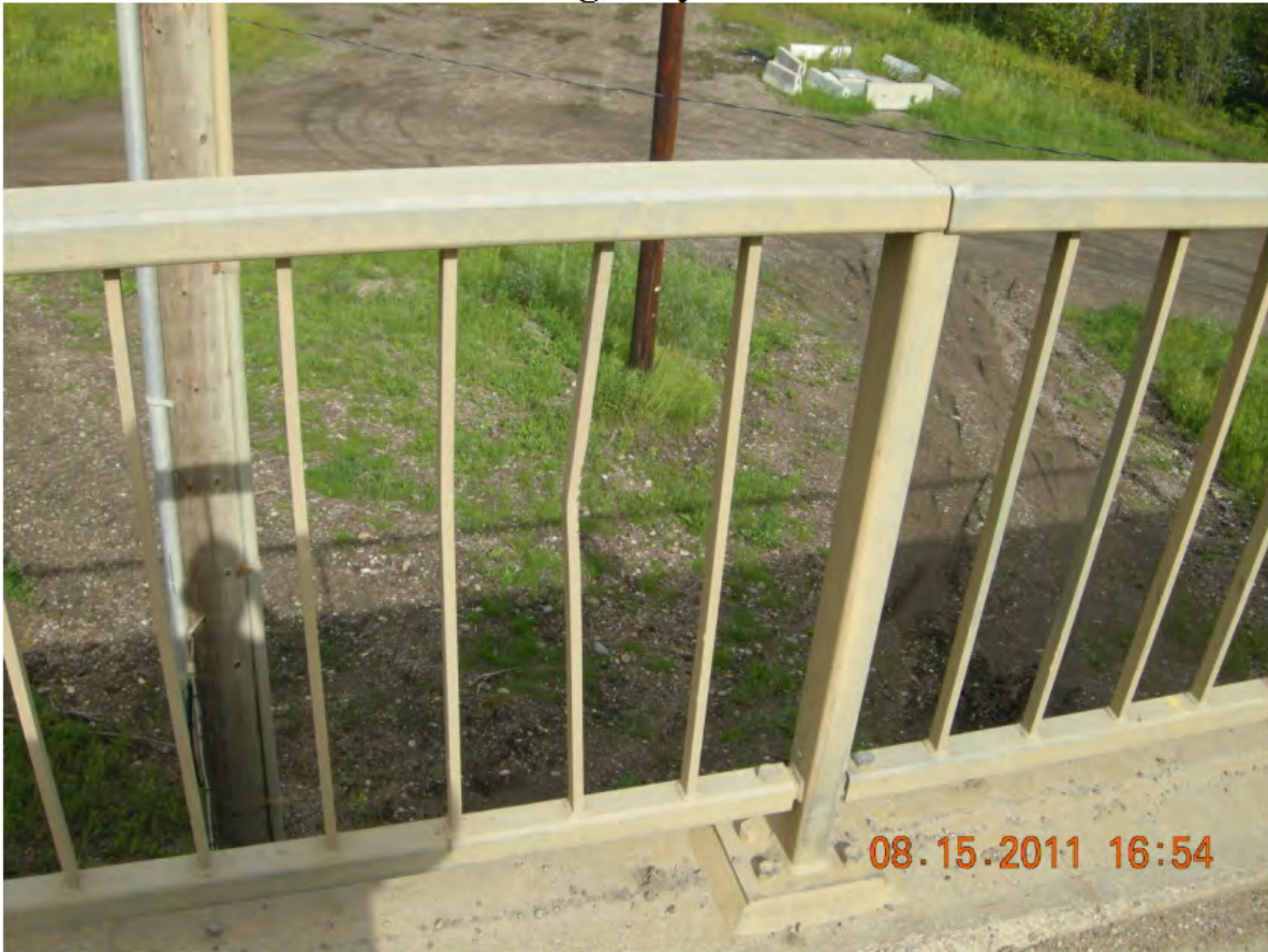
P17 - Galvanized Steel Pedestrian Railing on East Side - Minor Collision Damage in Several Locations
