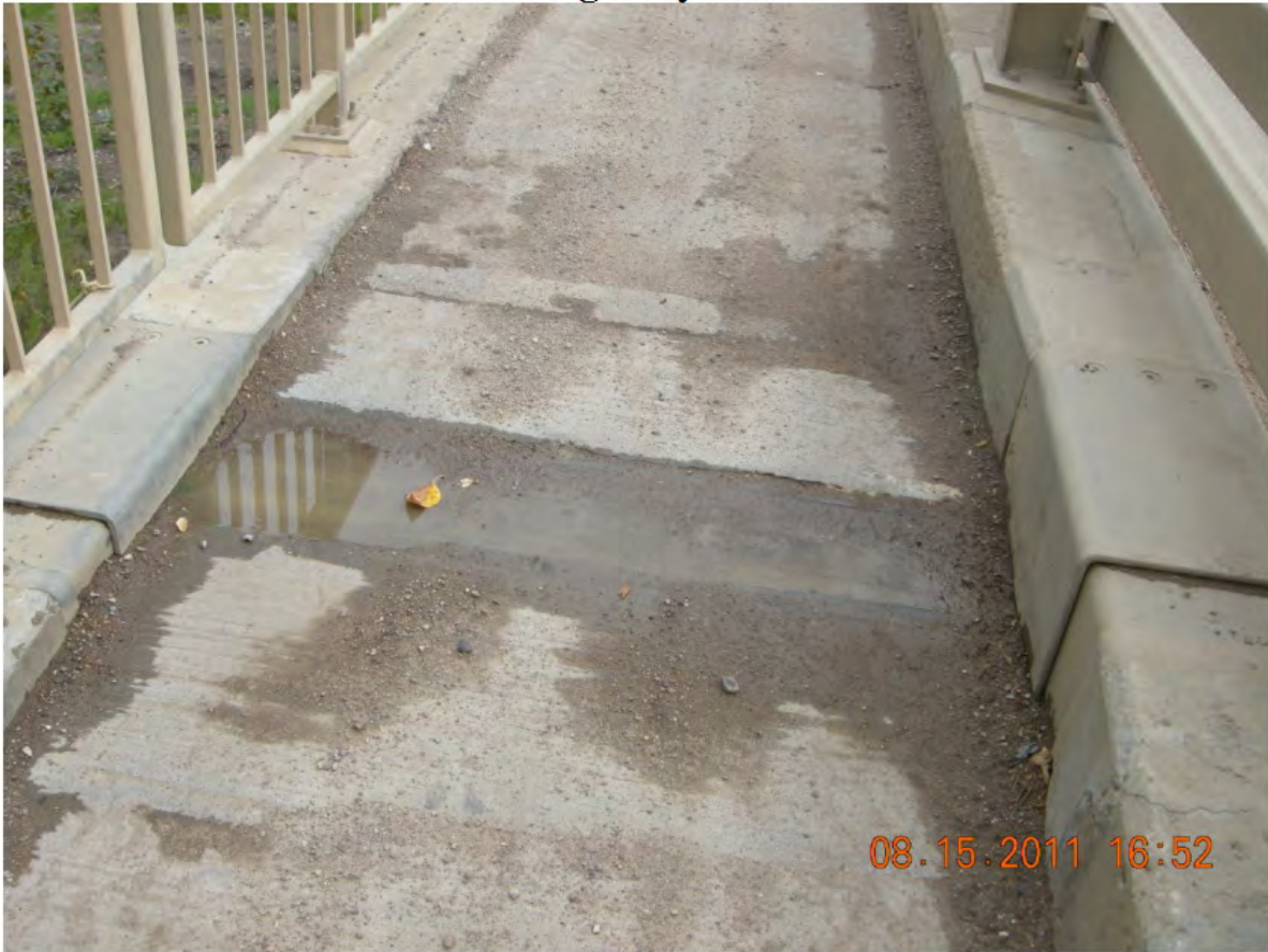
P11 - Water Ponding in NE Sidewalk Deck Joint
