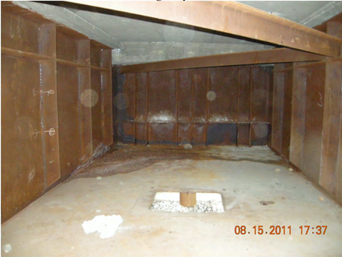
P49 - East Girder - Span 5 - North End - Moisture Staining in Bottom Flange
