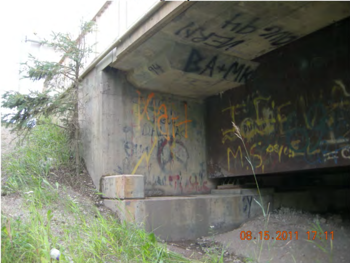
P57 - South Abutment and SE Wingwall - Utility Conduit Running Along East Curb
