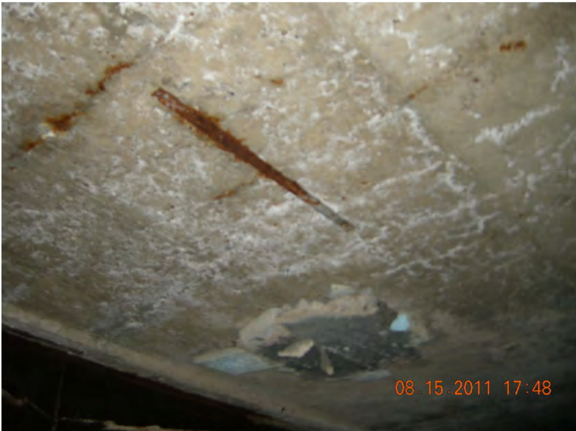
P42 - East Girder - Span 3 - Soffit Patch and Rust Staining Near Midspan - Formwork Left in - No Delaminations
