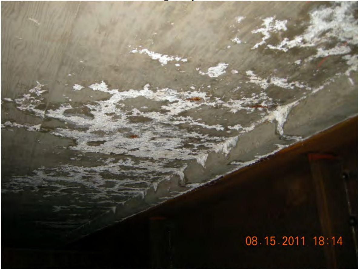
P51 - West Girder - Span 2 Soffit - Leaching Hairline Map Cracks - No Signs of Recent Moisture Staining - No Delaminations
