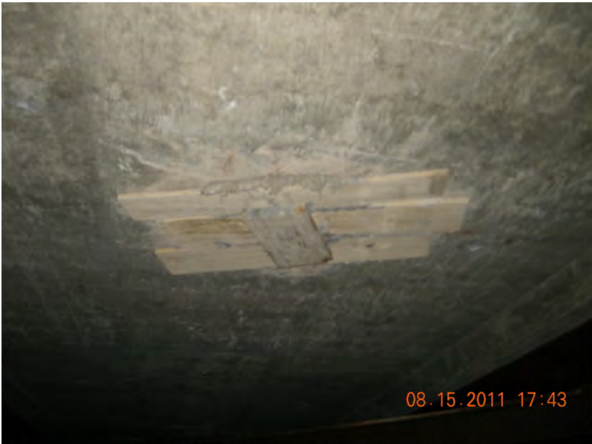
P44 - East Girder - Span 4 - Soffit Patch - Formwork Left In
