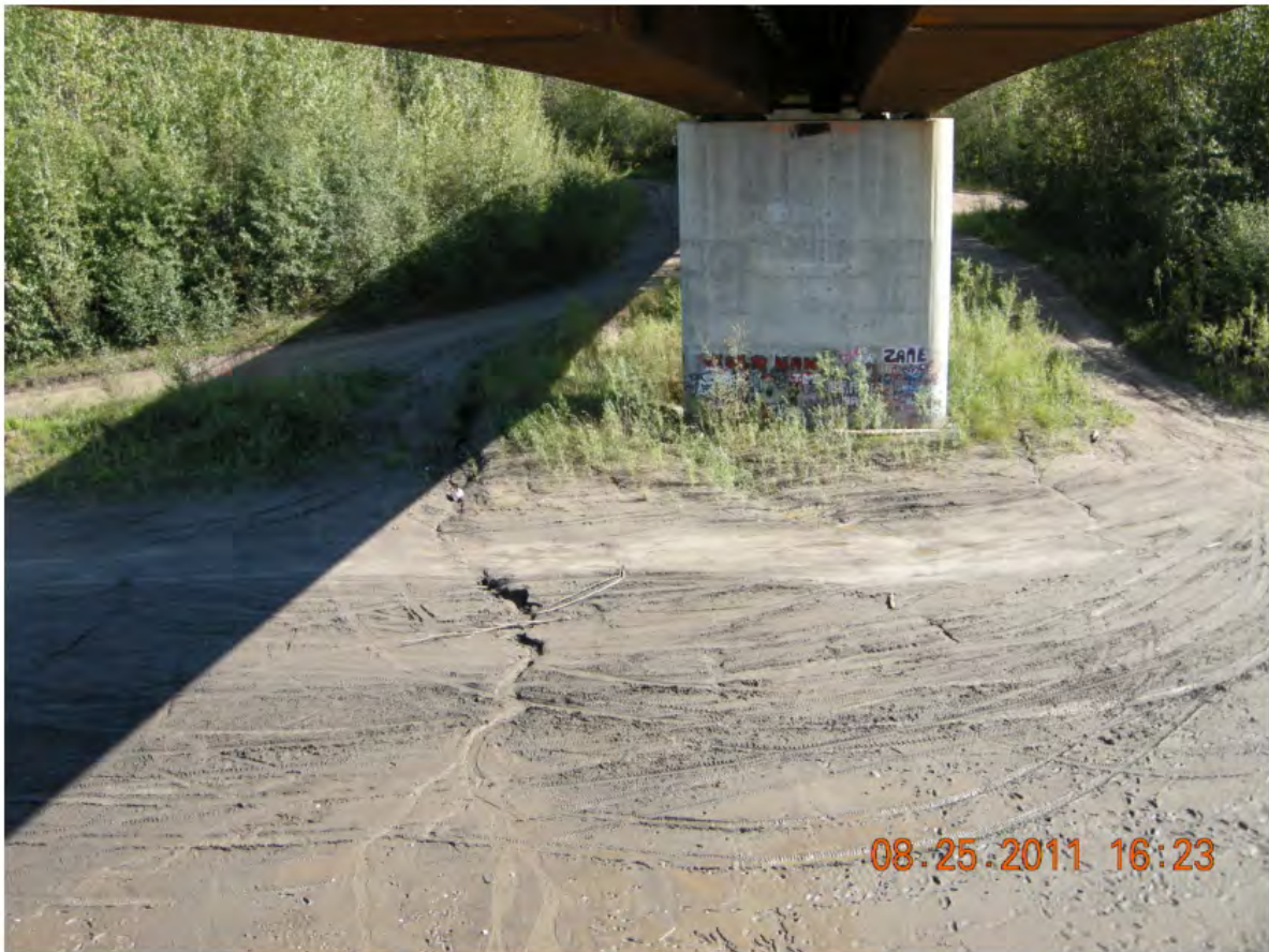
P64 - Pier 2 - North Face - Erosion Gully in South Embankment
