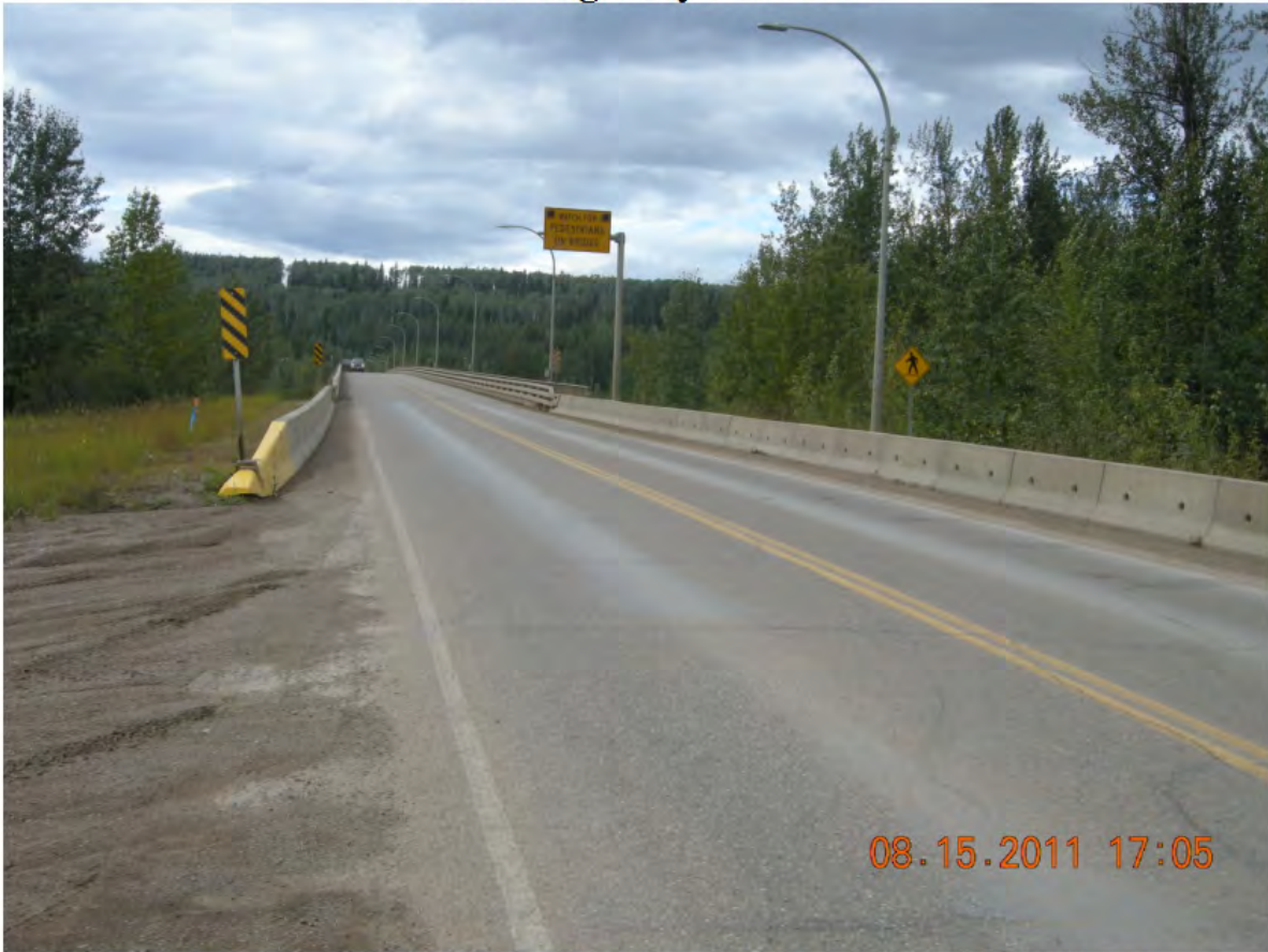
P01 - South Approach - Looking North - 3 Delineators in Place but River Name Sign Missing
