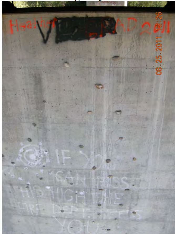
P67 - Pier 2 - North Face - Stones Epoxied to Pier Face Likely for Climbing
