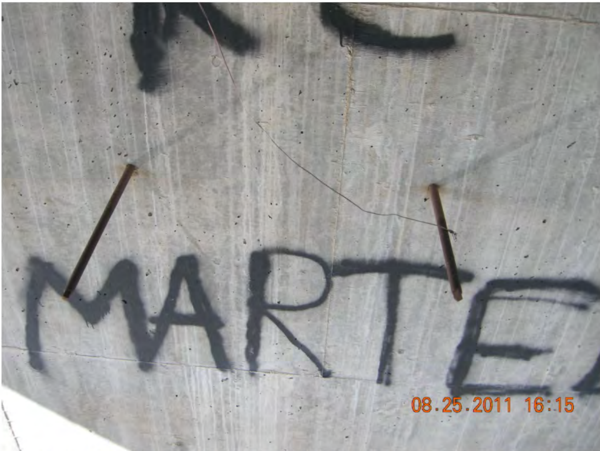
P70 - Pier 3 - South Face - 2 Pieces of Rebar Sticking out of South Face near Bearing Seat
