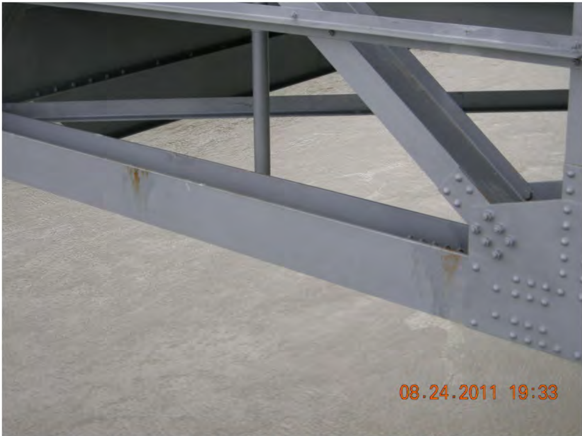
P40 - Span 2 - Bottom East Chord at L9-L10 - Localized Light Surface Corrosion
