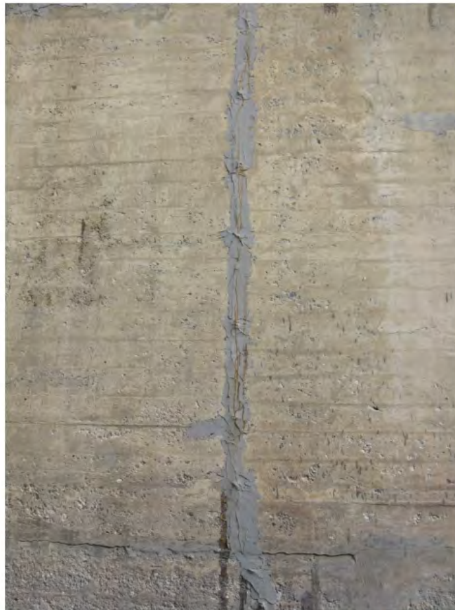
UW10 - Pier 1 Typical crack repair with grout - Pier 1 LC face
