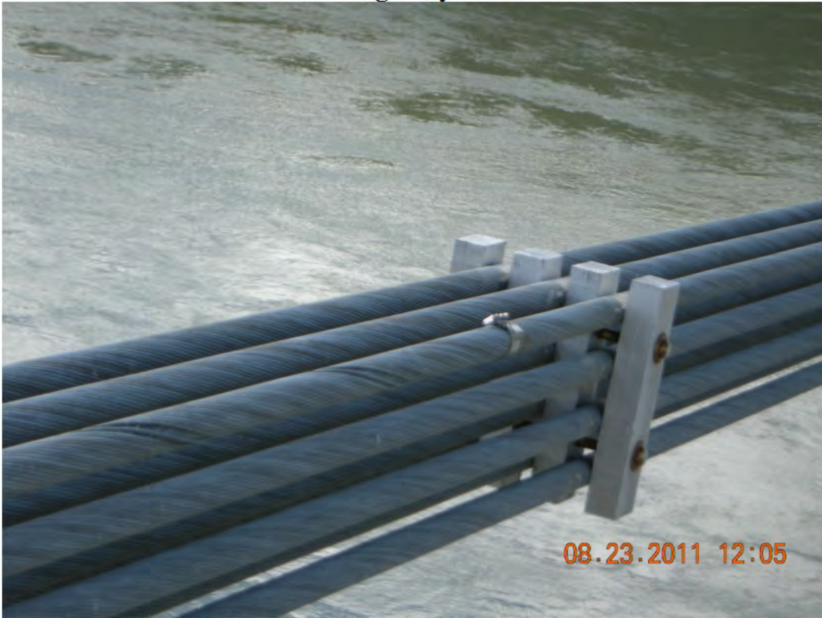
P81 - Span 2 - East Cables 22N to 20N - Three #10 Broken Wires Clamped
