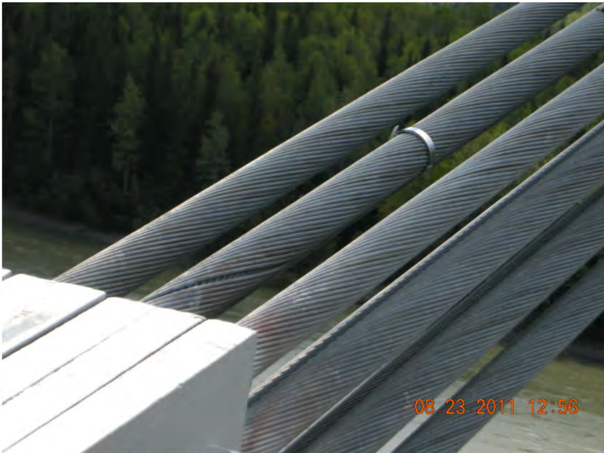
P88 - Span 3 - East Cables 10N to 8N - One #11 Broken Wires Clamped
