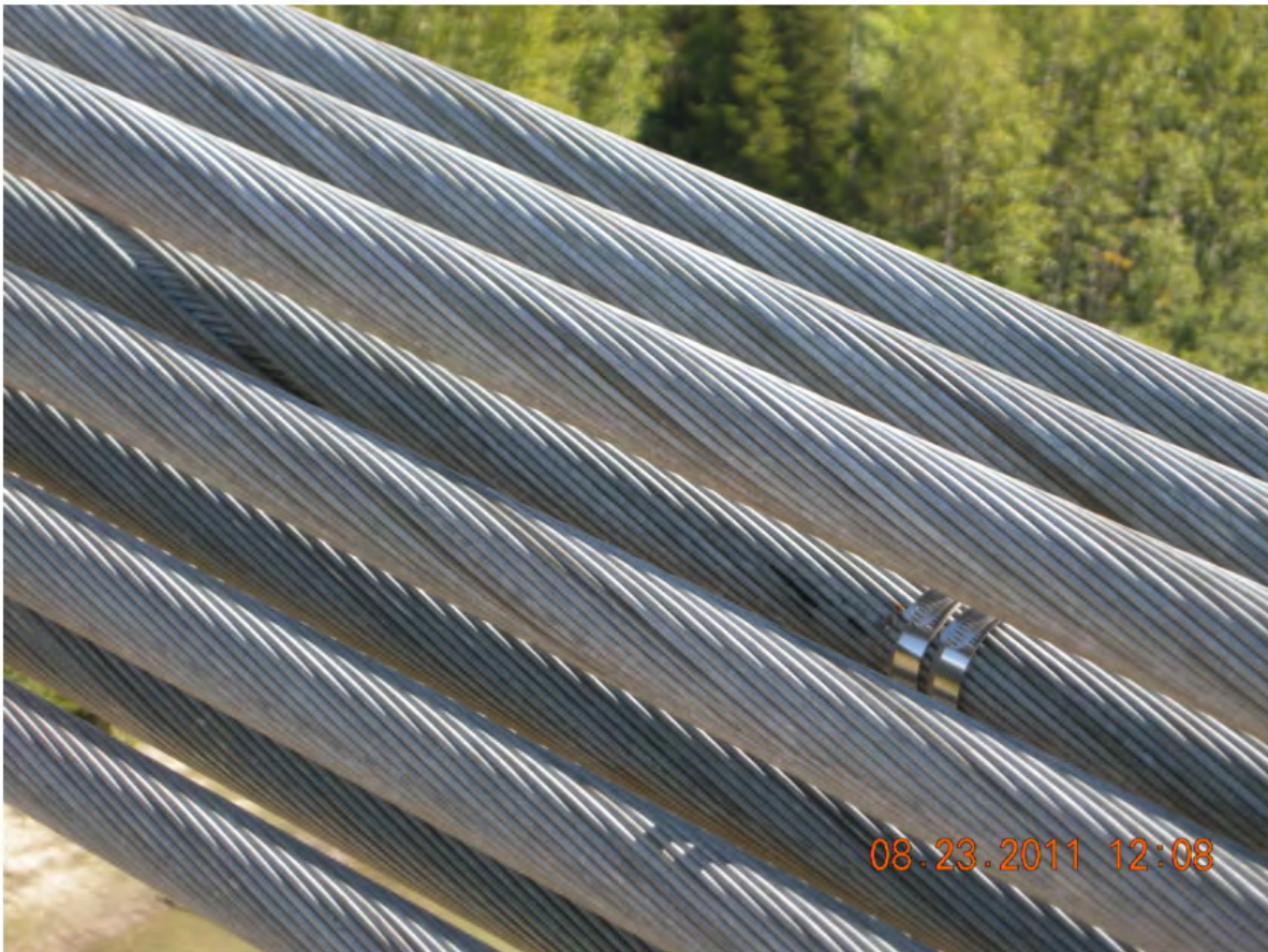
P80 - Span 2 - East Cables 18N to 16N - Two #7 Broken Wires Clamped
