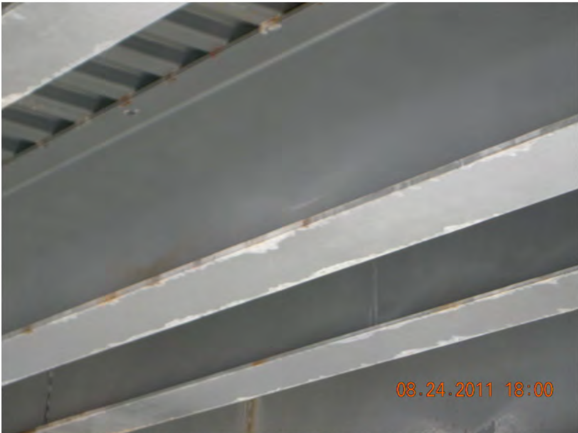
P38 - Span 2 - Near Midspan - Stringer Bottom Chords - Top Coat of Paint Flaking off
