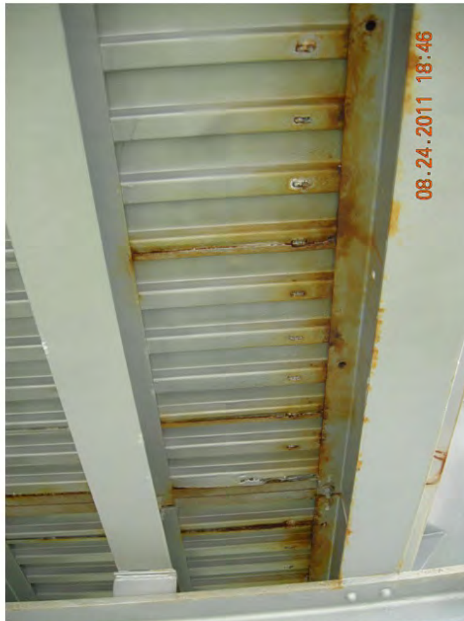
P26 - Span 1 - Corrosion Staining of Permanent Soffit Formwork and West Stringer Top Flange Near Midspan on West Side of Deck
