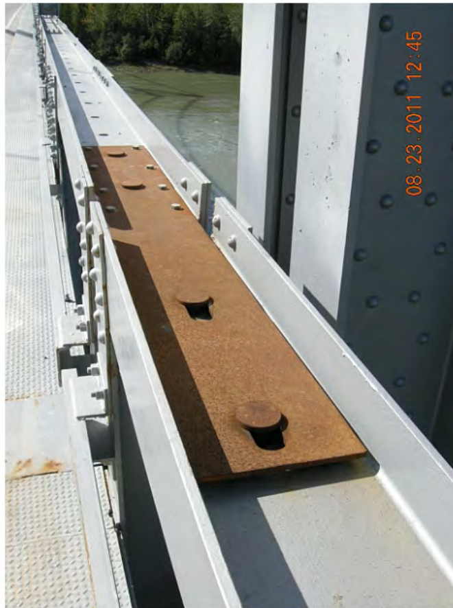
P22 - Deck Stiffening Truss - Expansion Plate on West Top Chord - Similar on East Side
