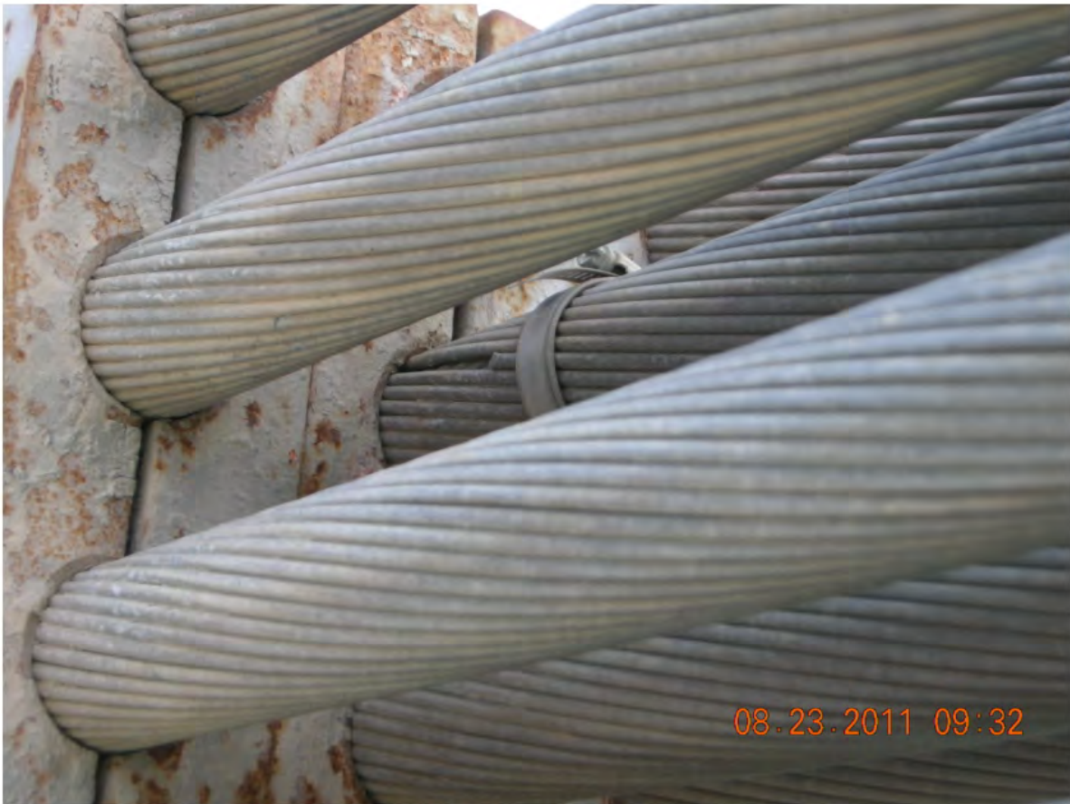
P78 - Span 2 - East Cables 24S to 26S - 1 Clamp on #8
