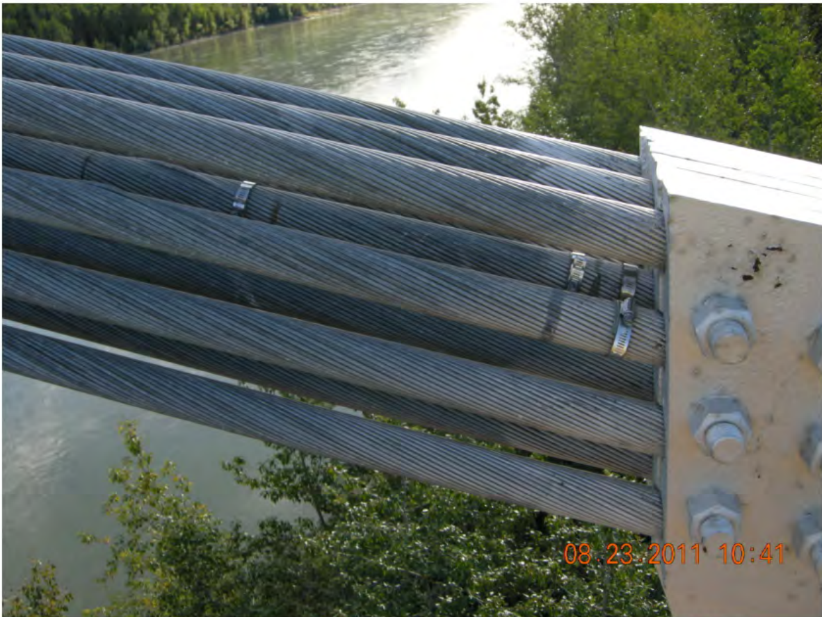
P56 - Span 1 - East Cables 6S to 8S - 1 #7 and 3 #8 Broken Wires Clamped
