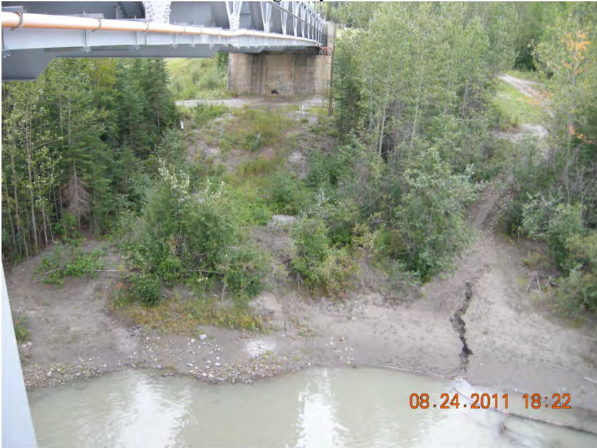
P89 - South Abutment and Embankment - Minor Erosion Gully at Waterline
