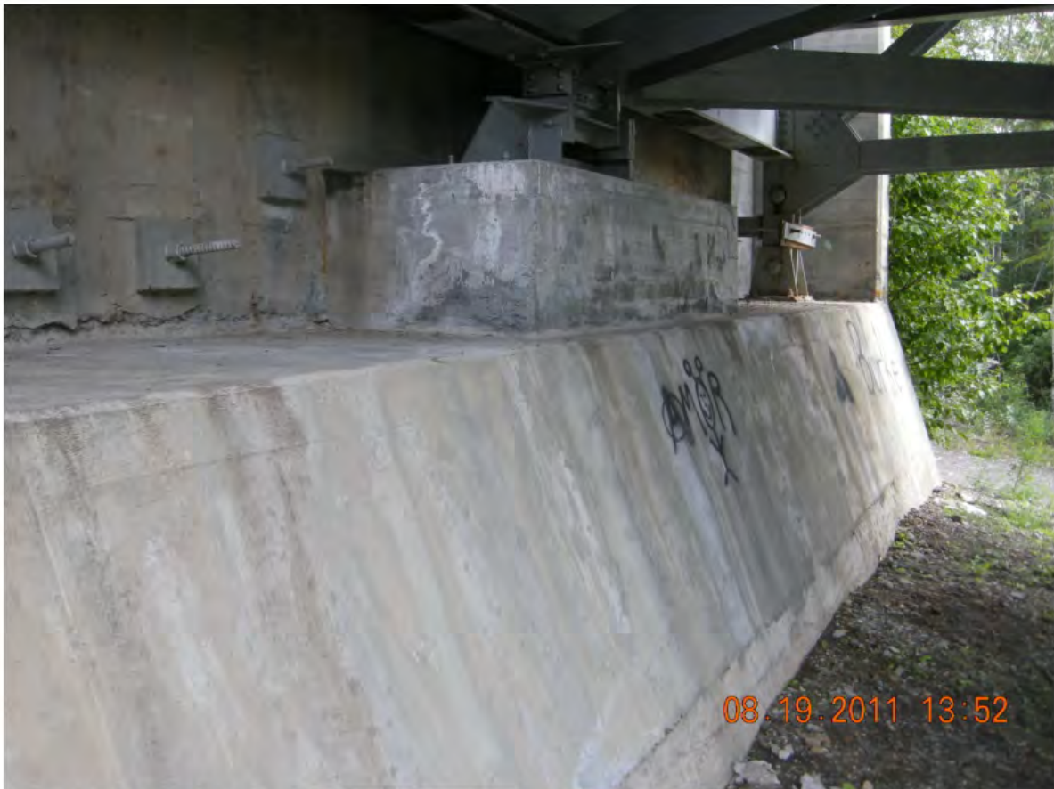
P116 - North Abutment - Repairs Carried out to Spalls in Bearing Seat Since 2009 Inspection
