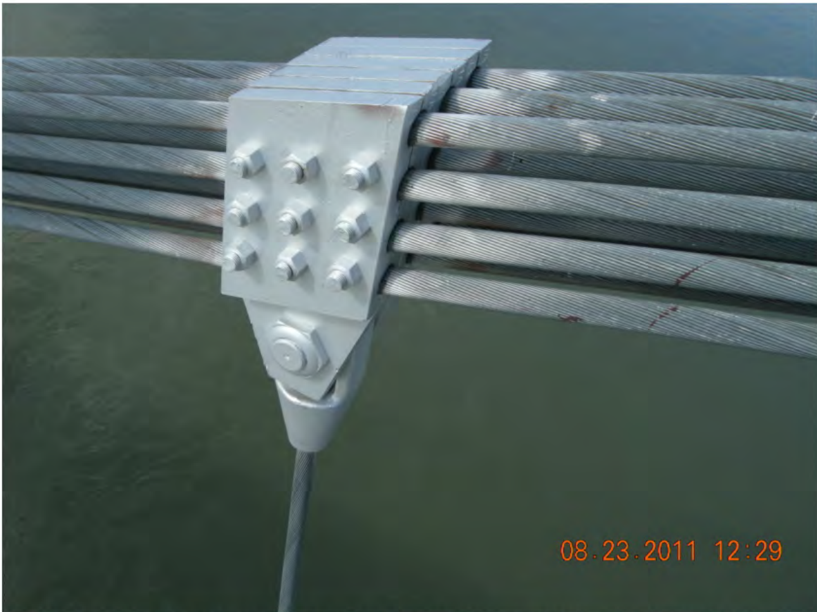
P64 - Span 2 - West Hanger 14N - Slipped 5 mm as Previously Noted - No Additional Slippage
