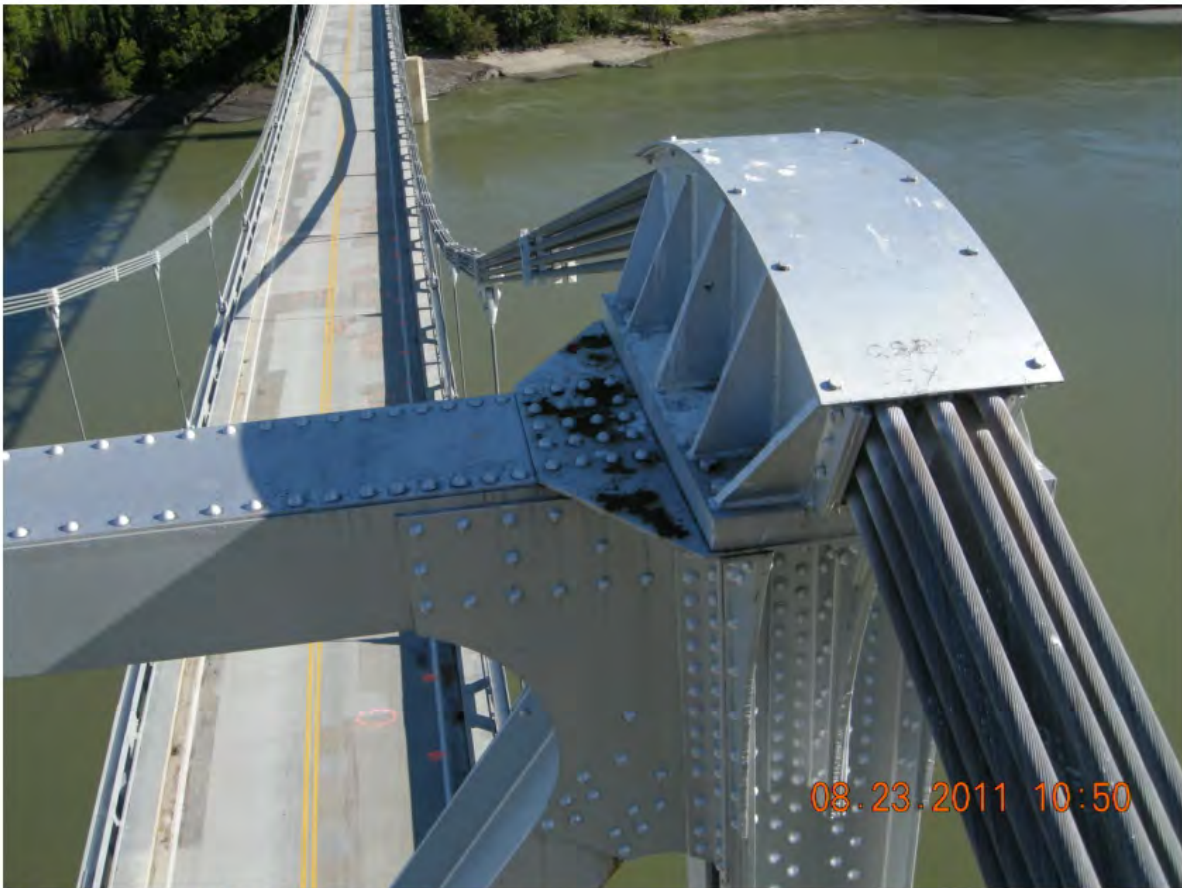
P102 - South Tower - Saddle for East Cables - Paint Peeling and Light Surface Corrosion on top of Gusset Plate
