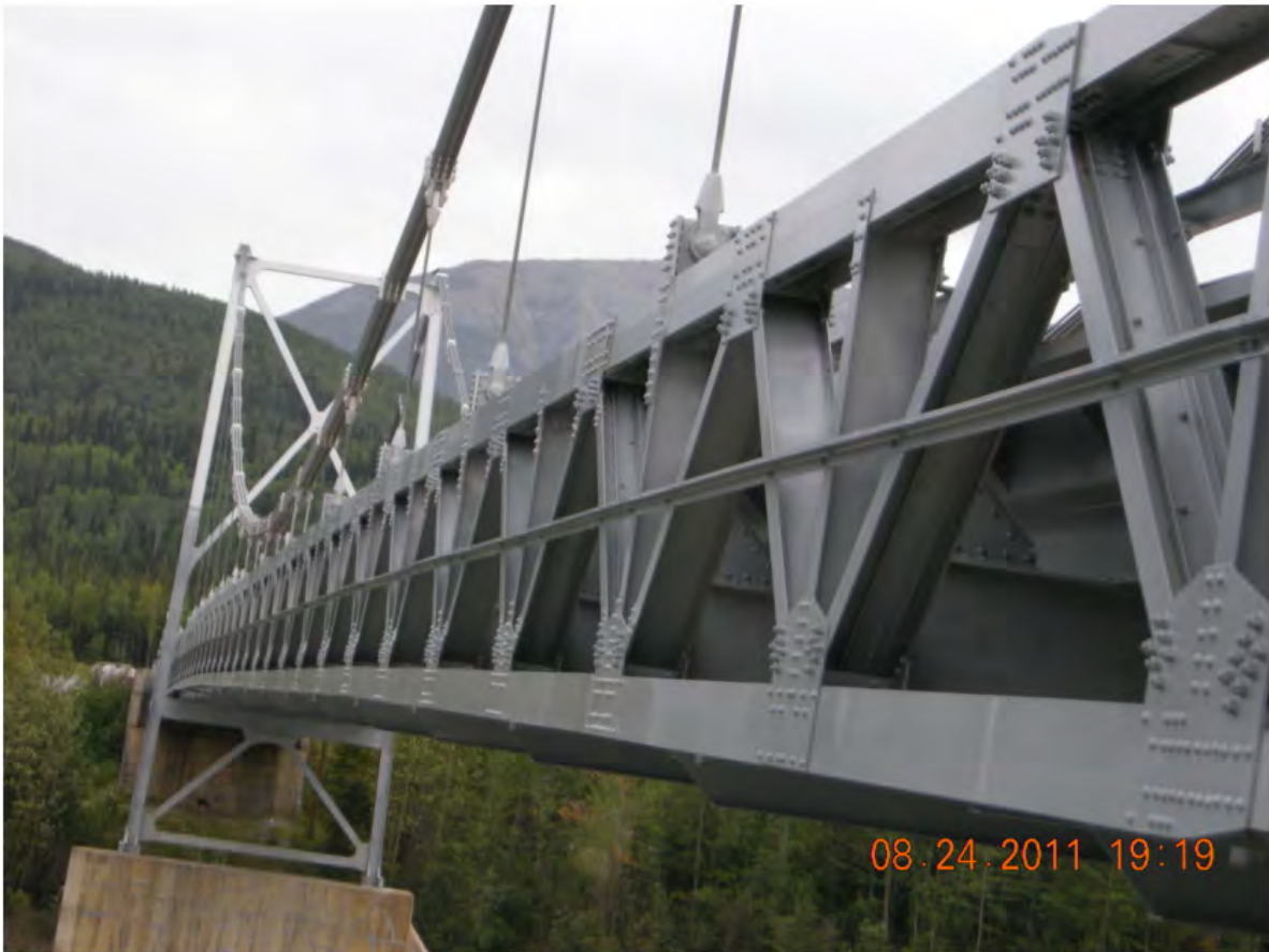
P32 - Span 2 - East Truss Profile - Looking South - Profile Flattens out Near Midspan
