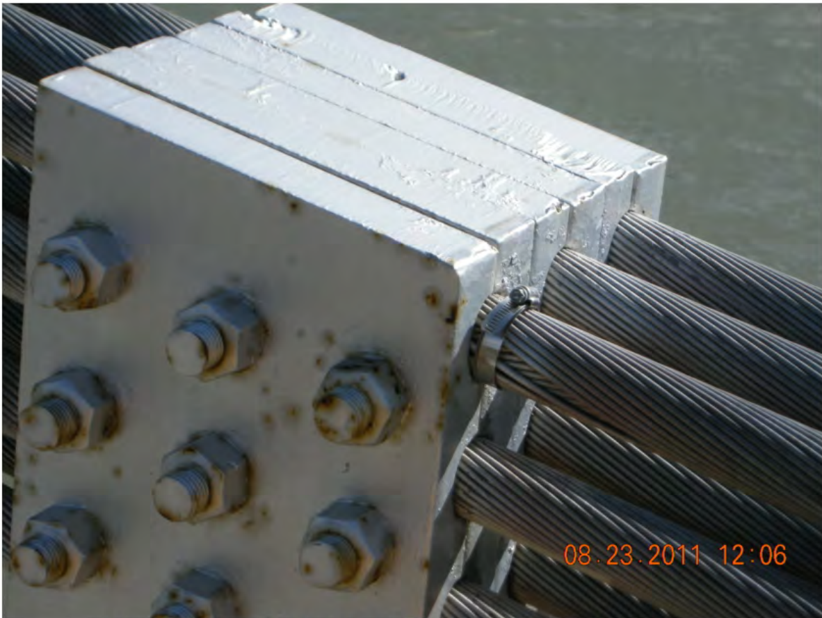
P82 - Span 2 - East Cables 22N to 20N - Three #10 Broken Wires Clamped
