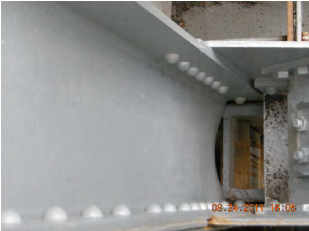
P118 - Deck Truss Vertical at NE Corner of Bridge - Bent Web - No Cracking
