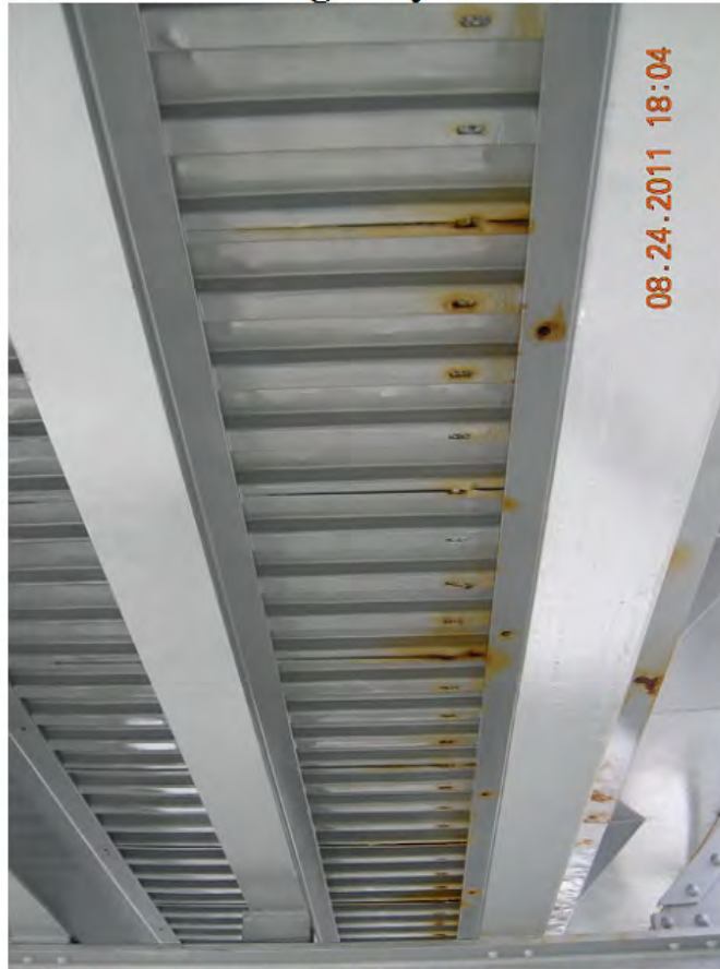
P39 - Span 2 - Corrosion Staining of Permanent Soffit Formwork near Midspan on West Side of Deck
