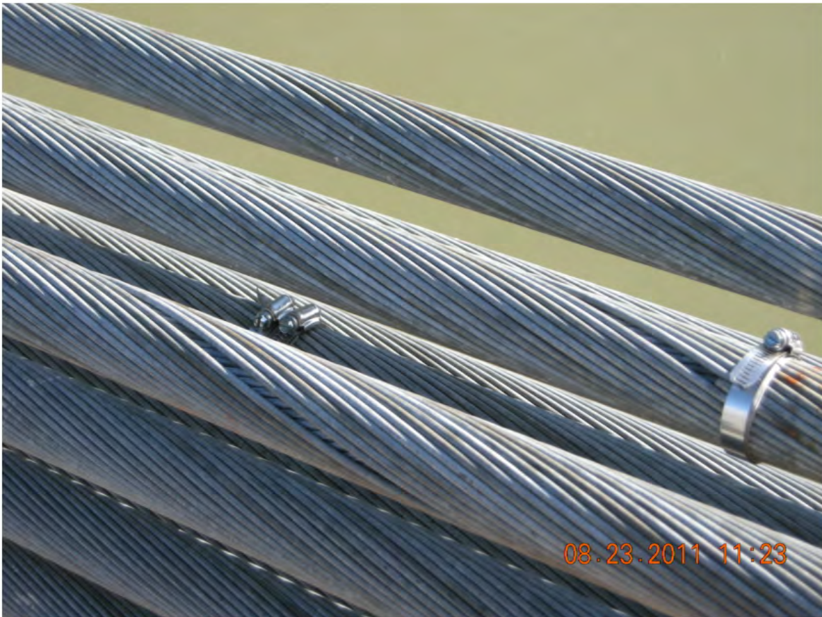
P70 - Span 2 - East Cables 16S to 18S - One #8 and One #11 Broken Wire Clamped
