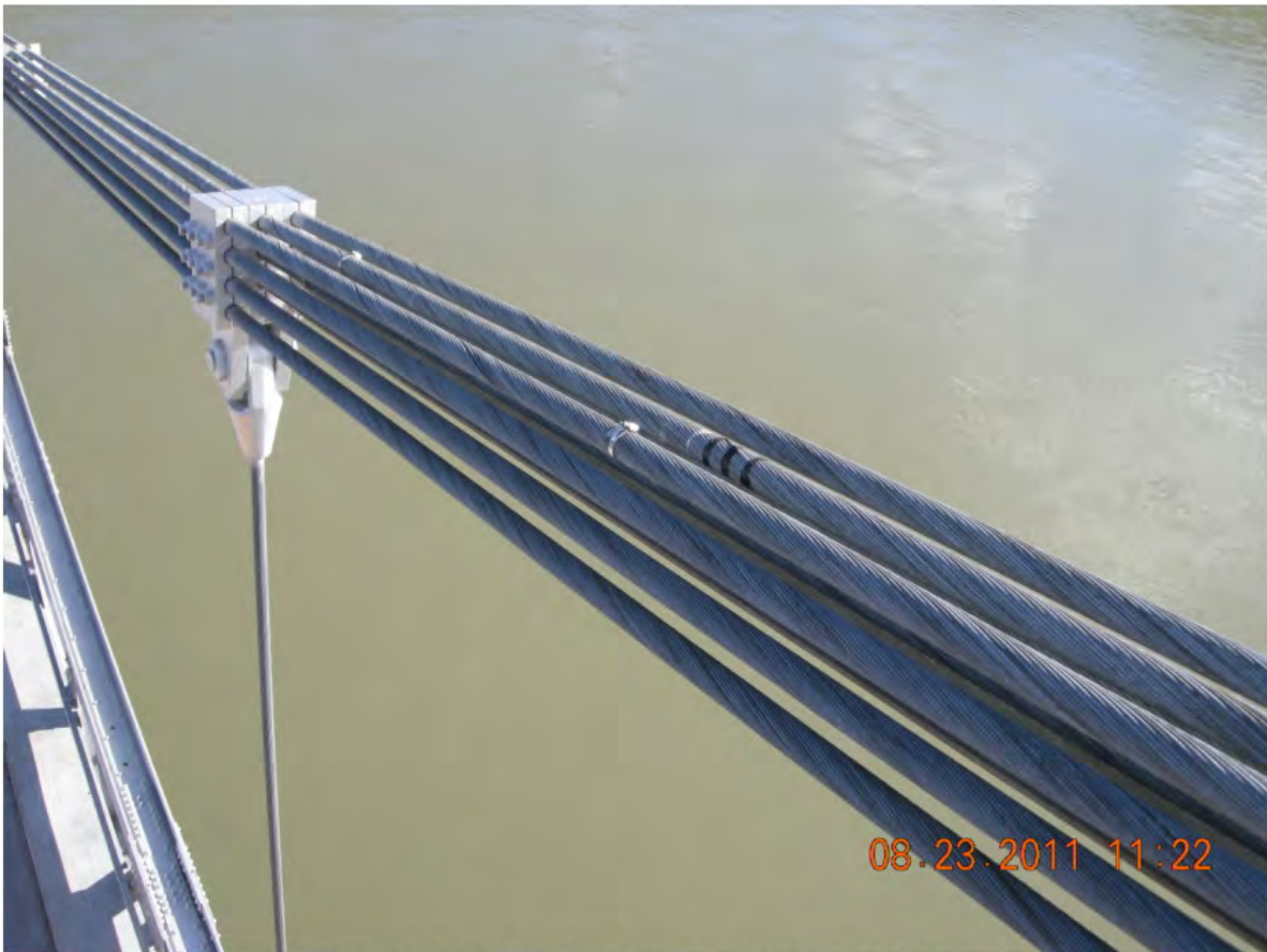
P72 - Span 2 - East Cables 16S to 18S - One #10 and One #11 Broken Wire Clamped
