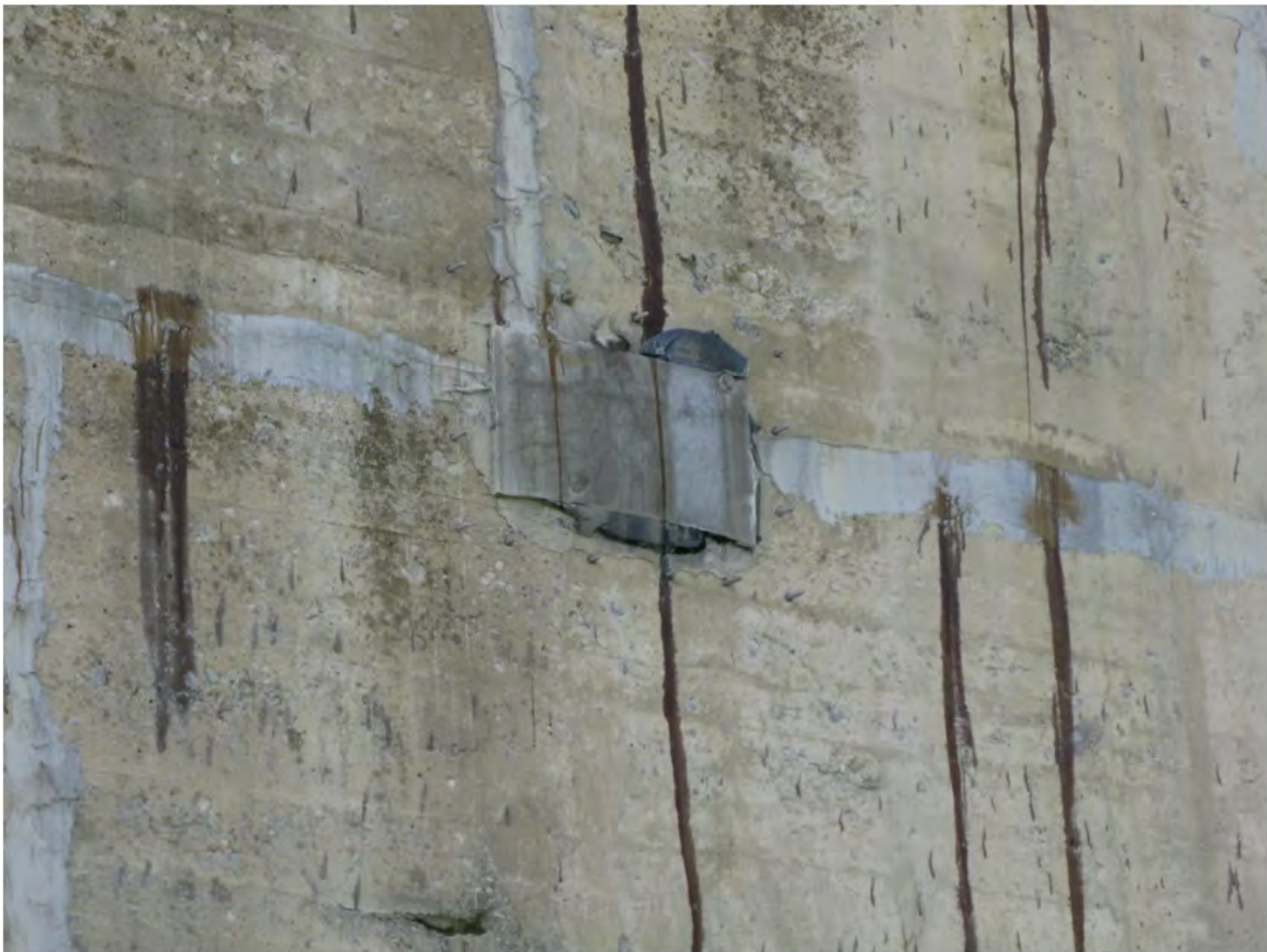
UW04 - Pier 1 Spall repair HC face
