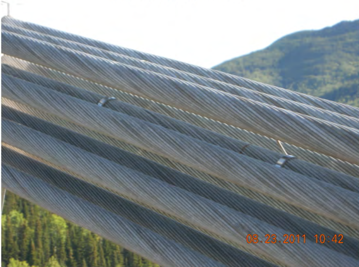
P57 - Span 1 - East Cables 6S to 8S - 2 Additional Clamps on #8 Cable
