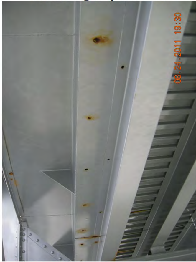
P37 - Span 2 - Rust Staining in East Sidewalk near Midspan
