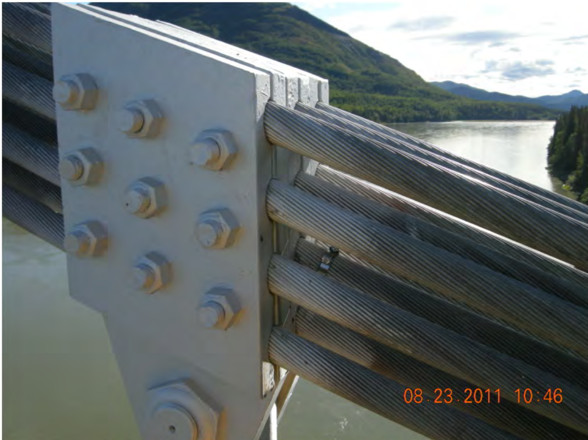
P58 - Span 1 - East Cables 8S to 10S - 1 #5 Broken Wire Clamped
