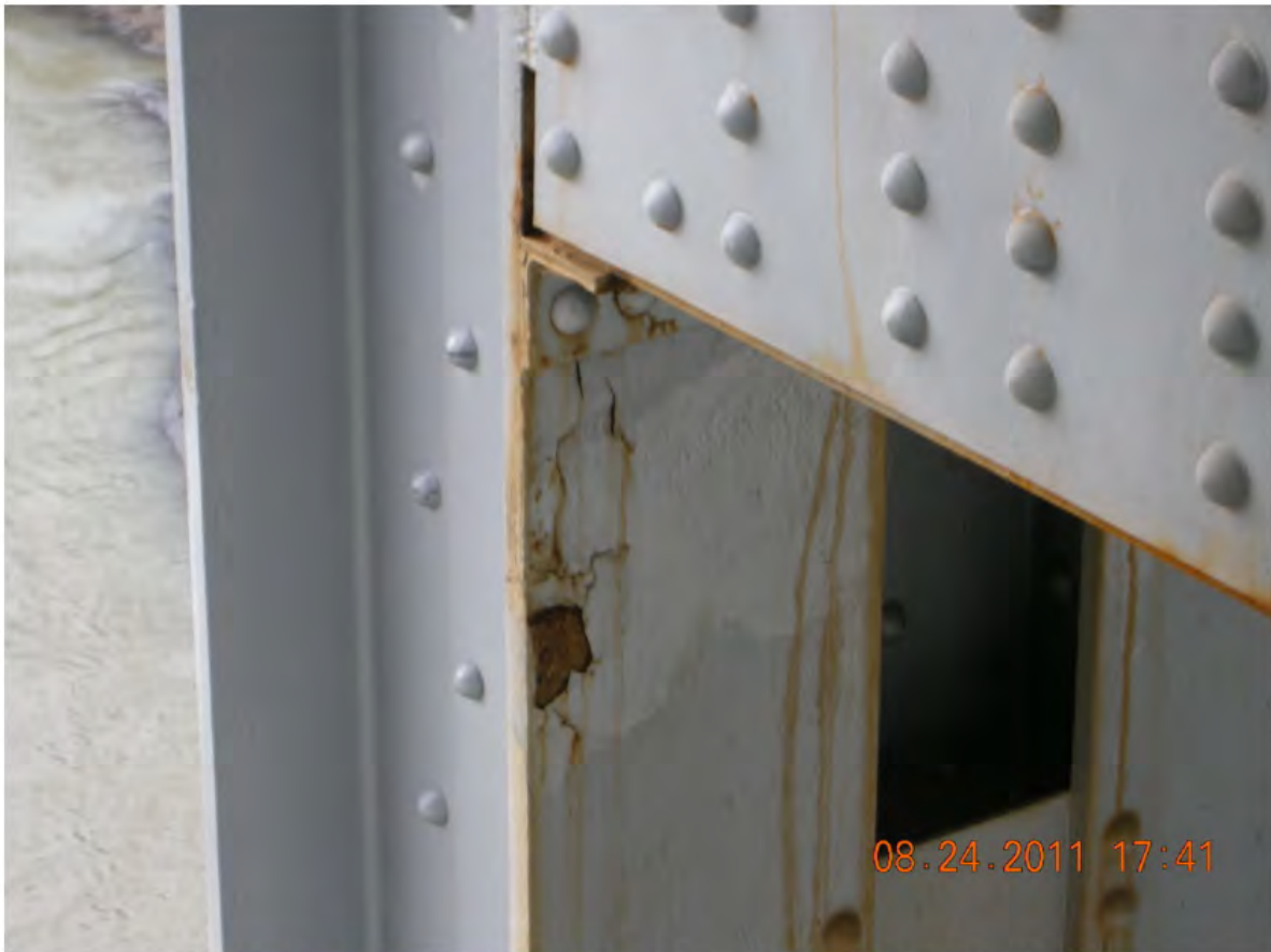
P108 - North Tower - West Leg - Localized Paint Peeling below Deck
