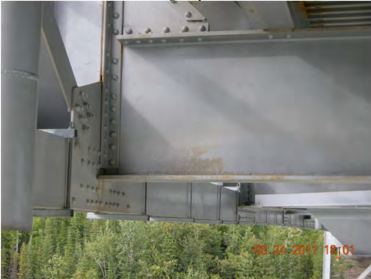
P41 - Span 2 - Floorbeam L10 - Top Coat of Paint Incomplete at West End
