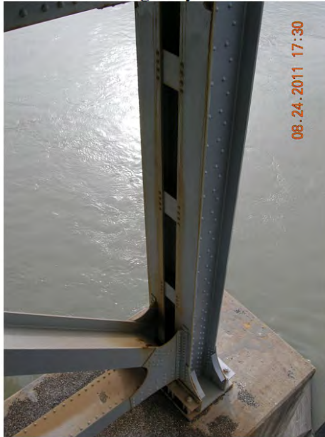
P107 - North Tower - West Leg - Corrosion Staining Leaking from Unpainted Interior of Leg
