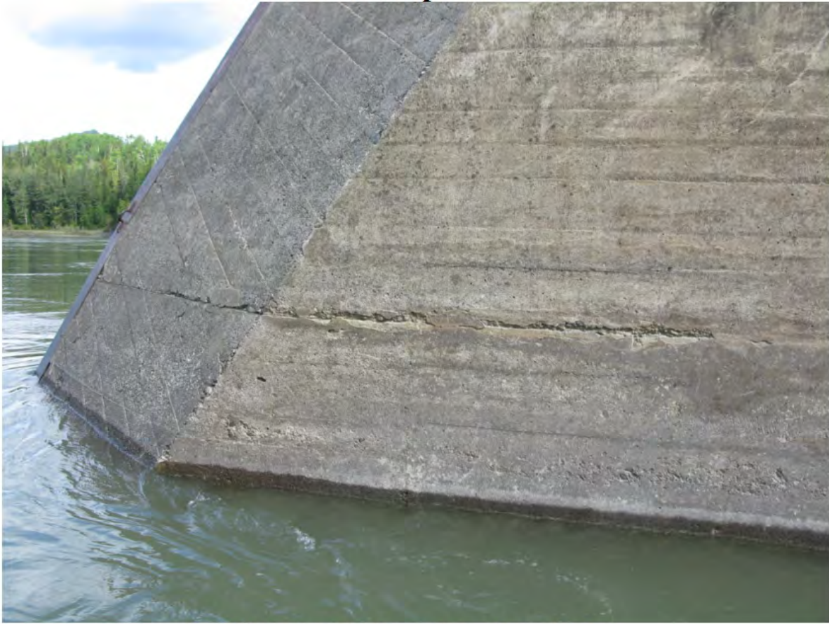
UW07 - Pier 1 LC face spall at cold joint 5m long
