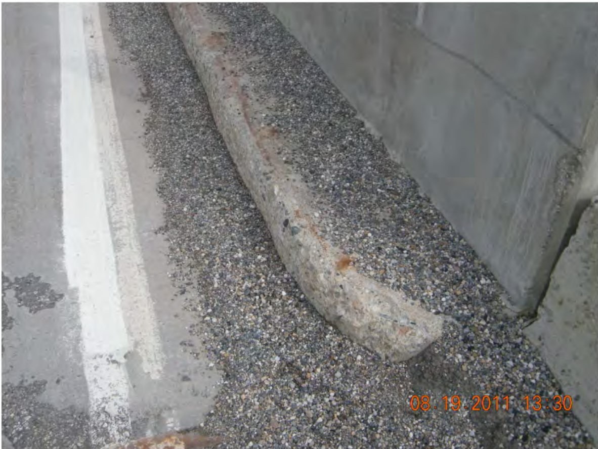
P18 - South Abutment Curbs - Medium Scaling from Snowplow Abrasion
