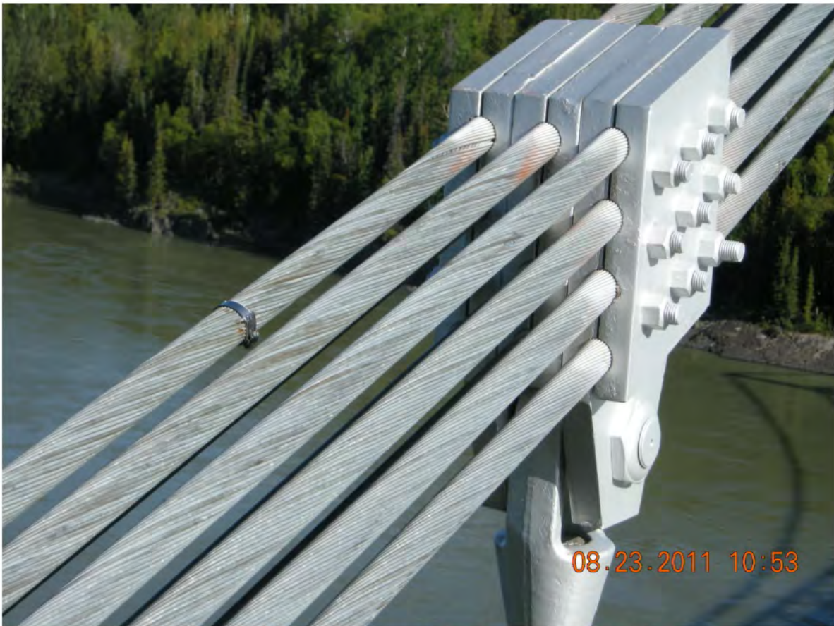
P54 - Span 1 - West Cables 8S to 10S - 1 #10 Broken Wire Clamped
