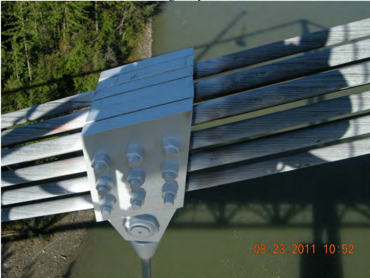
P55 - Span 1 - West Hanger 10S - Slipped 5 mm as Previously Noted - No Additional Slippage
