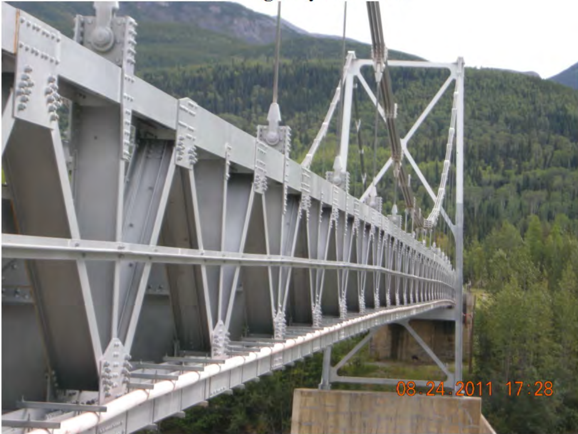
P31 - Span 2 - West Truss - Looking South - Fibre Optic Cable along Bottom Chord - Profile Flattens out Near Midspan
