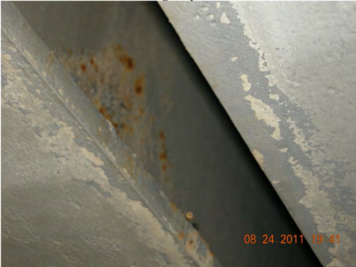
P27 - Span 1 - South Tower Floorbeams at L12 - Corrosion on Floorbeam Web below Finger Joint
