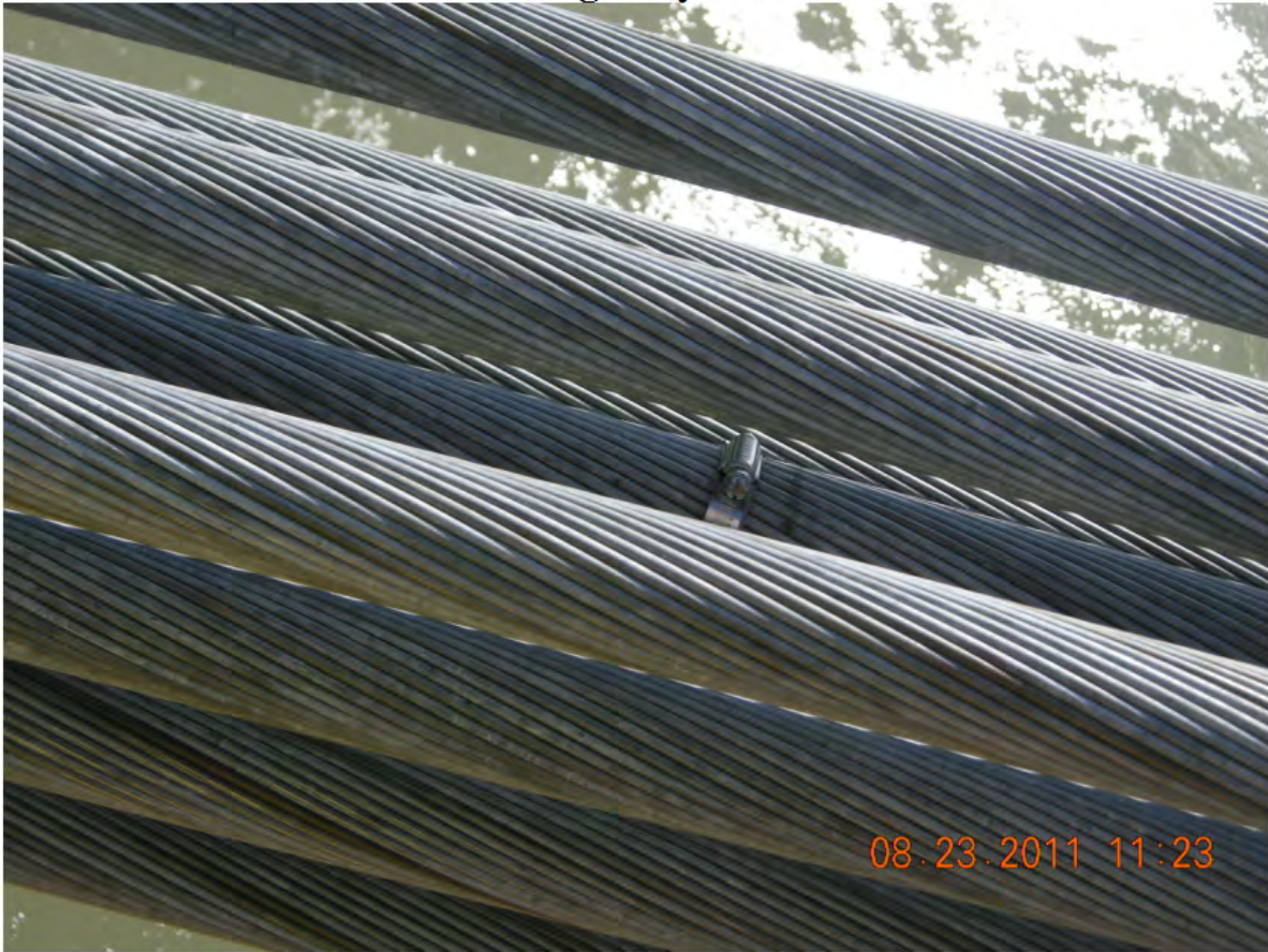
P71 - Span 2 - East Cables 16S to 18S - One #8 Broken Wire Clamped
