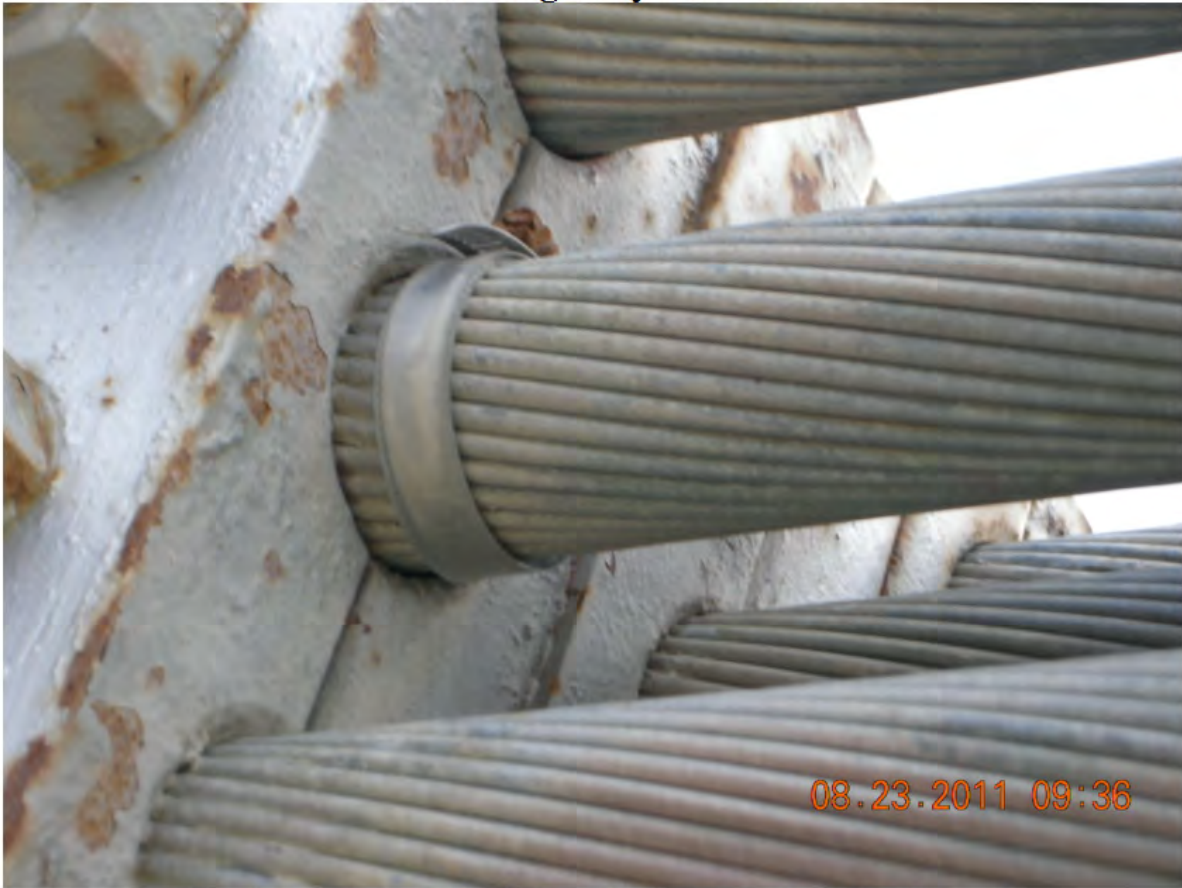
P77 - Span 2 - East Cables 22S to 24S - One #7 Broken Wire Clamped
