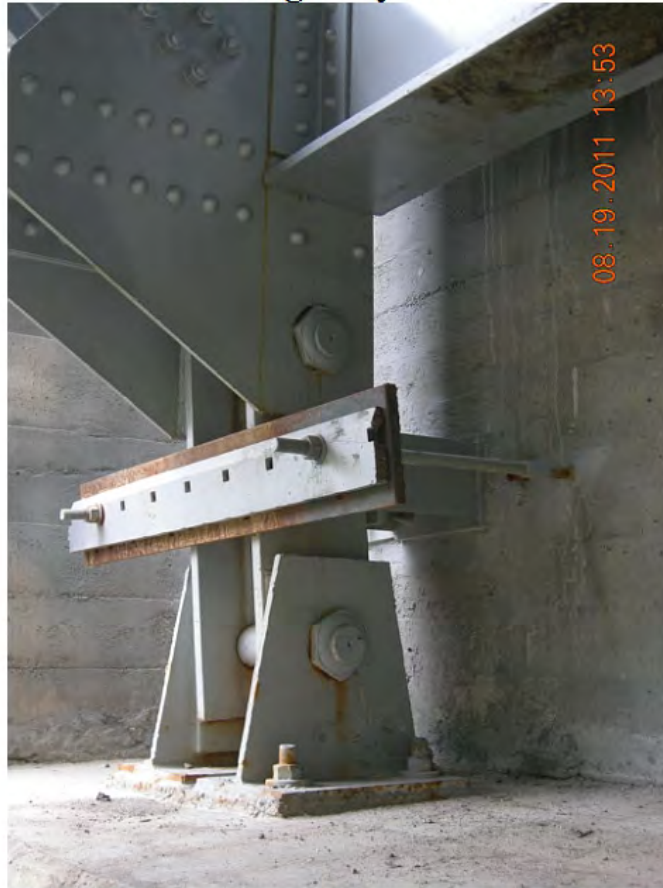
P117 - North Abutment - Keeper Bars at NW Bearing
