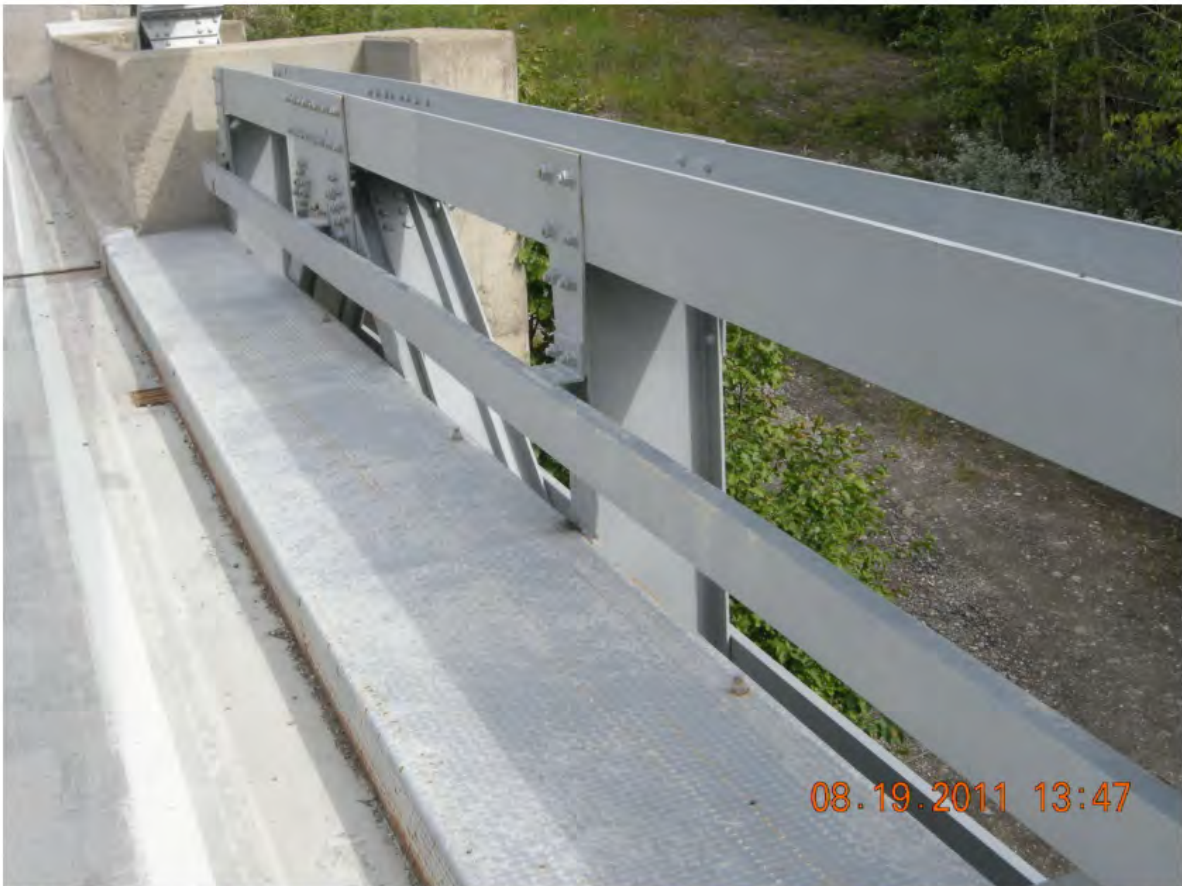
P20 - Bridge Railing - Channel Secured to Stiffening Deck Truss - Narrow Steel Sidewalks both Sides of Bridge
