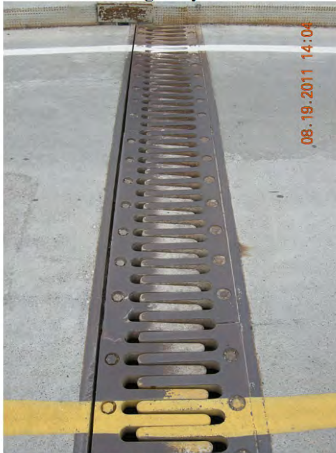
P13 - North Tower - Finger Joint - One Set of Fingers has Dropped 22 mm in West Lane - Rattles Loudly under Traffic
