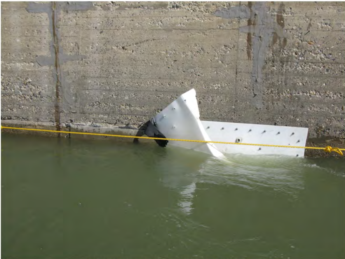
UW20 - Pier 2 LC face 16' from DS damage repair
