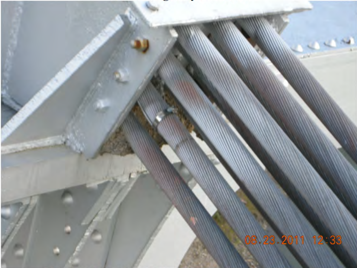
P63 - Span 2 - West Cables 14N to 12N - One #6 Broken Wires Clamped
