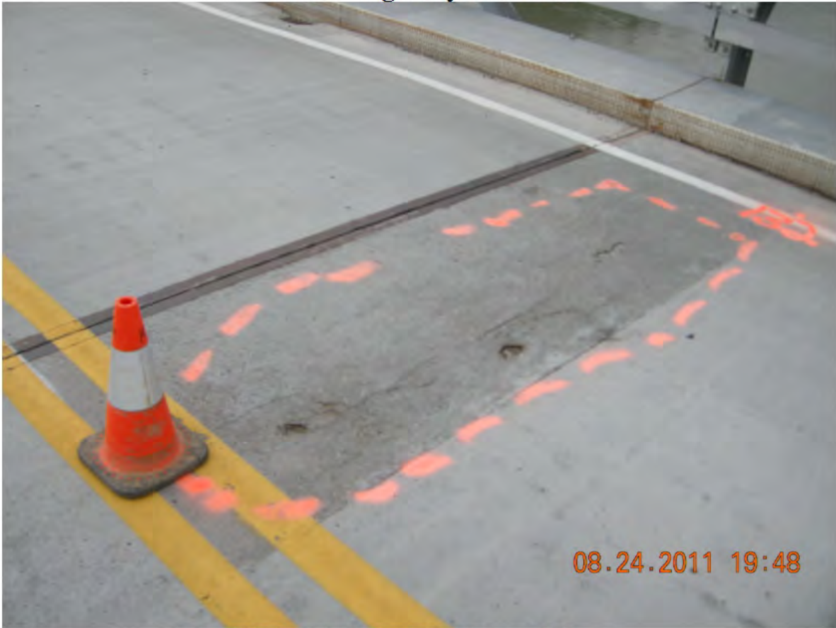
P09 - Span 2 - Potholes Forming near Midspan
