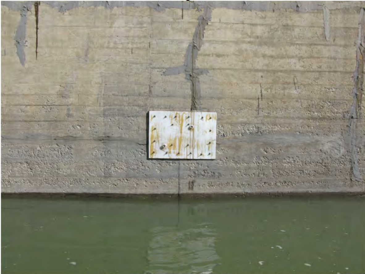
UW09 - Pier 1 Spall repair LC face 1.5' above water 2
