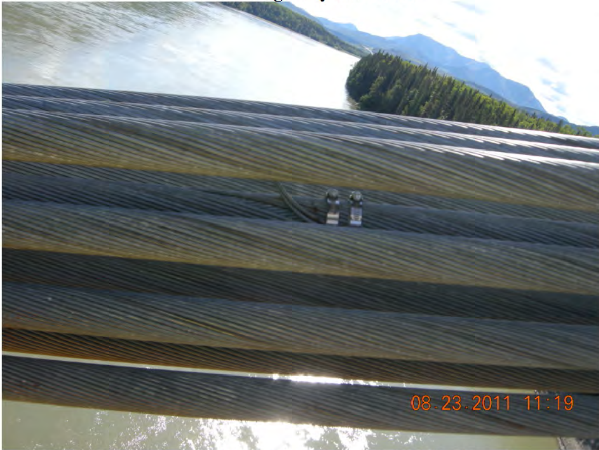
P69 - Span 2 - East Cables 14S to 16S - Two #8 Broken Wires Clamped
