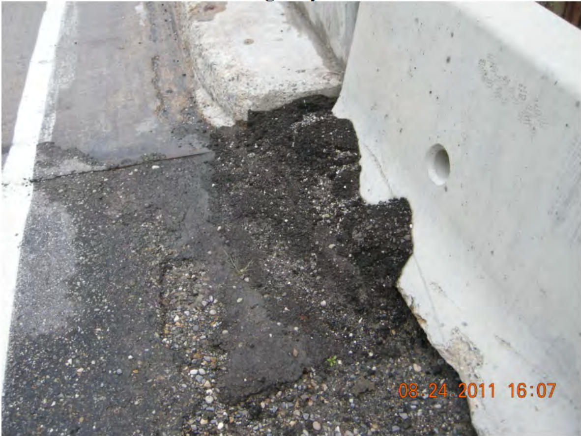
P19 - North Abutment - NW Curb - Asphalt Taper is Eroding Away
