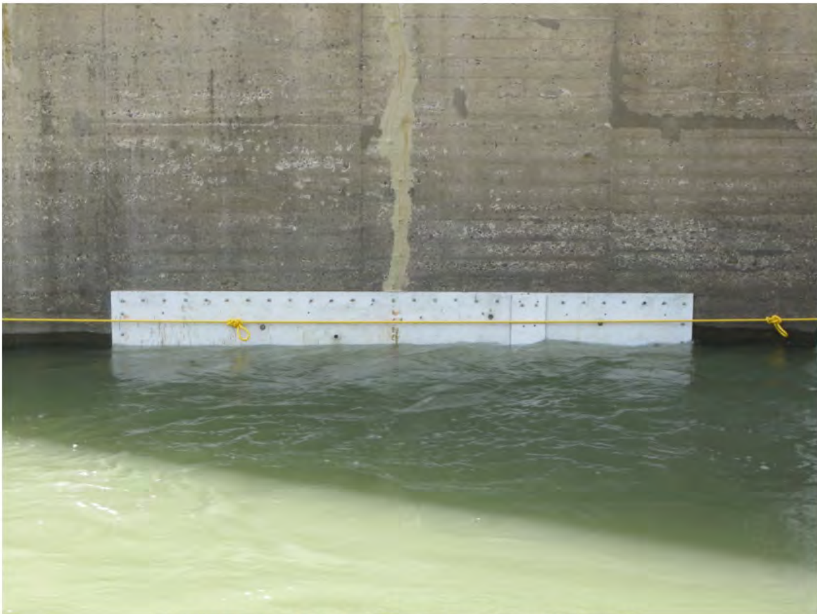
UW14 - Pier 2 HC face close up horz repair 33' from US
