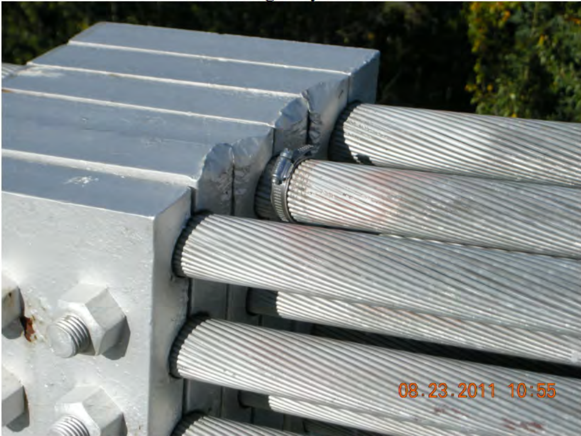
P53 - Span 1 - West Cables 6S to 8S - 1 #11 Broken Wire Clamped
