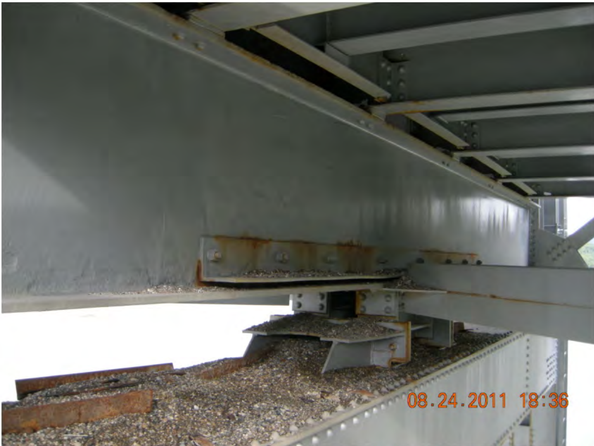
P28 - South Tower - Gravel Leaking through Finger Joint onto Horizontal Surfaces - Rust Staining from Unpainted Surfaces
