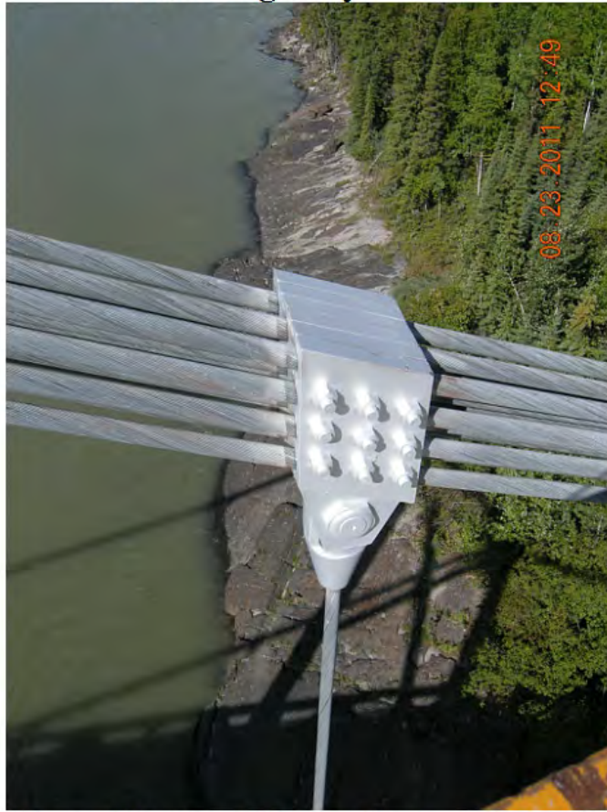
P87 - Span 3 - West Hanger 10N - Slipped 25 mm as Previously Noted - No Additional Slippage
