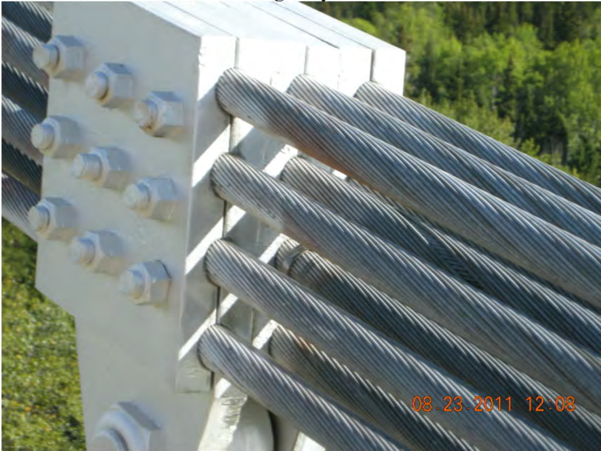
P79 - Span 2 - East Cables 18N to 16N - One #5 Broken Wires Clamped
