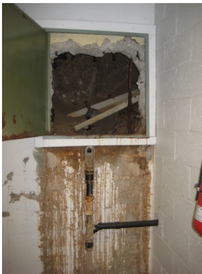
Figure S-1 (left): Existing access hole cut in foundation wall at water leak from storm drain
