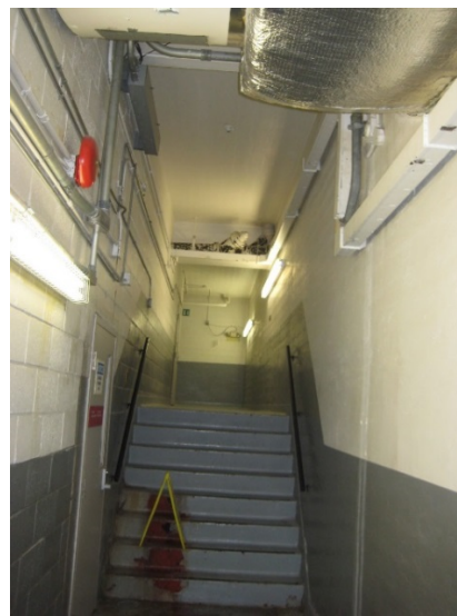
Figure S-2 (right): Signs of water leak in basement corridor stairs
