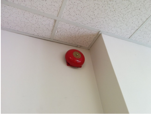
E-Figure 15 Non-conformant bells, typical
