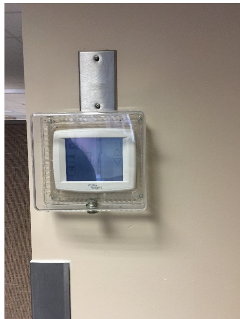
M-Figure 10 Existing Thermostat
