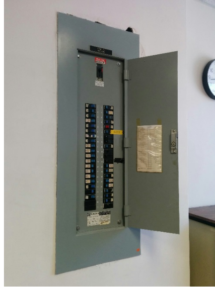
E-Figure 4 Typical 120/208V panelboard
