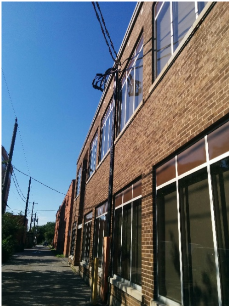
E-Figure 1 Incoming Service and pole mounted transformers in background
