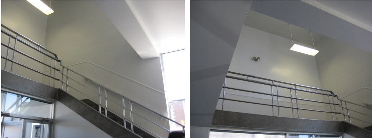
Figure S-4 A&B: Existing north-east staircase to be removed
