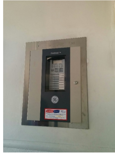
E-Figure 16 Recently replaced main fire alarm panel, good condition
