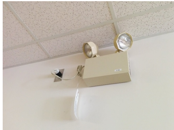
E-Figure 8 Typical emergency battery unit with lamp heads
