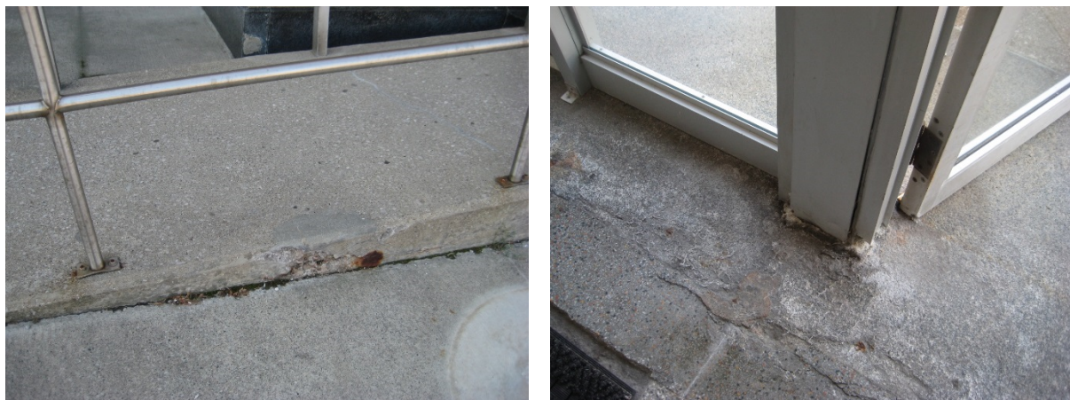
Figure S-3 A&B: Signs of concrete spalling at north-west main entrance
