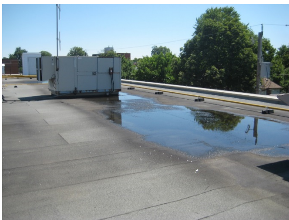
Figure S-6: Sagging of roof deck and water ponding
