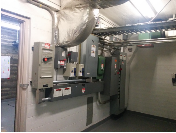
E-Figure 3 600V Splitter and Disconnects – Recommended for replacement
