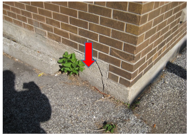
Figure 19 Foundation Cracking S/E Corner (Photo: DIALOG 07-15-15)
