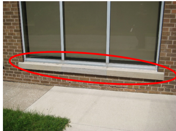
Figure S-9: Spalling of exterior brick face
