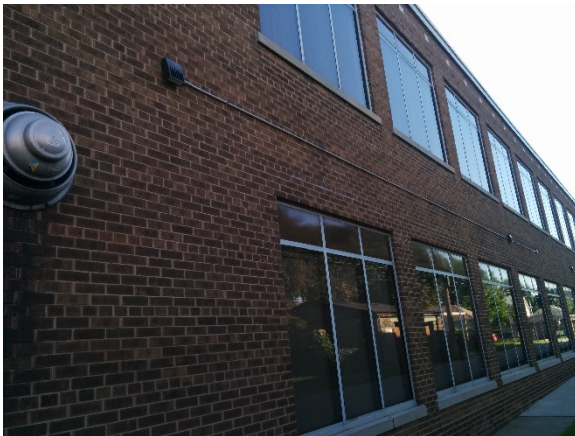
E-Figure 7 Typical Exterior LED Lighting
