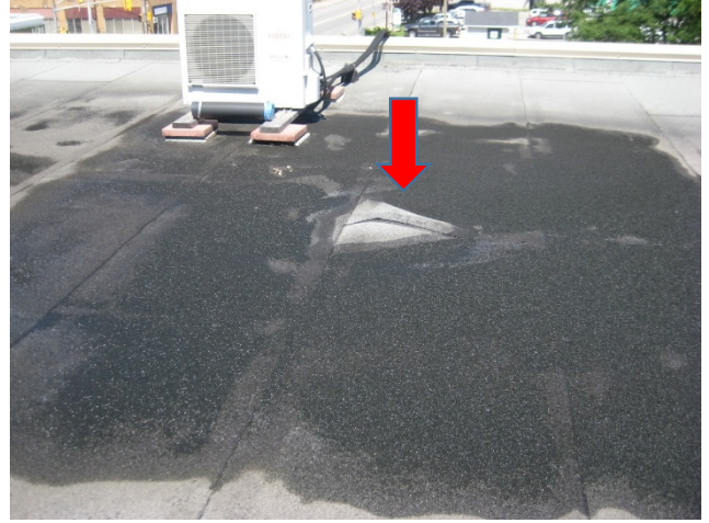
Figure 13 Delaminating Roof Membr. (Photo: DIALOG 07-15-15)
