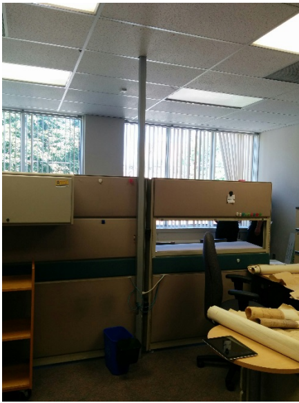
E-Figure 5 Typical Office Fluorescent Troffer
