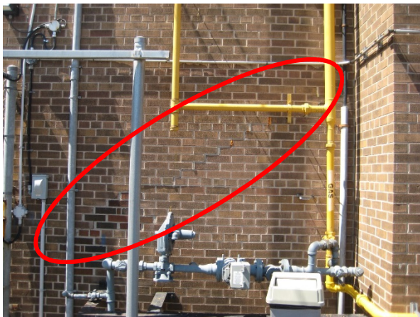
Figure S-7: Cracking in existing exterior brick veneer at south-west elevation
