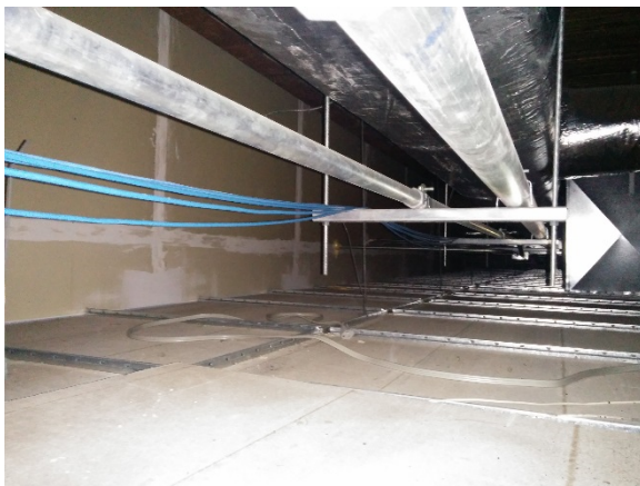
E-Figure 9 Typical Loose Horizontal Communications Wiring
