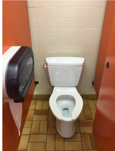
M-Figure 2 Existing Water Closet
