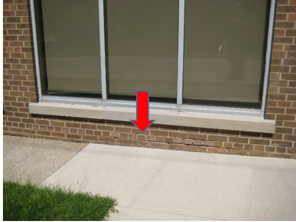
Figure 7 Spalling of Brick Veneer (Photo: DIALOG 07-15-15)
