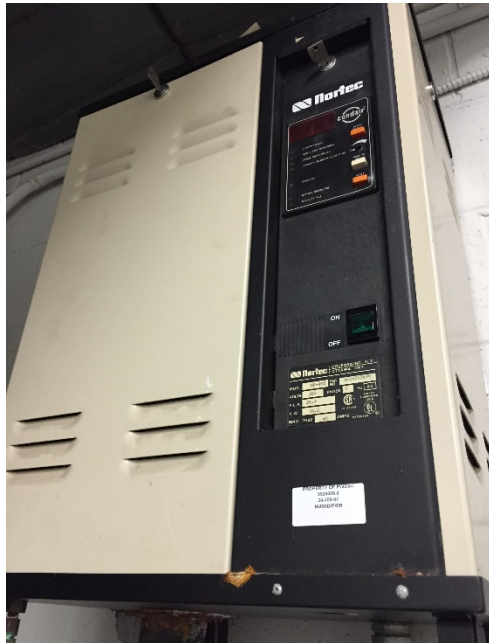
M-Figure 3 Existing Humidifier
