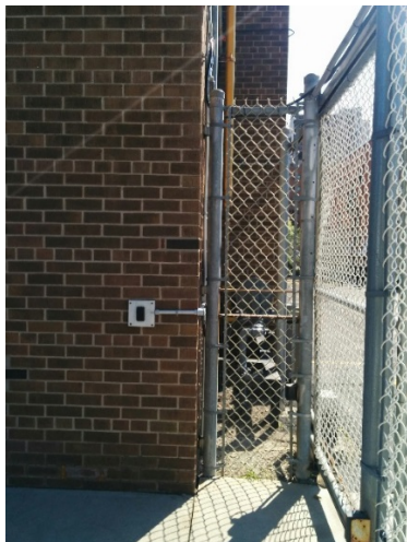
E-Figure 13 Exterior gate access card reader on base building security system
