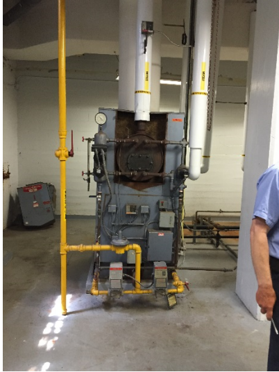
M-Figure 7 Existing Boiler
