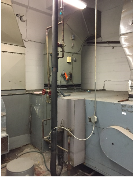
M-Figure 1 Existing Indoor AHU
