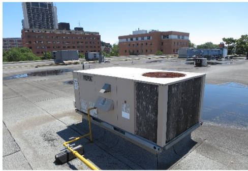
M-Figure 5 Existing Rooftop Units
