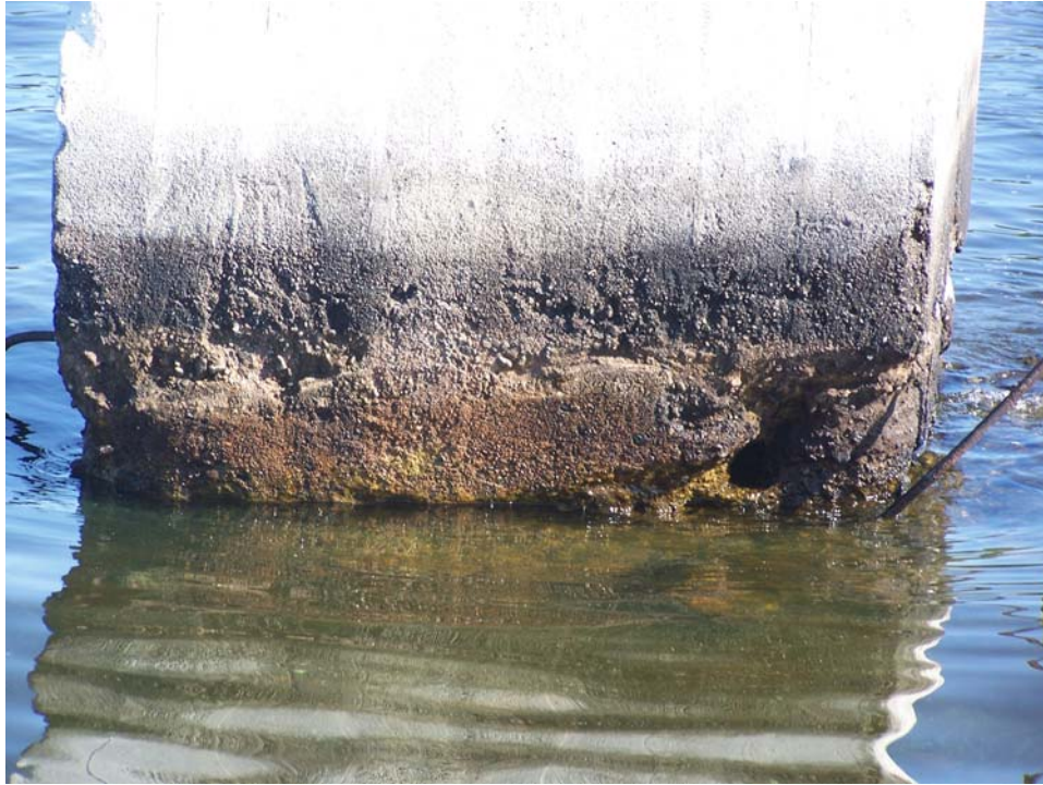
Existing concrete pier (extends below waterline) Concrete to be removed to bedrock elevation
