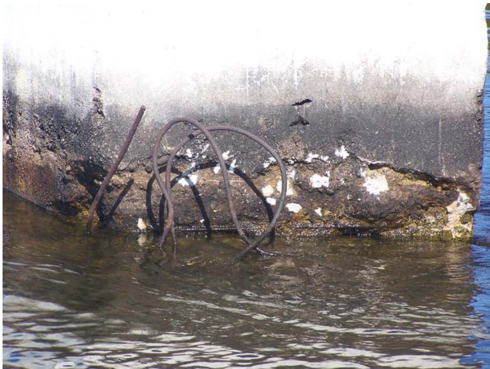
Existing concrete pier, exposed reinforcing steel to be cut flush to bedrock elevation
