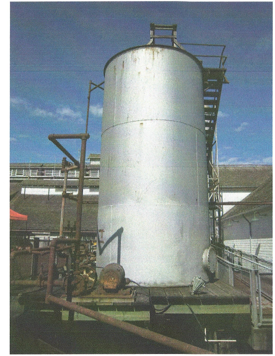
FISH OIL TANKS - 1
