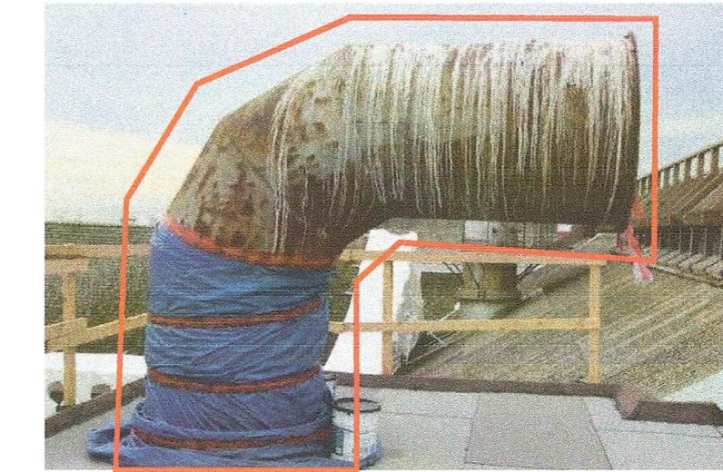
3 EXISTING DRYER ADDITION EXHAUST VENT
