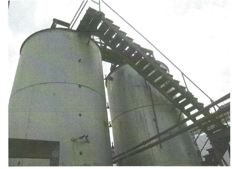
FISH OIL TANKS - 5
