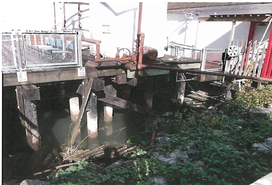
Photo # 6: Timber Deck and Timber Piles supporting the Fish Oil Tank Artifact
