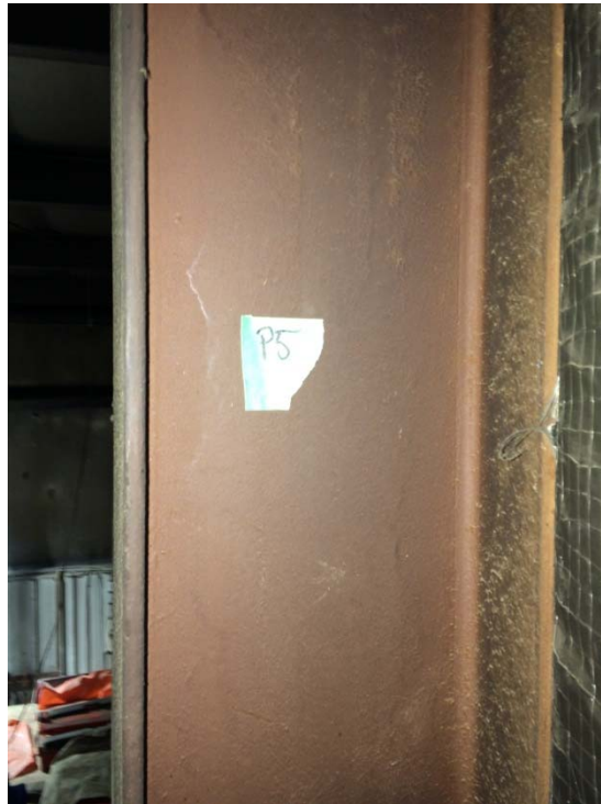
Photograph 5: Sample P5 – Maintenance Garage – Lead-containing red paint on the framing I-beams.
