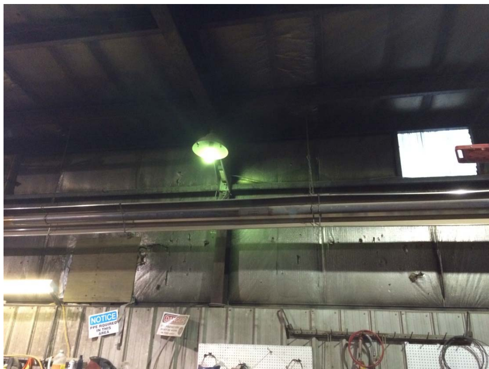
Photograph 12: Suspect PCB-containing HID ballast in the Maintenance Garage. This HID was the only wall-mounted HID identified.
