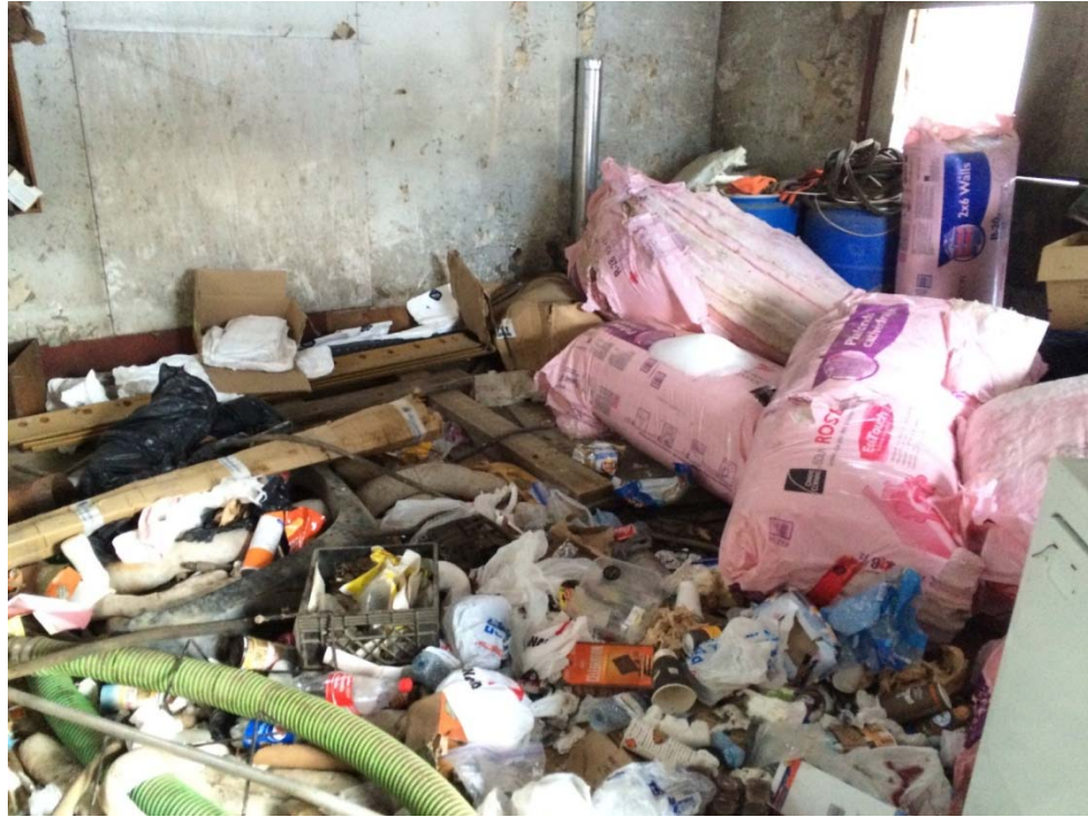
Photograph 27: Old Generator Shed – garbage and debris throughout building.
