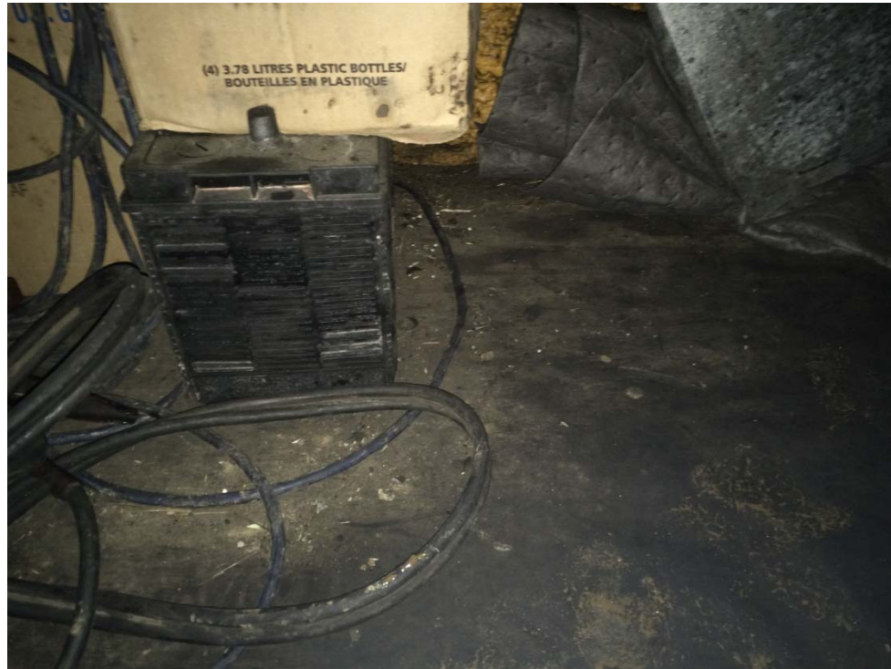
Photograph 25: New Generator Shed – battery & absorbent pads.
