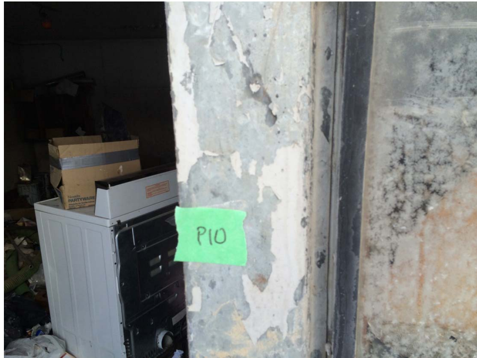
Photograph 11: Sample P10 – Old Generator Shed – Lead-containing grey paint on the entry door.
