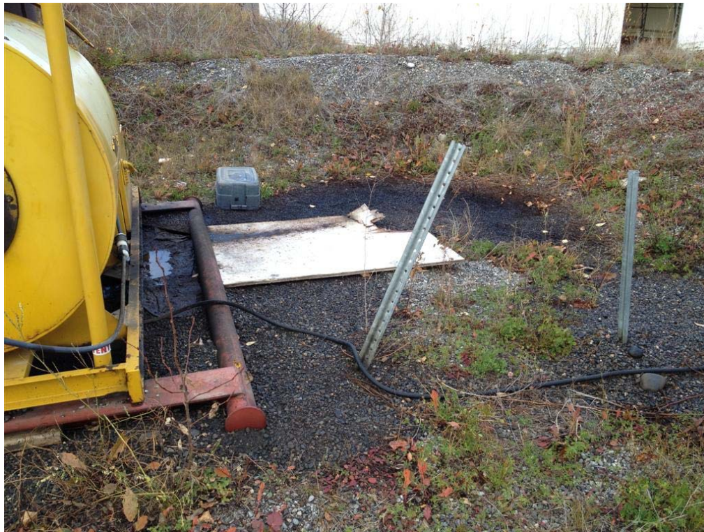
Photograph 5: Spillage from fuel storage to be disposed of offsite as Hazardous Waste.
