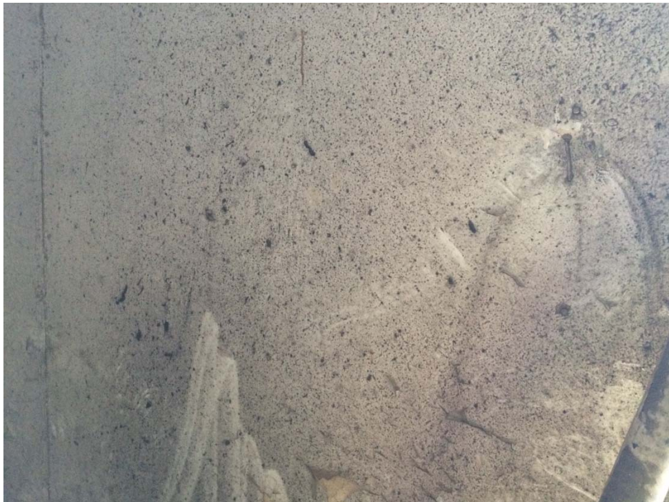
Photograph 28: Old Generator Shed – mould on entrance wall left side (behind door).
