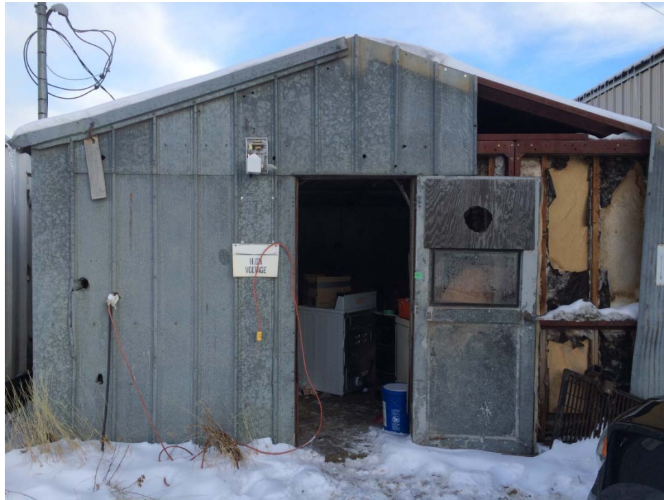
Photograph 15: Suspect PCB-containing HID fixture on the exterior of the Old Generator Shed.
