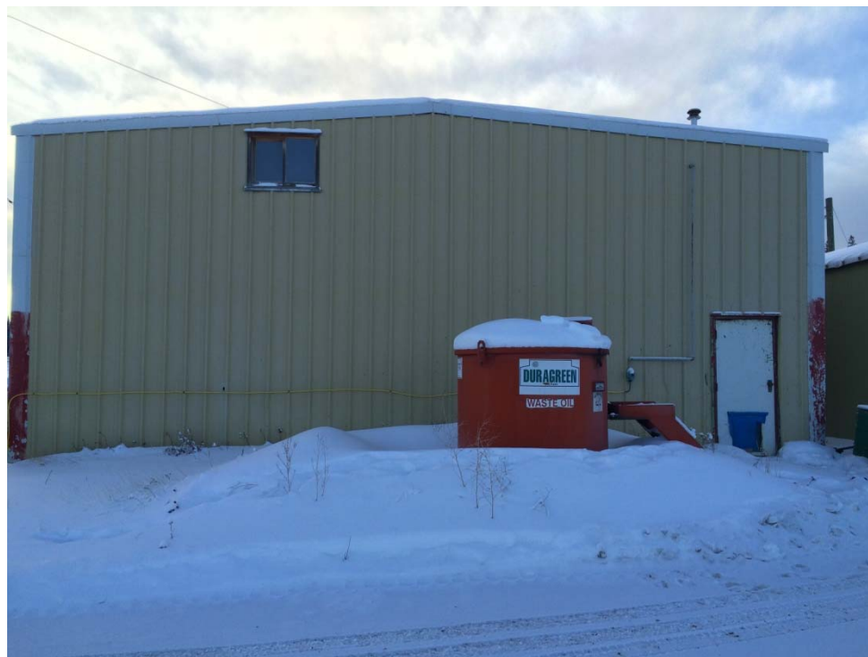
Photograph 8: Sample P17 – Maintenance Garage – Lead-containing yellow paint on the exterior. A waste oil tank is also visible.
