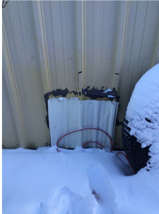
Photograph 3: Sample A14 – Maintenance Garage – Asbestos-containing black mastic surrounding a patch on the exterior wall.
