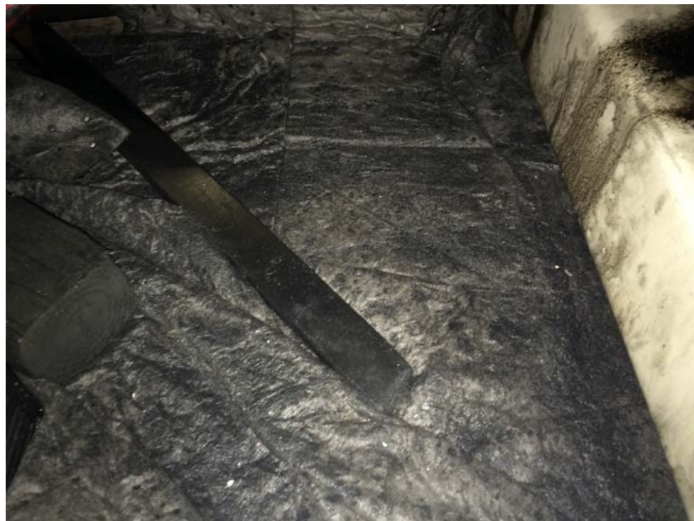
Photograph 26: New Generator Shed – absorbent pads under generator.
