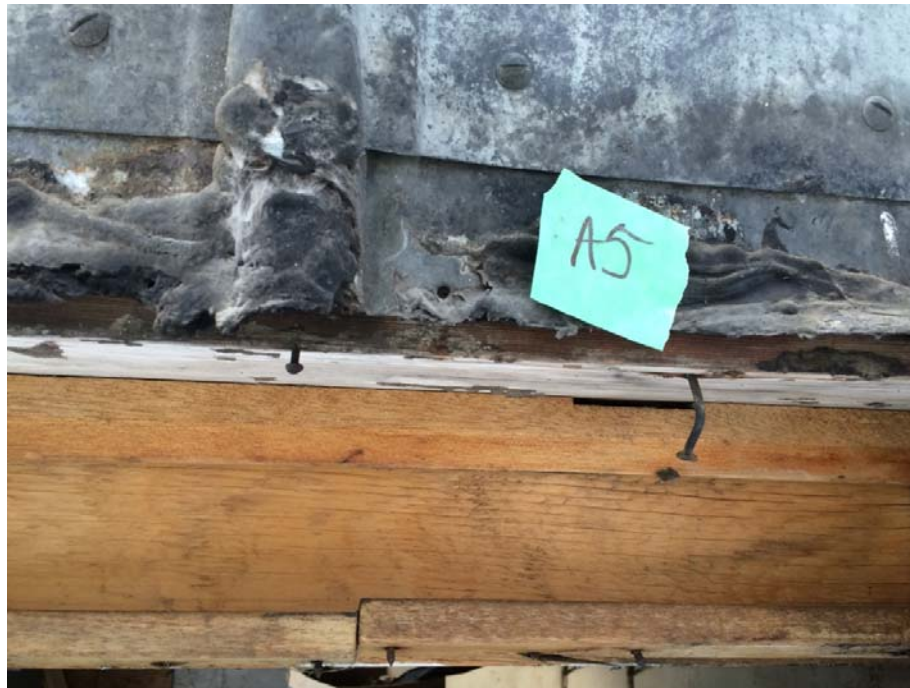
Photograph 1: Sample A5 – Old Generator Shed - Asbestos-containing black mastic above the exterior window.
