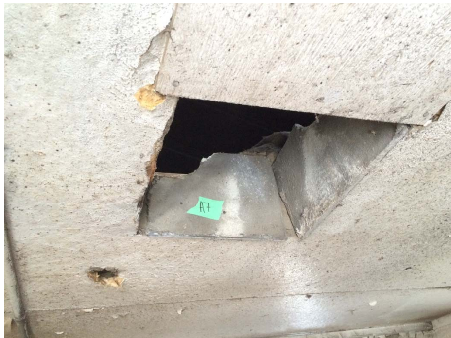
Photograph 2: Sample A7 – Old Generator Shed – Asbestos-containing off-white insulation in the chimney located nearest the entry door.
