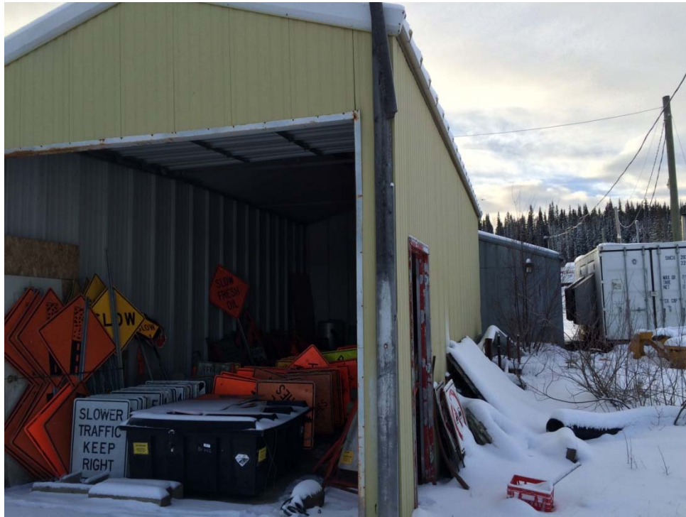
Photograph 9: Samples P14, P15 and P16 – Sign Shed – Lead containing red (P14), yellow (P15), and white (P16) paints on the exterior.
