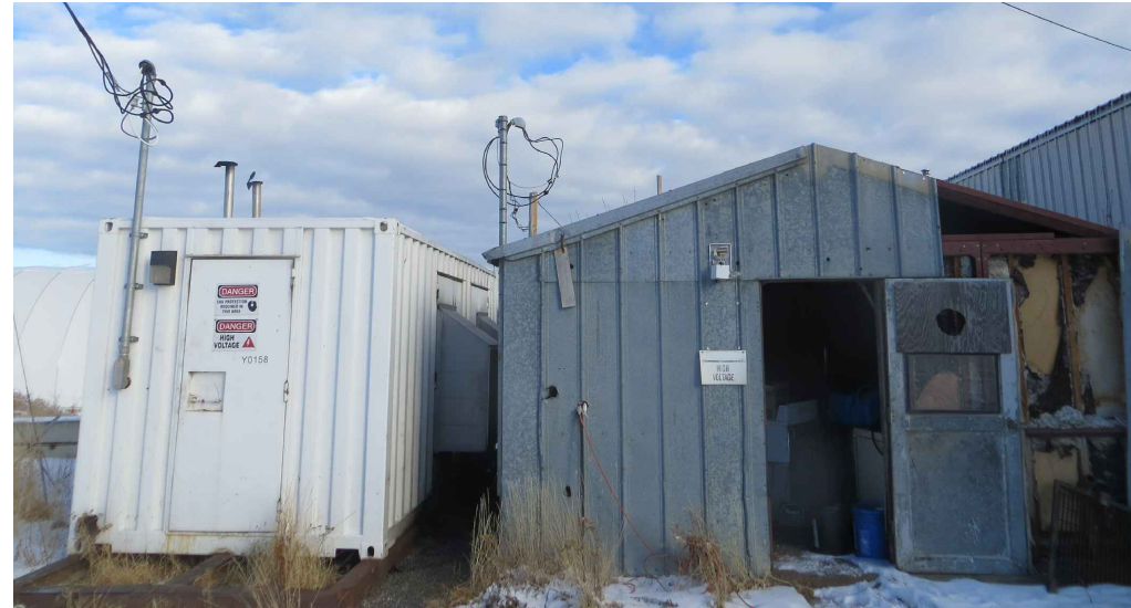
EXISTING STORAGE BUILDING IN POOR CONDITION TO BE DEMOLISHED AND EXISTING GENERATOR IN ENCLOSURE TO BE RELOCATED
