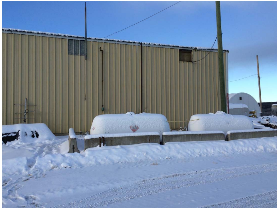
Photograph 17: Propane tanks located on the exterior of the Maintenance Garage.
