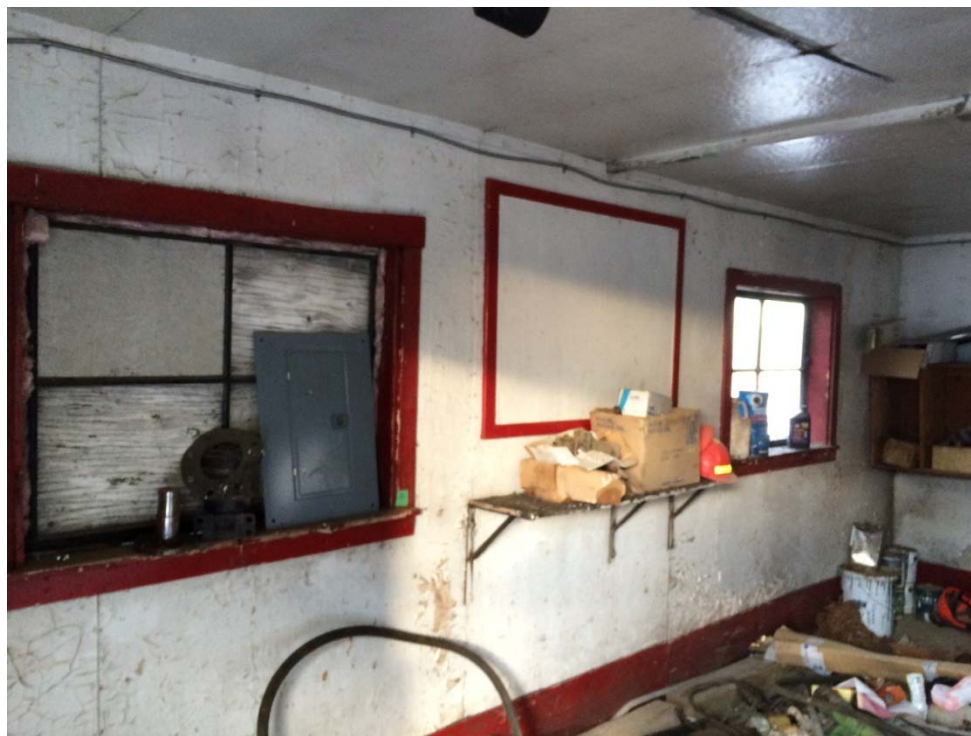
Photograph 10: Samples P6, P7, P8, P9 and P12 – Old Generator Shed – Lead-Containing white (P6 and P8) and red (P9) paint on the metal framing beams, and black (P12) and red (P7) paint on the window frames and wooden trim.
