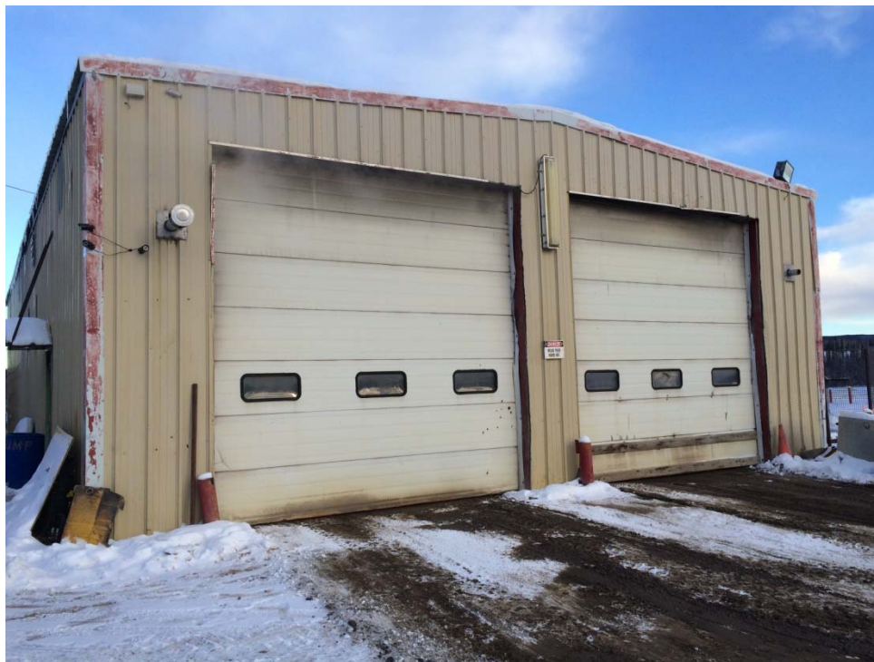
Photograph 14: Suspect PCB-containing HID fixture on the exterior wall of the Maintenance Garage.
