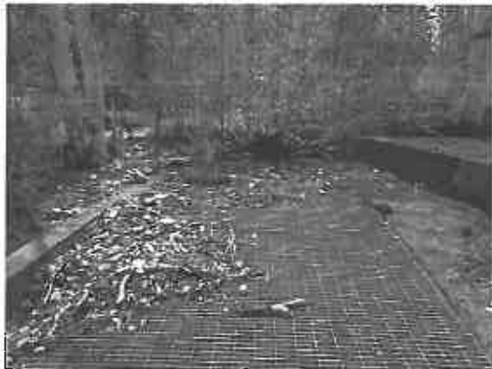
Picture No. 3: Typical Debris Atop Fishway at Time of Visit
