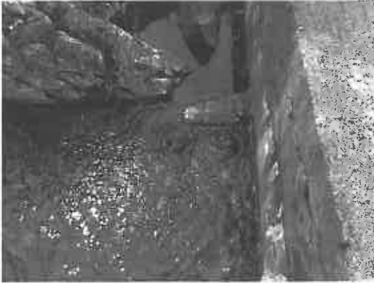
Picture No. 7: Location of Diversion Dam Leaks
