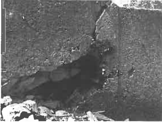
Picture No. 1: Location of Required Fishway Repair near Downstream Exit
