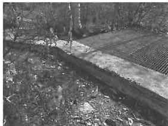
Picture No. 12: Condition of Wall Slated for Recapping
