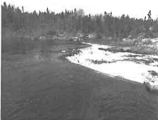
Picture No. 17: Location of Diversion Wall Repair Adjacent to Fishway Entrance at Lower Right
