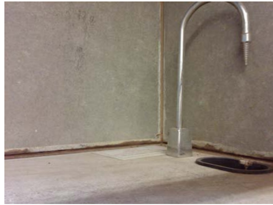
Photo 1.16 – Header House fumehood contains asbestos.
