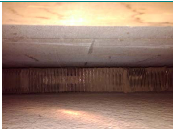
Photo 1.11 - Header House cement board lining inside heater-contains asbestos
