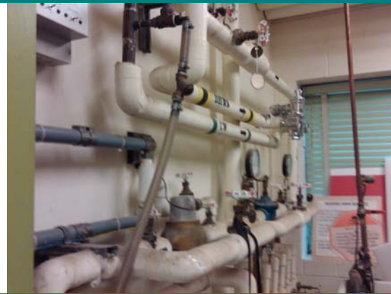
Photo 1.18 – Header House heating pipes H2O sampled, no asbestos detected.
