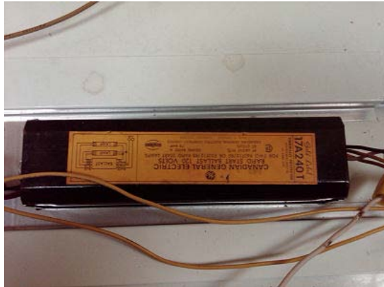
Photo 1.7 Annex Ballast-suspected to contain PCB's
