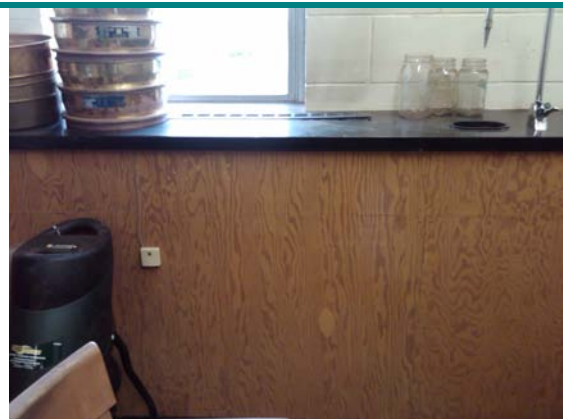
Photo 1.12 – Inside lining contains asbestos.
