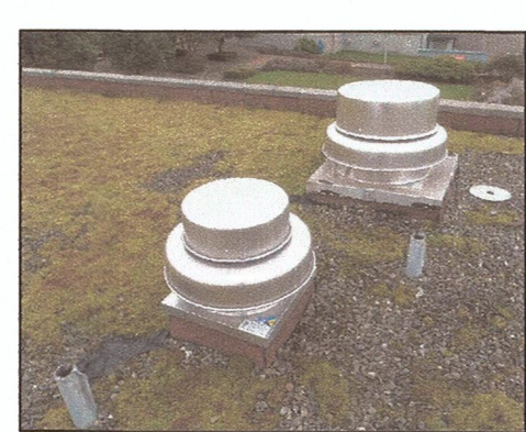
PHOTO 1 TYPICAL MECHANICAL DOWNBLAST EXHAUST FANS AND PLUMBING VENT STACKS
