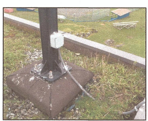
PHOTO 5 CCTV CAMERA CURB
