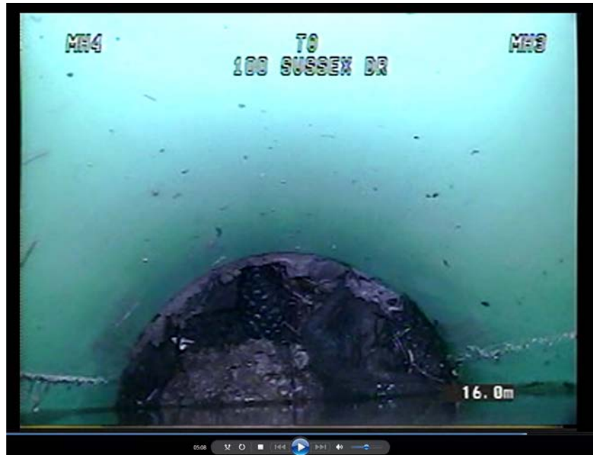
Blocked Pipe Looking North
