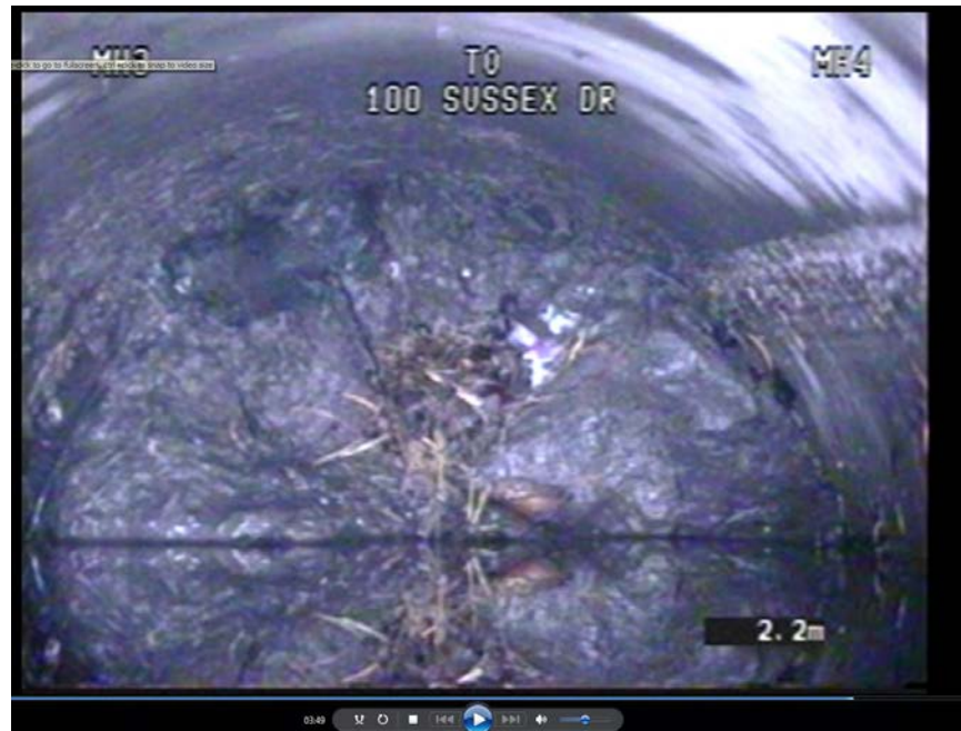
Blocked Pipe Looking South Toward Sussex - Zoomed
