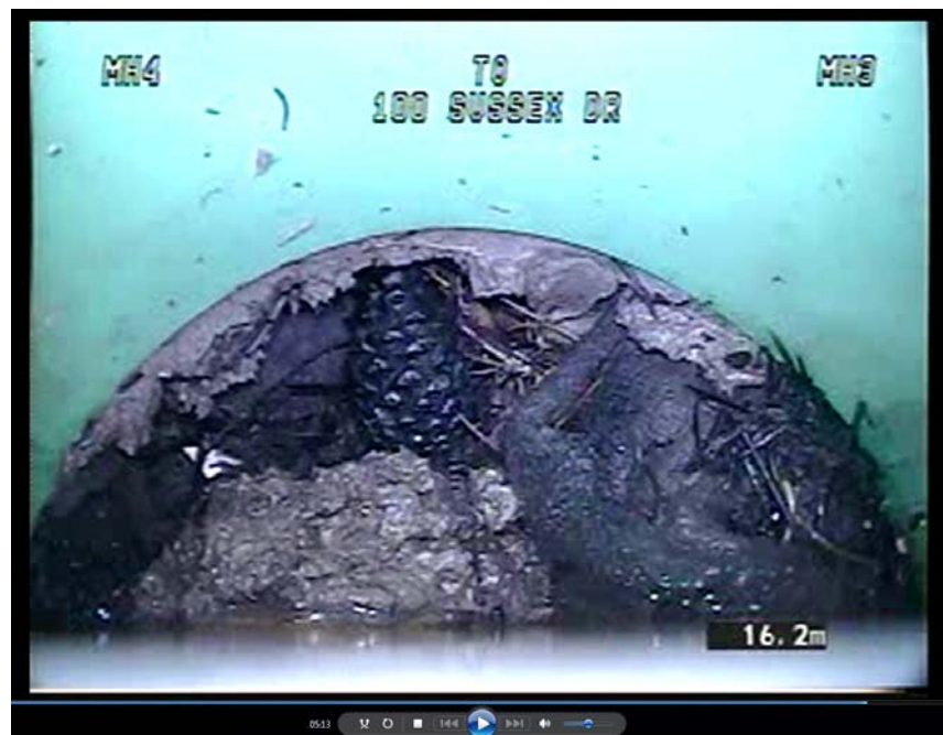
Blocked Pipe Looking North – Zoom
