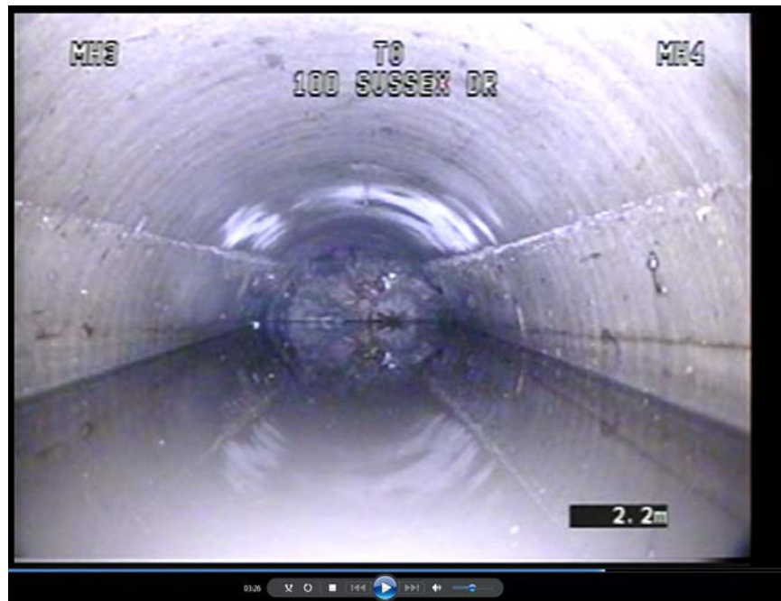
Blocked Pipe Looking South Toward Sussex
