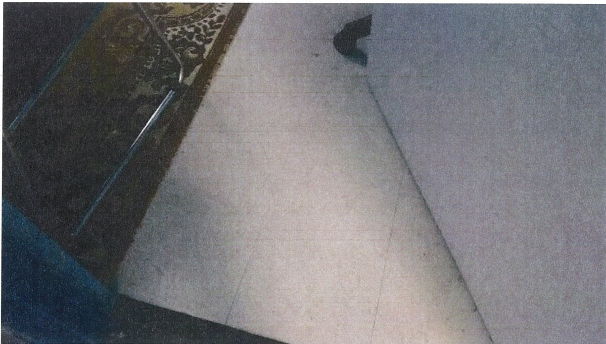
Sample B5 – floor tile same as 238 that was previously sampled – non ACM.
