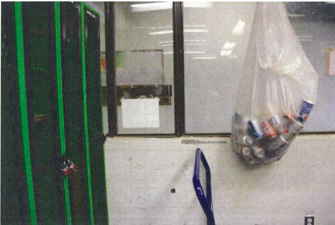
Damaged drywall on north windows.
