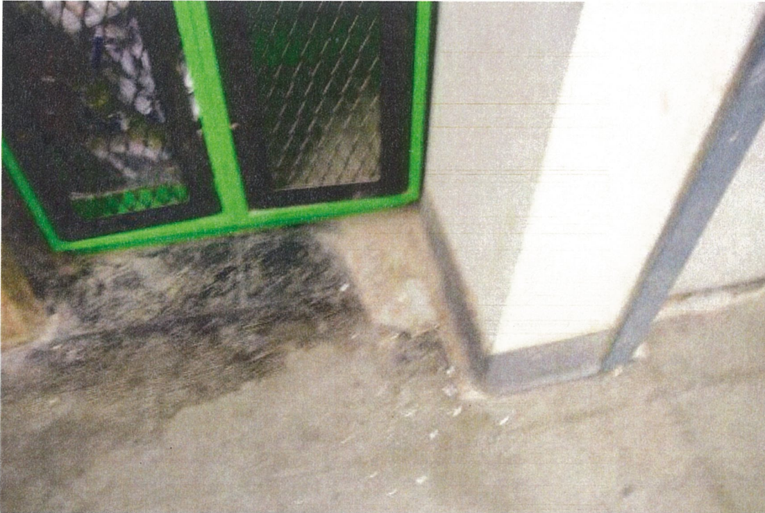
Traces of grey floor tile and exposed mastic throughout perimeter of Hobby Shop (Room 248).
