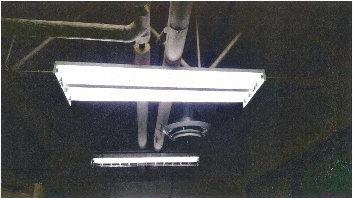
T8 light tubes throughout.
