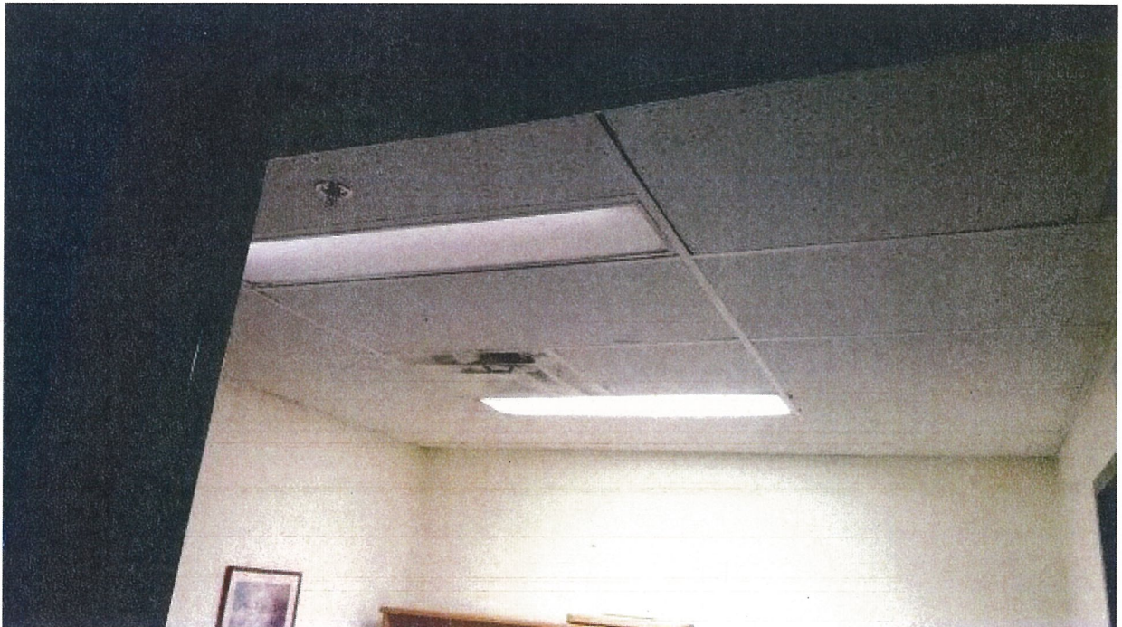
Ceiling tiles (Room 249).
