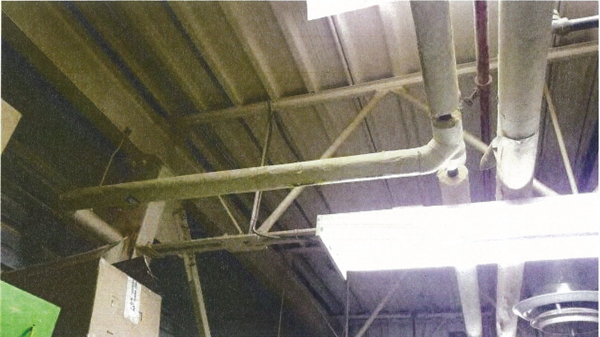
Fibreglass pipe lagging.
