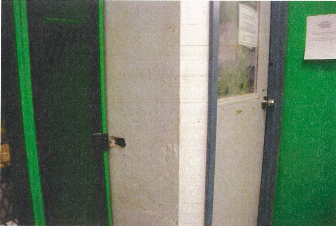
Damaged drywall on office entrance.
