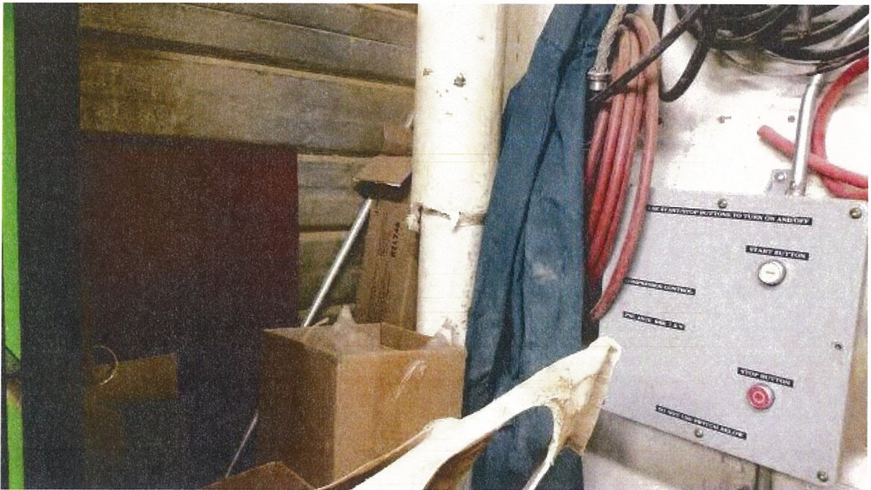
Damaged pipe insulation in Room 247 - Sample B15A.
