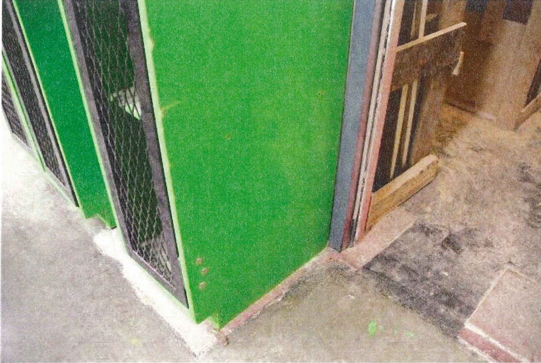
Room 247C and under lockers – traces of floor tile same as the rest of the floor (grey 12" VFT Samples B5 and B6) – tiles are just painted red.
