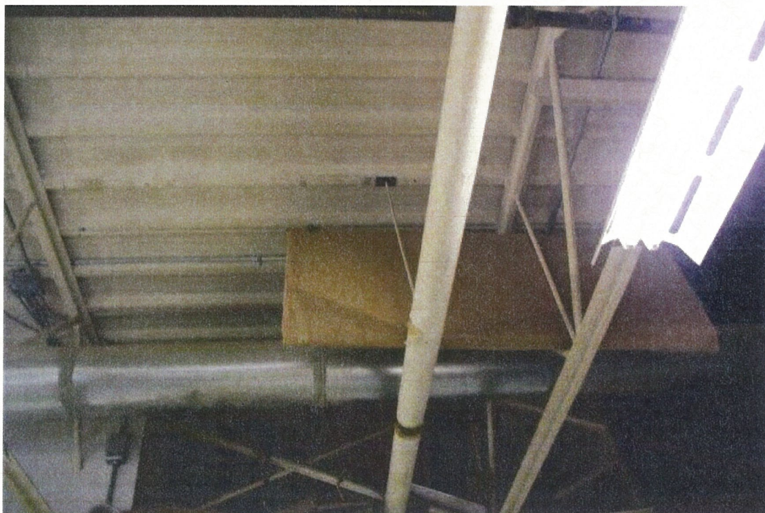
Pipe lagging – fibreglass.
