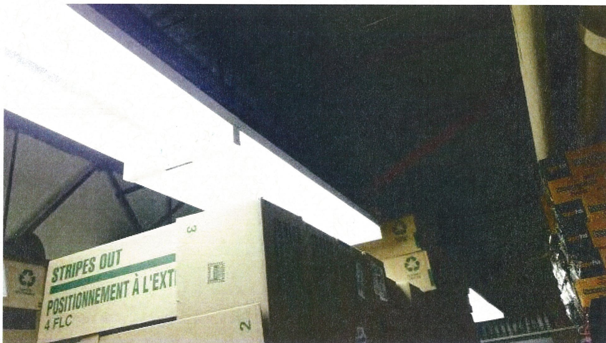
T8 lights throughout.
