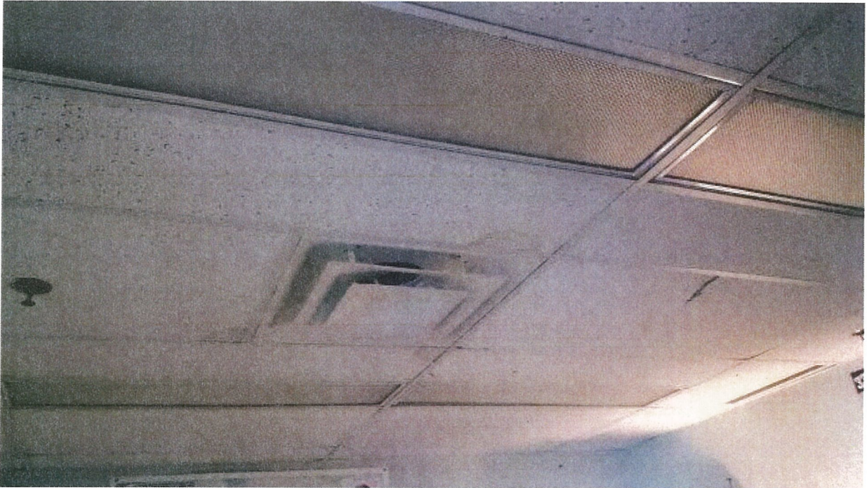
Minor water staining on ceiling tiles (in Room 238).
