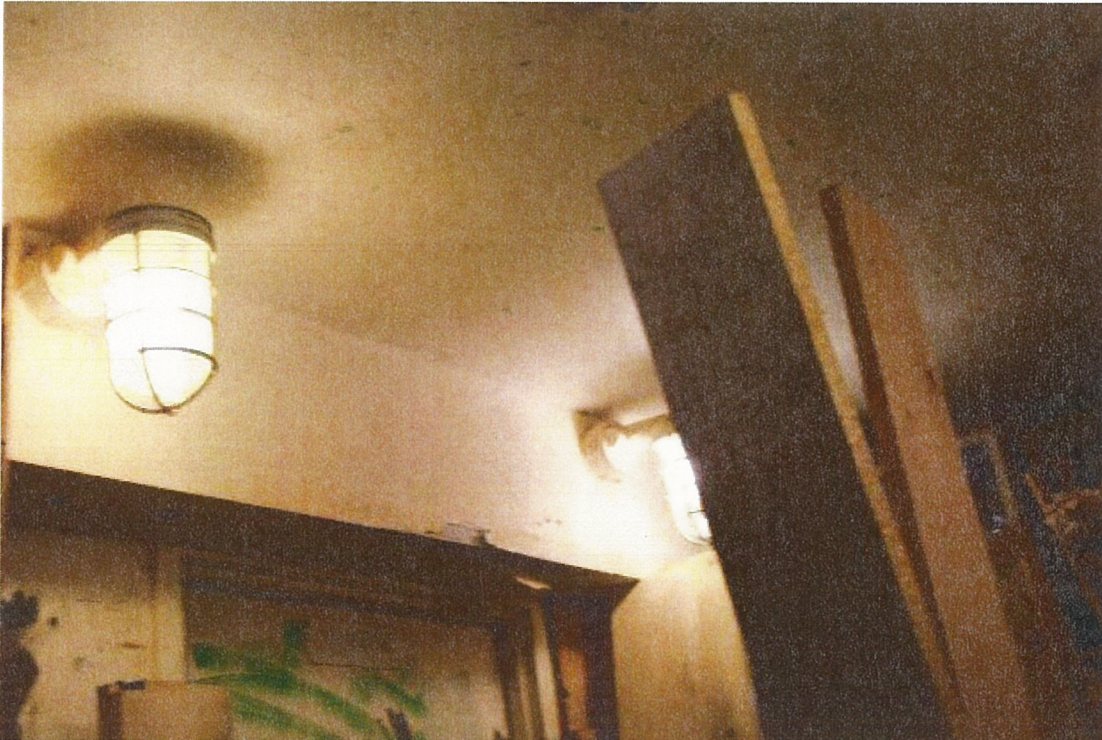
Room 247C – damaged drywall mud – north wall.
