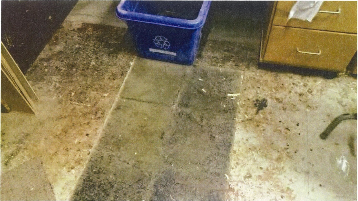
Some areas of missing floor tiles in 247A – not damaged – Known ACM.
