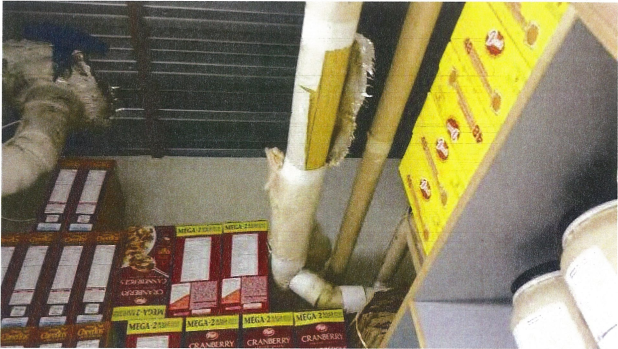
Fibreglass pipe insulation.
