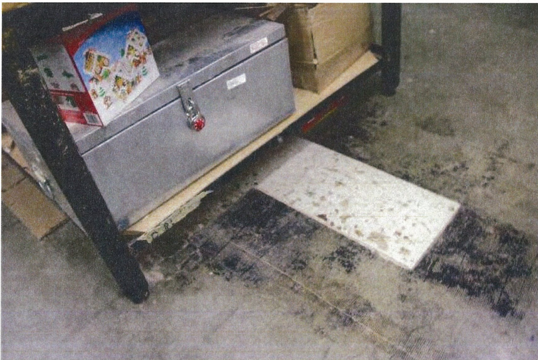
Traces of grey floor tile and exposed mastic throughout perimeter of Hobby Shop and under tables.
