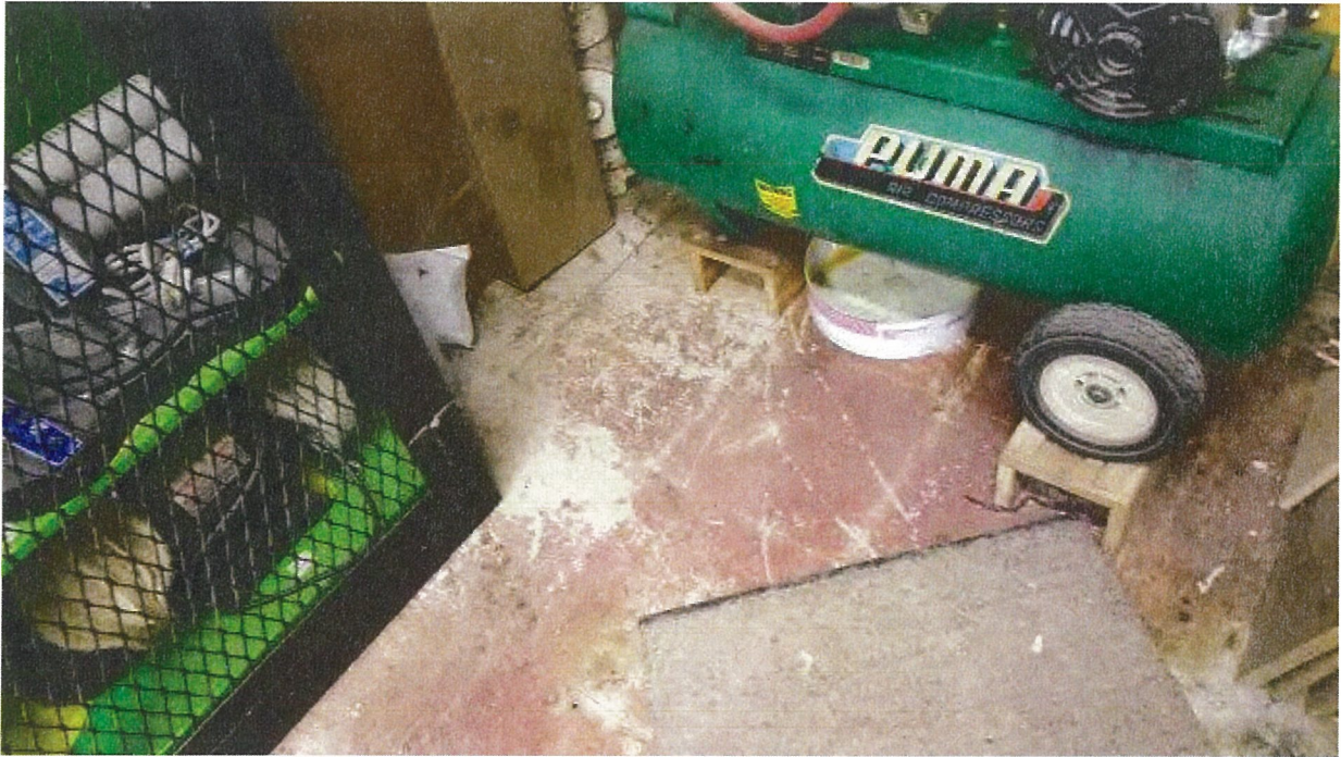
Known asbestos floor tiles in 247 – with red paint on top – minor damage.
