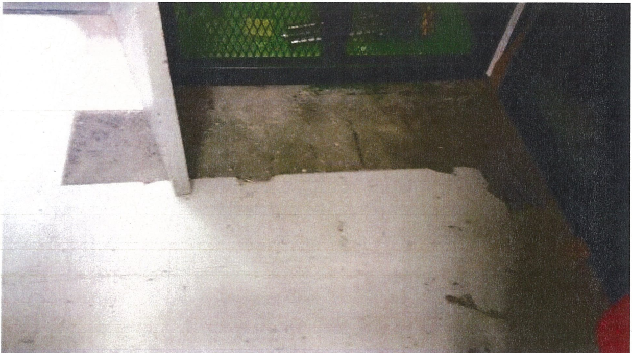
Some missing, damaged asbestos floor tiles in 247A.
