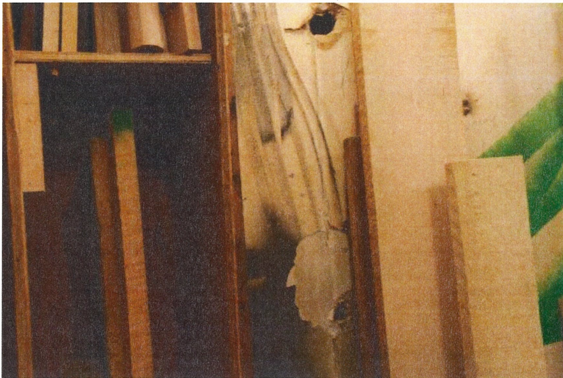
Room 247C – damaged drywall mud – north wall.
