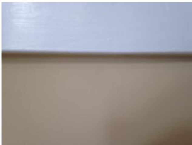
Figure 1: White paint on trim in house #10 (NL1724-L16)
