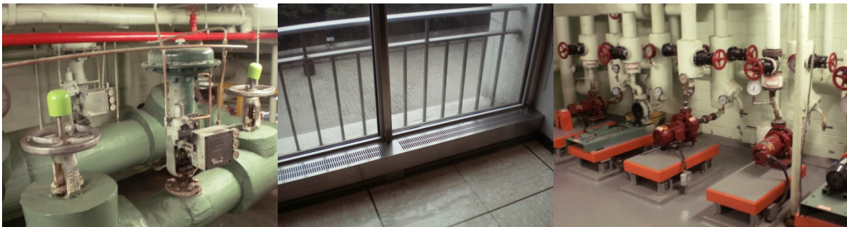
From Left: Pressure reducing valves for central steam supply, perimeter radiant heater on the ground floor, perimeter heating loop pumps
