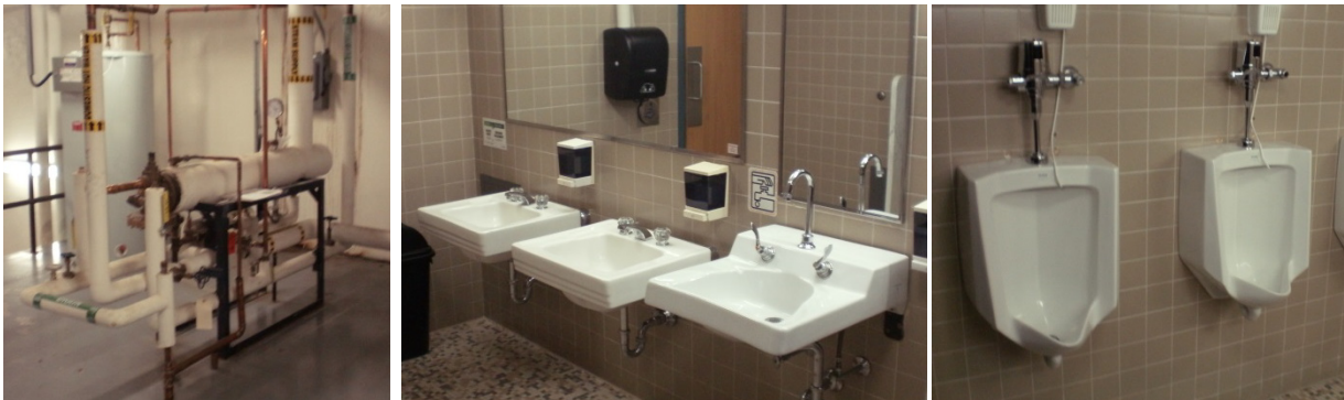
From Left: Domestic hot water heat exchanger, typical sink arrangement, motion sensor controlled urinals
