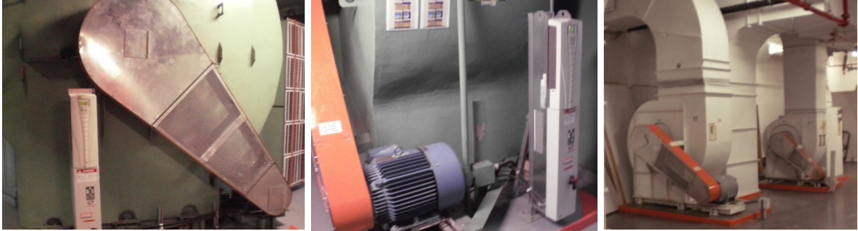
From Left: Supply fan S6-A, VFD on ventilation fan, smoke exhaust fans
