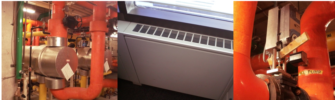
From Left: Steam heat exchangers, perimeter radiant heating unit, AHU heating coil bypass valve
