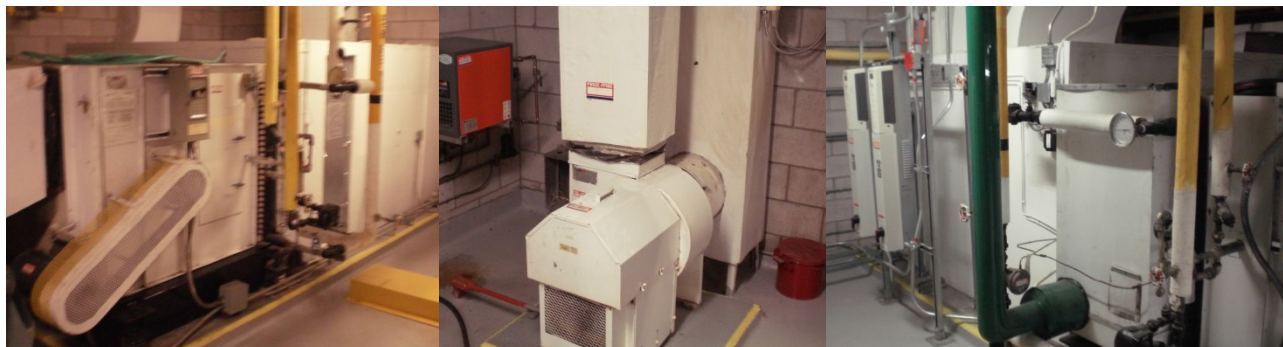
From Left: CAV air handling unit, exhaust fan, VAV air handling unit
