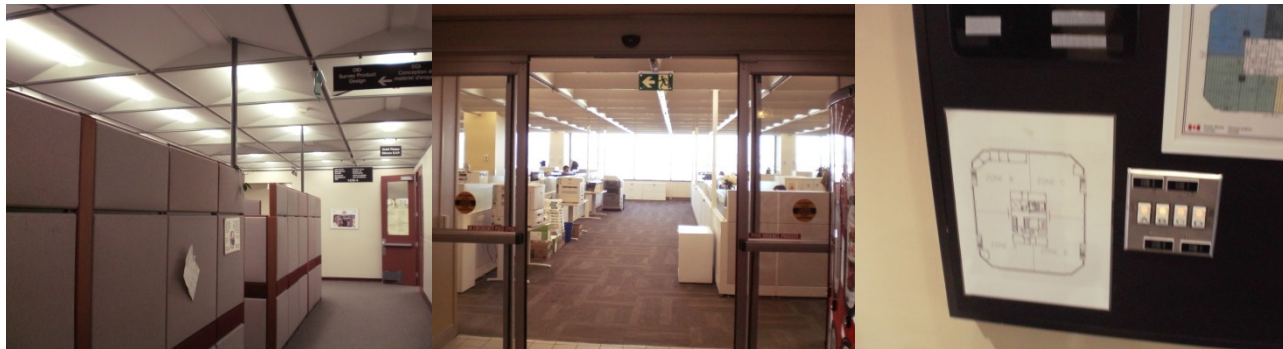
From Left: Interior office area lighting, perimeter office area lighting, lighting controls in the lobby
