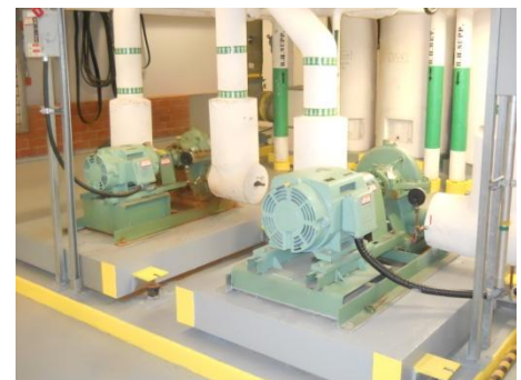
Primary and Backup Induction Unit Pumps
