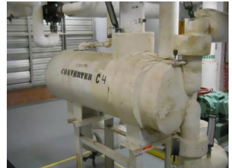
Typical AHU Converter
