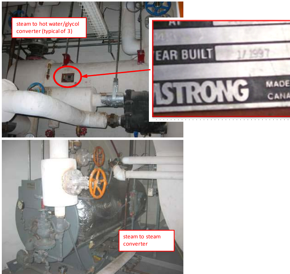
Figure 3.4: East Memorial Steam Converters and Steam to Steam Exchanger
