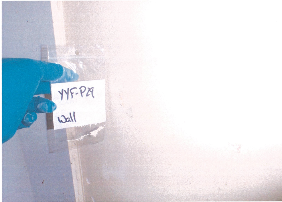
Photograph 79: Lead-based beige paint on walls of Room 138 ( Sample P29 ).
