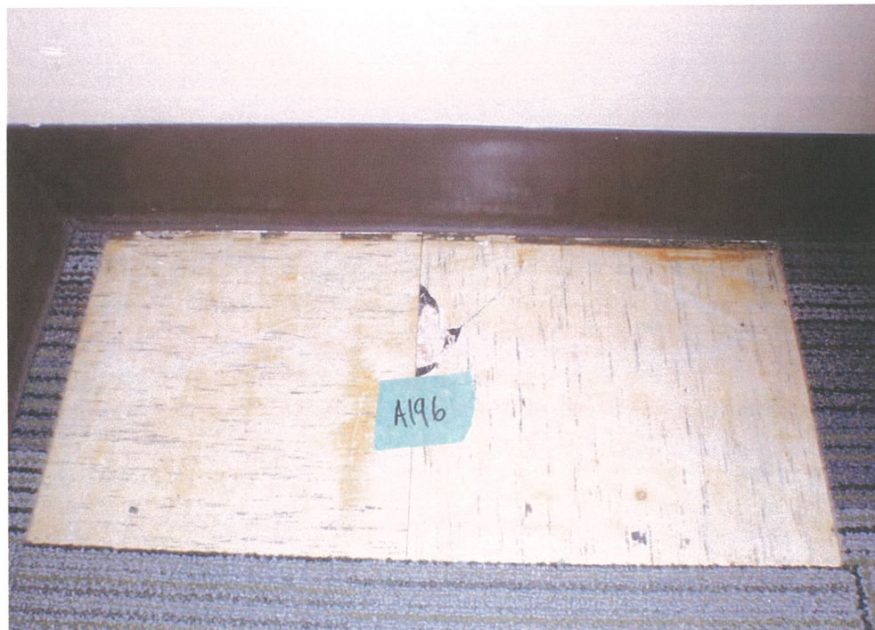
Photograph 56: Asbestos-containing white vinyl floor tile in Room 112 (Sample A196).
