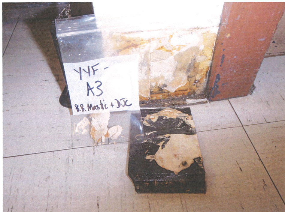
Photograph 28: Asbestos-containing drywall joint compound in Room 125 (Sample A3).
