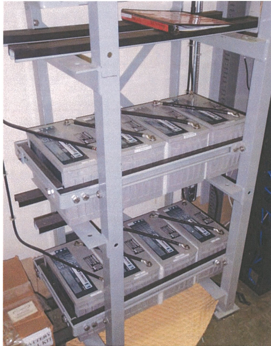
Photograph 23: Room 127 lead-containing batteries.
