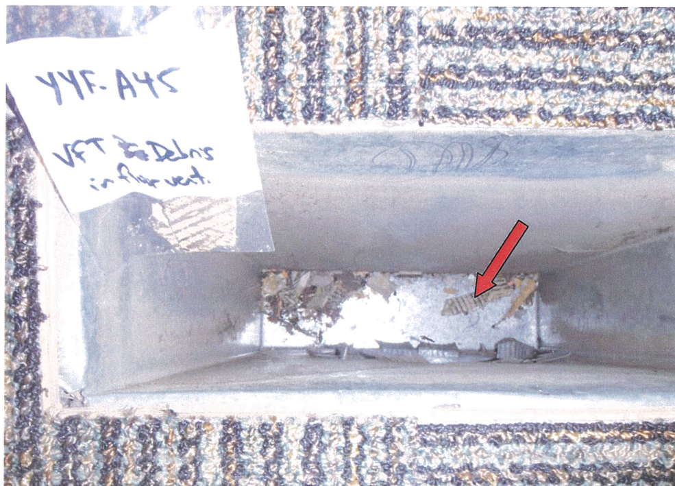
Photograph 42: Asbestos-containing grey vinyl floor tile debris located in the floor vent in Room 120 (Sample A45).
