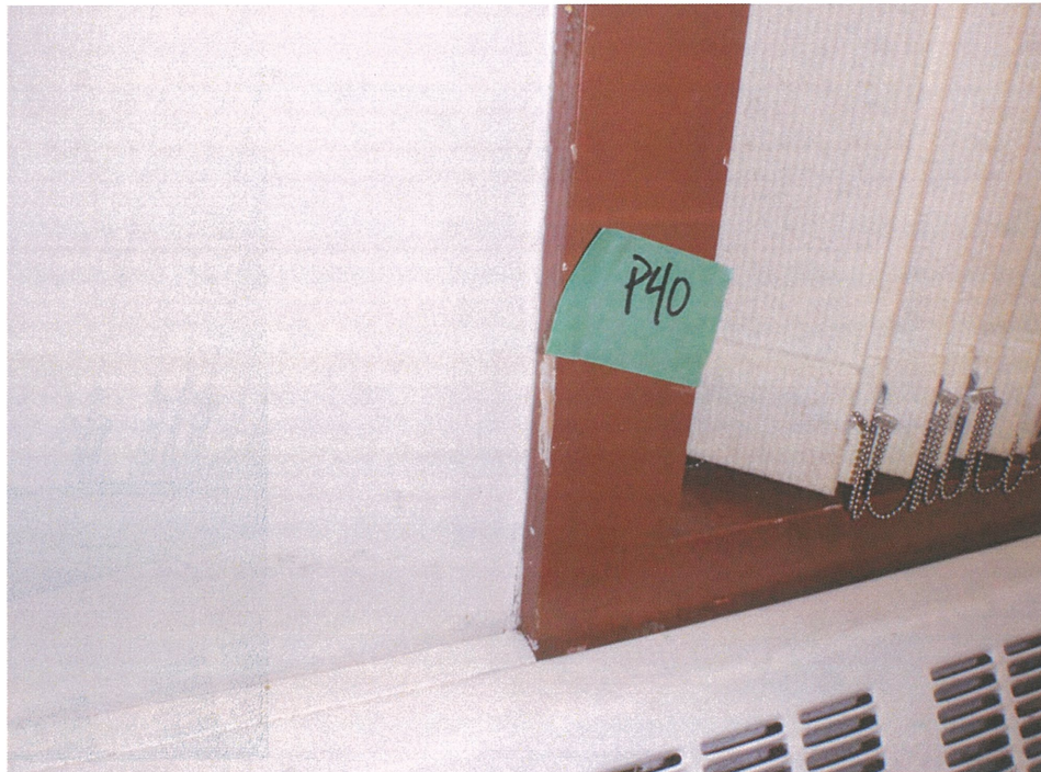
Photograph 83: Lead-based red paint on window trim along the west wall of Room 106B (Sample P40).
