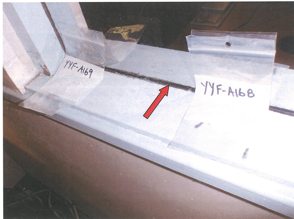
Photograph 52: Asbestos-containing grey window putty in Room 117 (Sample A168).
