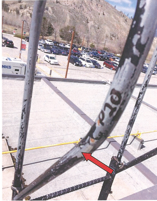
Photograph 71: Lead-based black paint on ladder to raised portion of roof (Sample P20).
