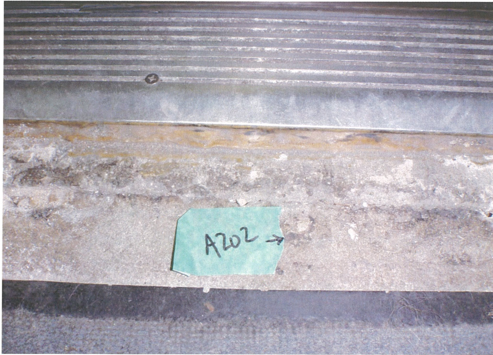
Photograph 57: Asbestos-containing tar on floor adjacent door step in Room 110 (Sample A202).
