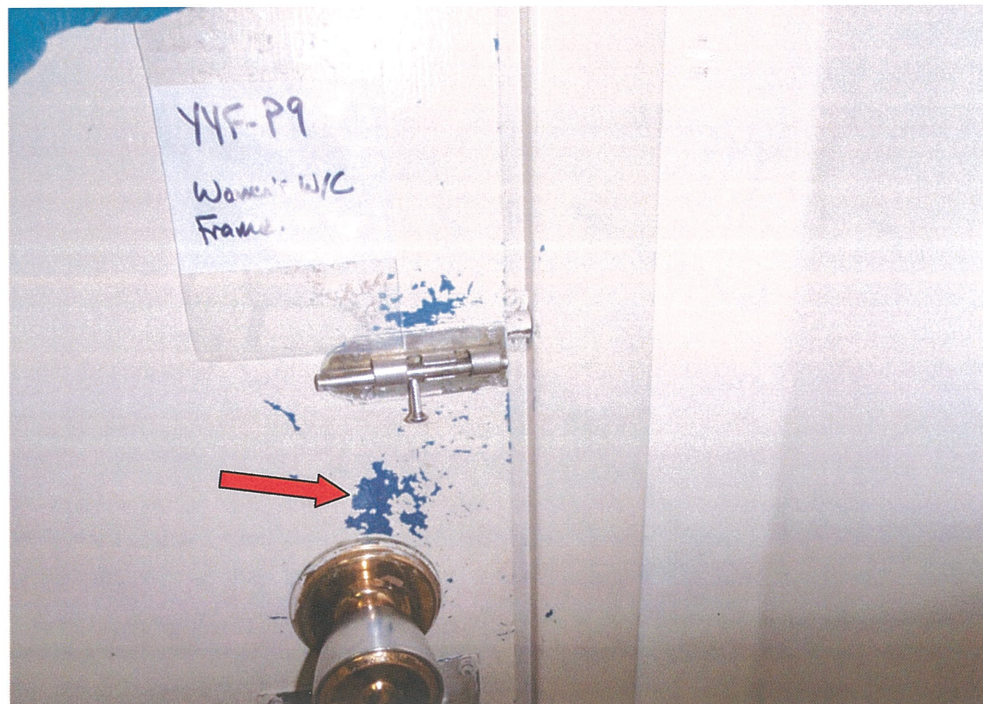
Photograph 64: Lead-based light brown / blue paint on door to Room 130 (Sample P9).
