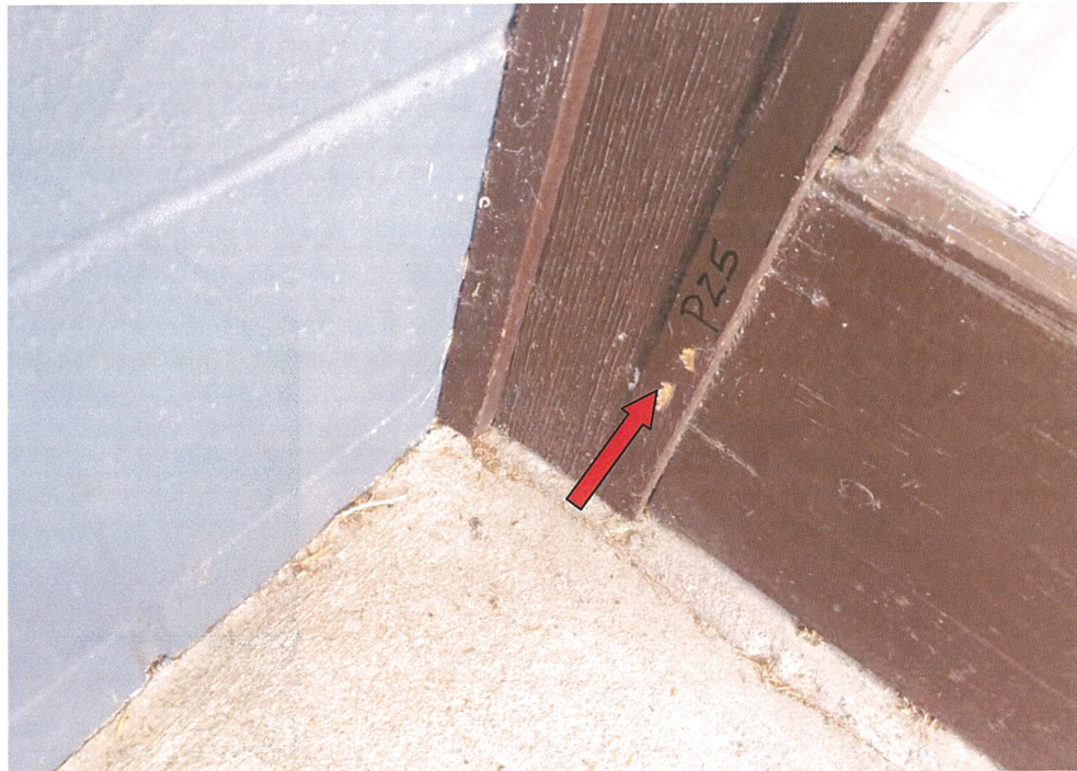
Photograph 75: Lead-based dark brown paint on exterior door frame to Room 125 ( Sample P25 ).
