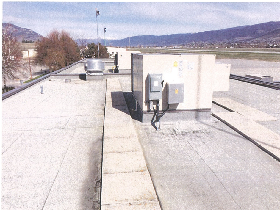
Photograph 26: Typical rooftop air conditioning unit.
