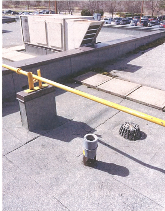
Photograph 27: Typical potential lead-containing roof vent pipe.
