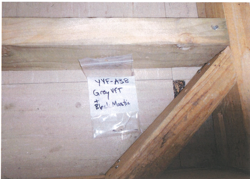
Photograph 38: Asbestos-containing grey vinyl floor tile ( Sample A38 ).
