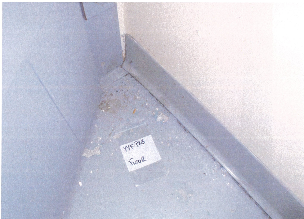
Photograph 78: Lead-based grey floor paint on concrete in Room 138 (Sample P28).
