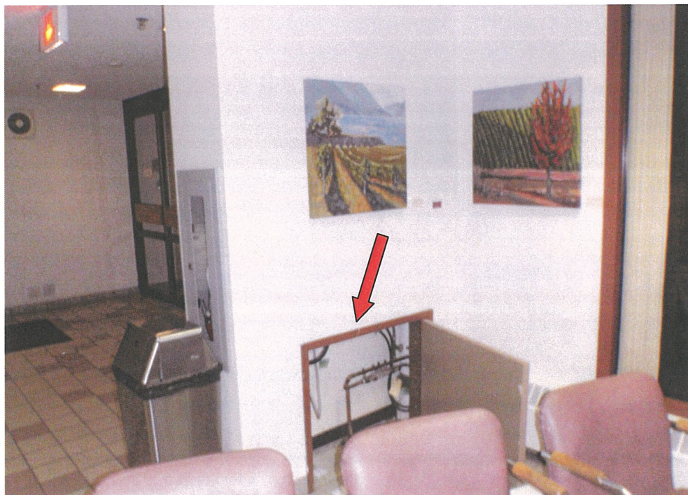
Photograph 12: Wall compartment in Room 106B (south wall), north of entrance – Facing southwest.
