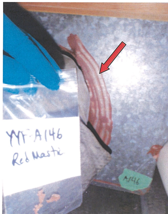
Photograph 50: Asbestos-containing red mastic on HVAC ducting in crawlspace beneath Room 136 (Sample A146).
