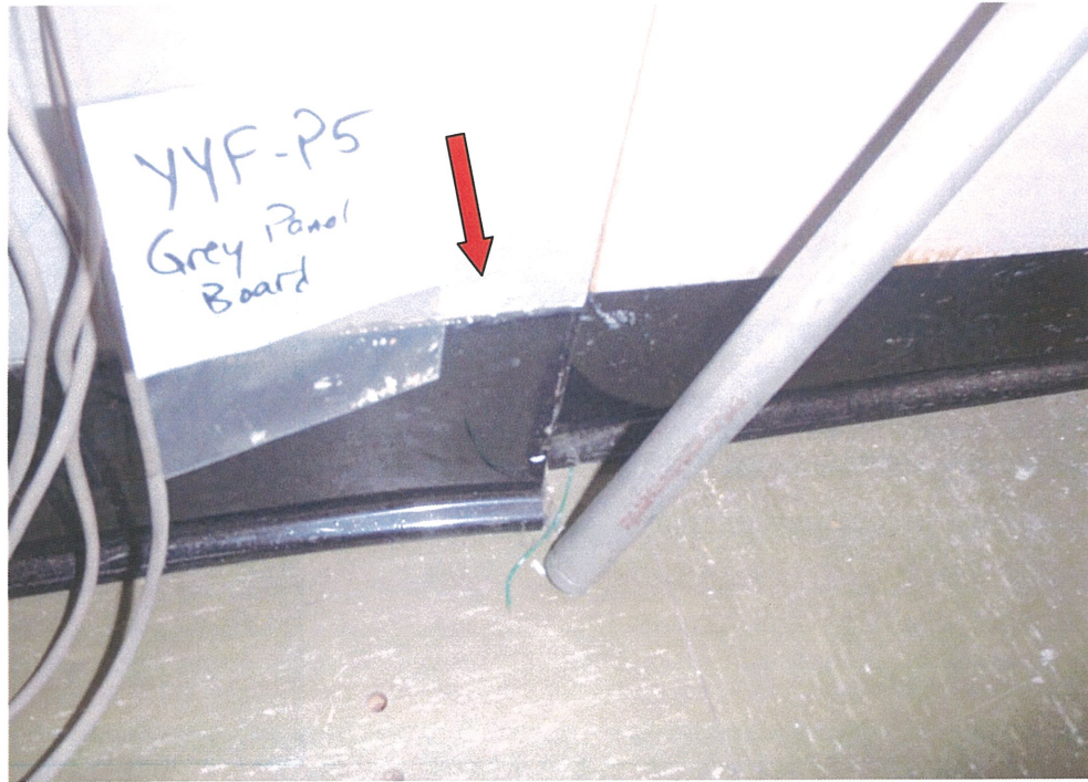
Photograph 63: Lead-based grey paint on a wall panel in Room 127 (Sample P5).
