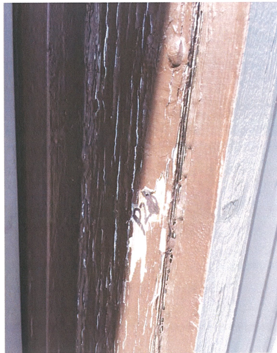
Photograph 72: Lead-based dark brown paint on window trim on east side of raised portion of roof (Sample P21).
