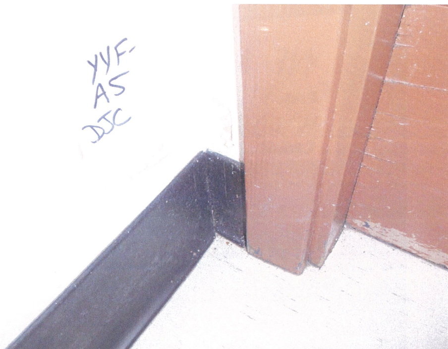
Photograph 30: Asbestos-containing drywall joint compound in Room 125 (Sample A5).
