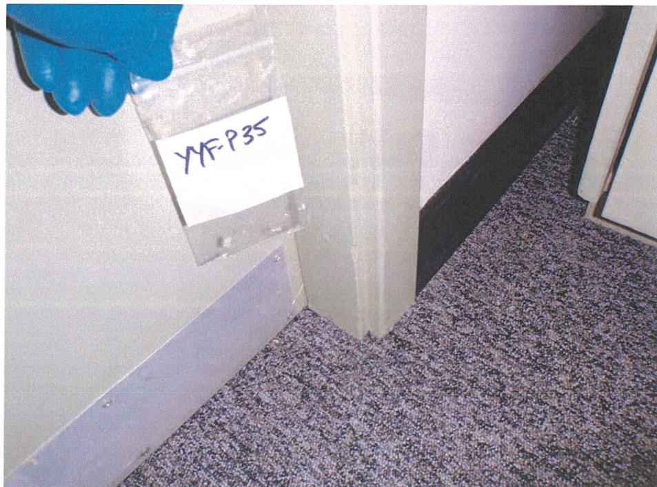
Photograph 82: Lead-based green paint on door frame of Room 135 ( Sample P35 ).
