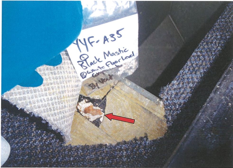
Photograph 37: Asbestos-containing grey vinyl floor tile ( Sample A34 ) and associated black mastic ( Sample A35 ) over white floor leveling compound ( Sample A35 – Layer 2 ) in Room 123.
