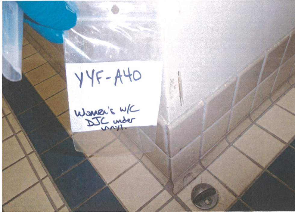
Photograph 39: Asbestos-containing drywall joint compound in Room 130 ( Sample A40 ).
