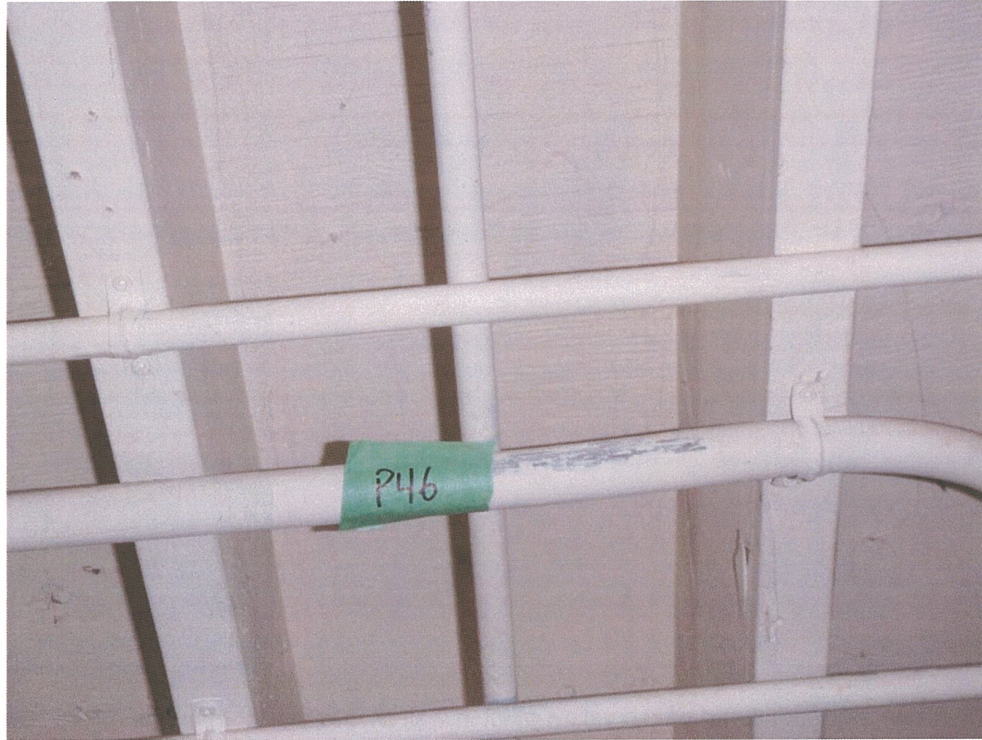
Photograph 87: Lead-based beige paint on steel pipe near ceiling of Room 107 ( Sample P46 ).
