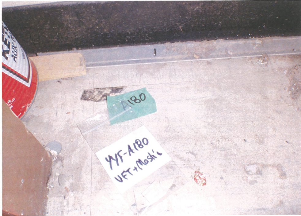
Photograph 55: Asbestos-containing grey vinyl floor tile located inside wall compartment in Room 106B (Sample A180).
