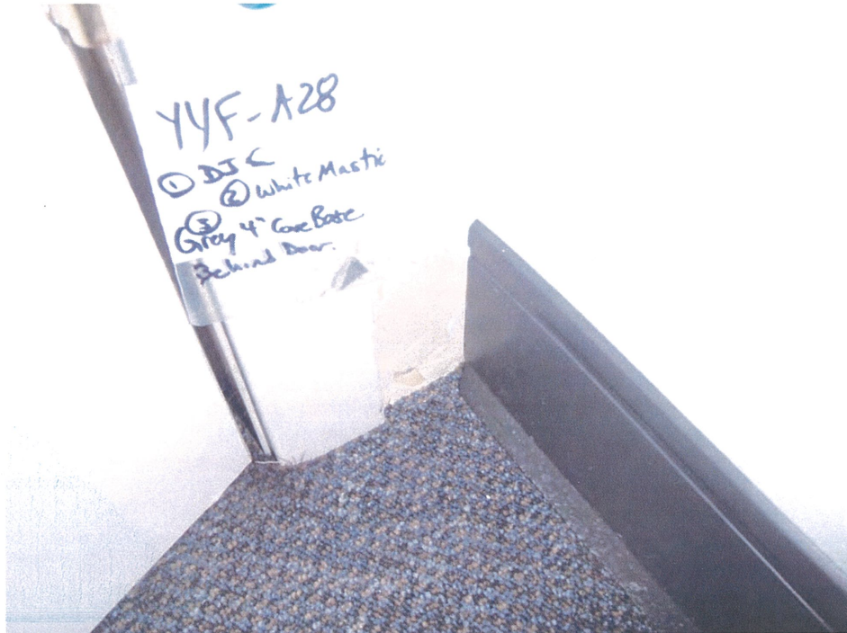
Photograph 35: Asbestos-containing drywall joint compound in Room 124 (Sample A28).
