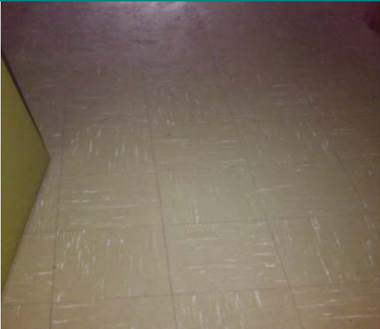
Photo 1.21 - Typical Floor tiles-contains asbestos.
