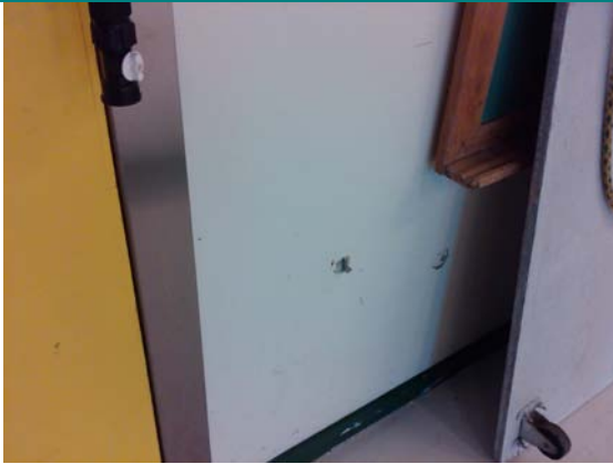
Photo 1.13 Header House drywall joint compound contains asbestos
