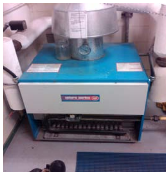
Photo 1.17 - Header House building heater
